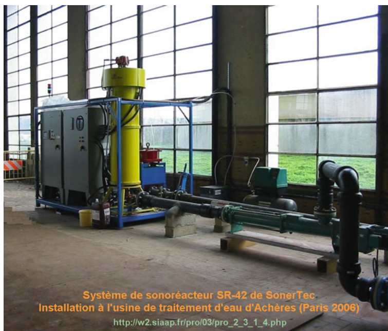
Fig. 7.9 The “DigestSonic” SR-42 system installed in a sludge treatment plant in France
