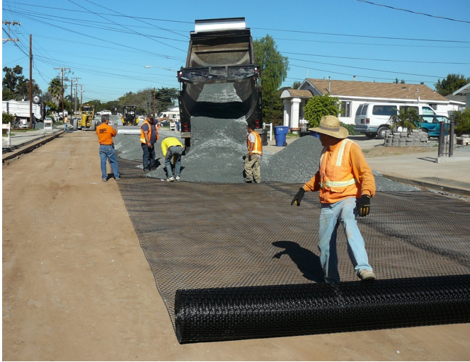
Figure 14.25 Triaxial geogrid beneath base coarse for a paved roadway. Courtesy of Tensar International Corp.
