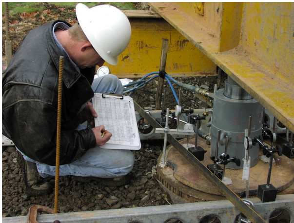
Figure 6.22 Field load test of a Geopier® system. Copyright by Geopier Foundation Company, Inc. Reprinted with permission.
