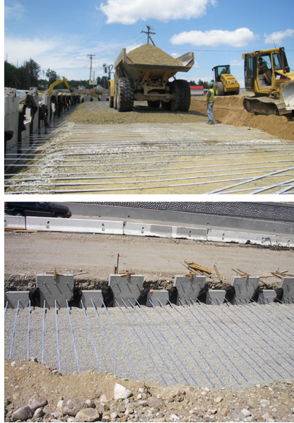
Figure 14.2 Construction of a metallic strip reinforced wall. Courtesy of The Reinforced Earth Company.
