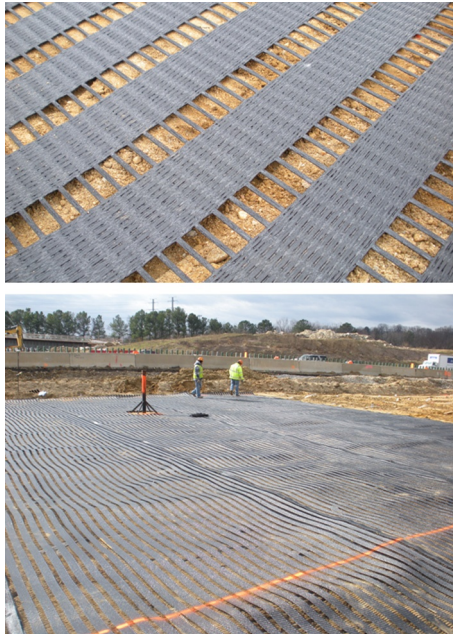
Figure 14.20 Application of high strength polyester/polyethylene geogrid for a new highway interchange. Courtesy of Maccaferri-USA.
