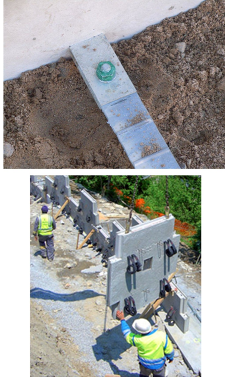
Figure 14.11 Typical wall connections for precast facing panels. Courtesy of The Reinforced Earth Company.
