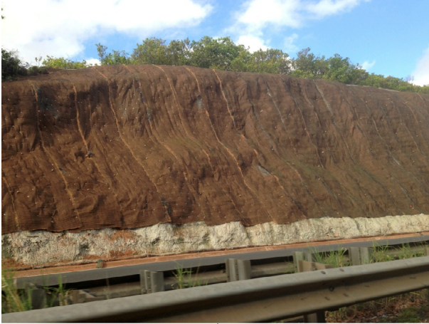
Figure 14.27 Pinned reinforcement mat for stabilization (erosion control and sloughing) of shallow, surface soils of steep roadcut, Kailua, HI.
