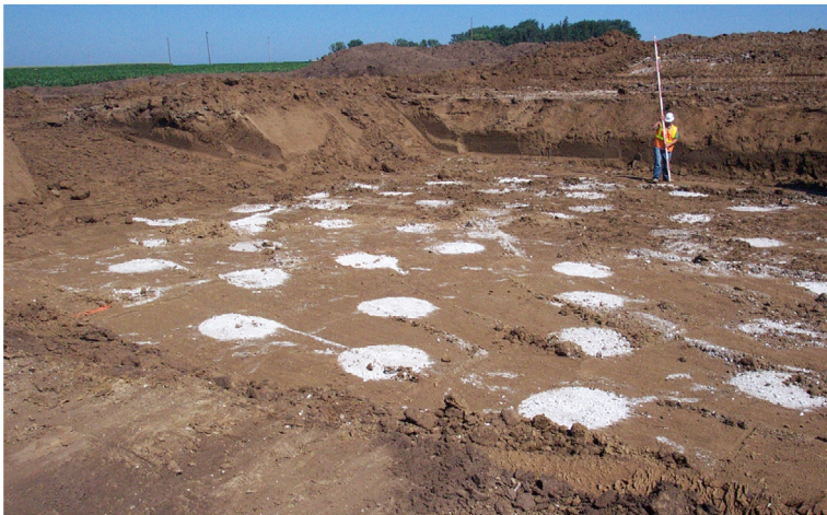
Figure 6.11 Geopier ® reinforced site. Copyright by Geopier Foundation Company, Inc. Reprinted with permission
