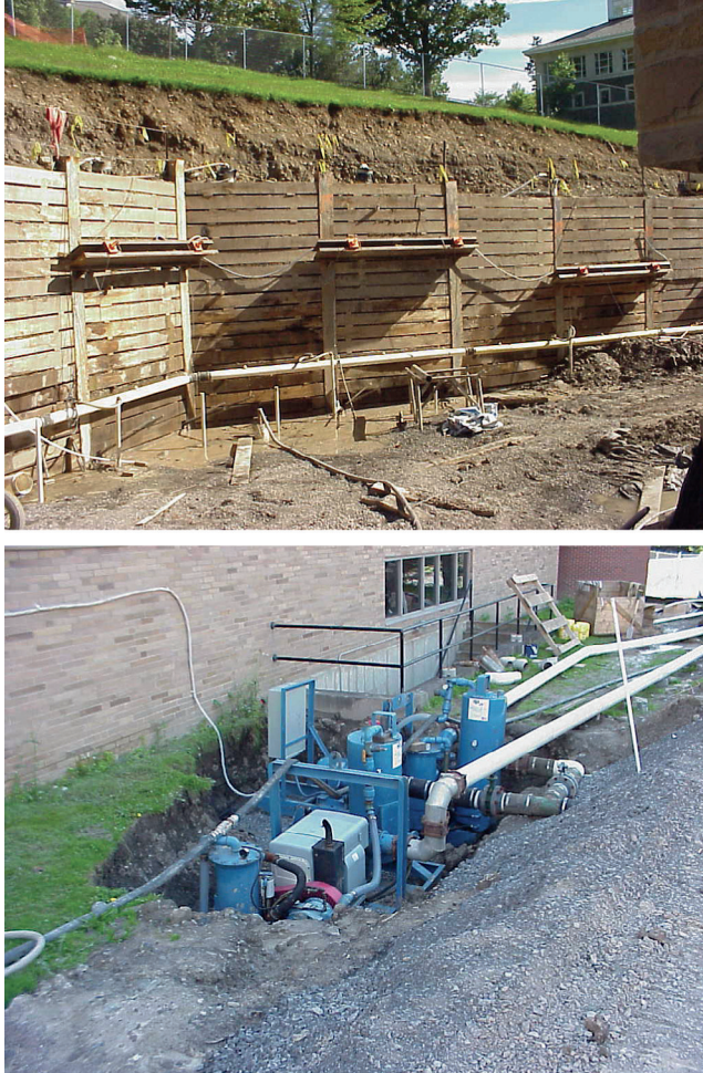
Figure 7.5 Wellpoint application and pump for a building excavation, Colgate University, NY. Courtesy of Moretrench.
