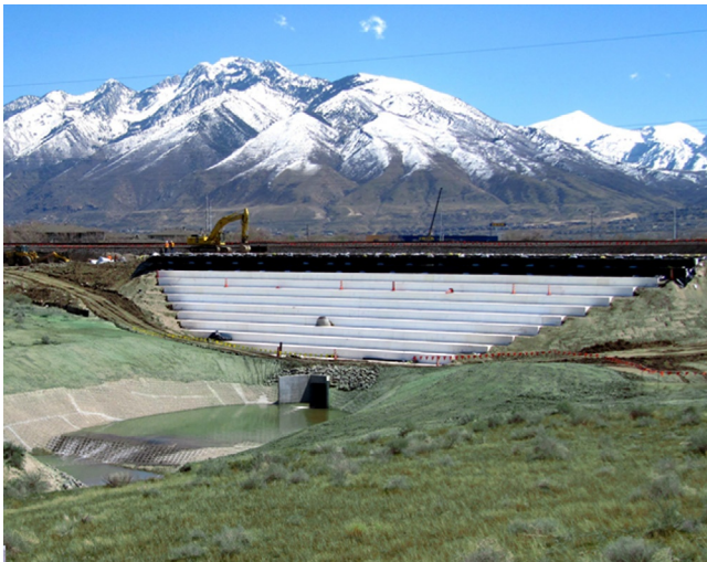
Figure 17.5 Commuter rail embankment over a box culvert, Draper, UT. Courtesy of ACH Foam Technologies.
