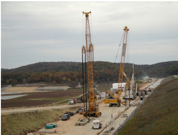
Figure 7.2 Installation of a 60 m (200 ft) deep slurry cutoff wall at Clearwater Dam, Piedmont, MO. Courtesy of Layne Christensen.
