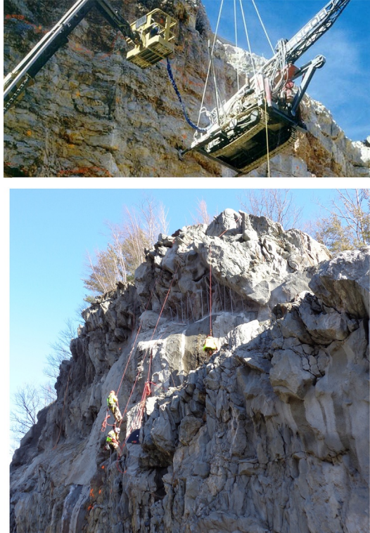
Figure 15.8 Rockfall mitigation with nails/rock bolts. Top: Courtesy of Layne Christensen; Bottom: Courtesy of GeoStabilization International.
