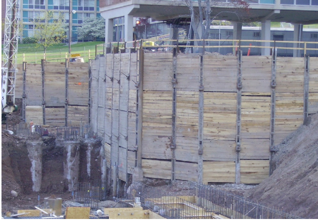
Figure 15.1 Ground anchor supported soldier beam and lagging excavation wall. Courtesy of Hayward Baker.
