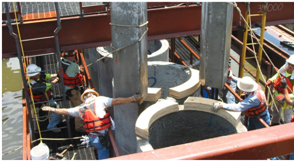
Figure 12.18 Jet grouted assisted pile installation and closure IHNC MRGO. Courtesy Layne Christensen.
