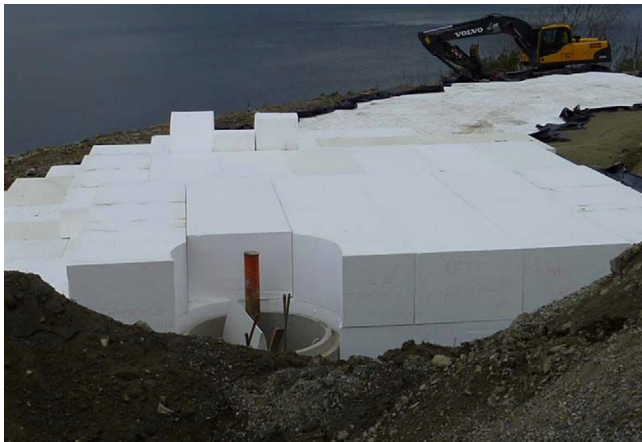
Figure 17.9 Cut and shaped geofoam fit around a drainage conduit. Courtesy of Atlas EPS.
