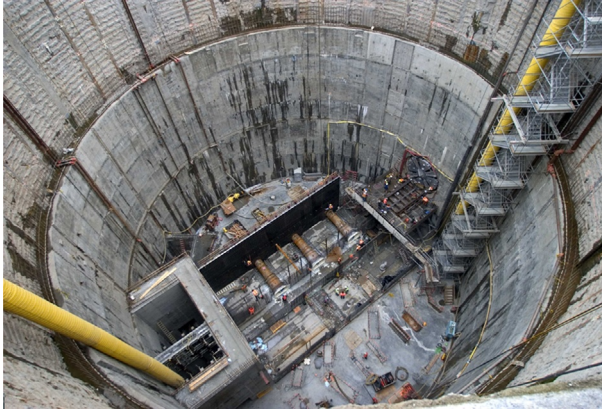
Figure 12.13 Deep shaft with jet grouted cut-off plug for sewer pump station in Portland, OR. Courtesy Layne Christensen.
