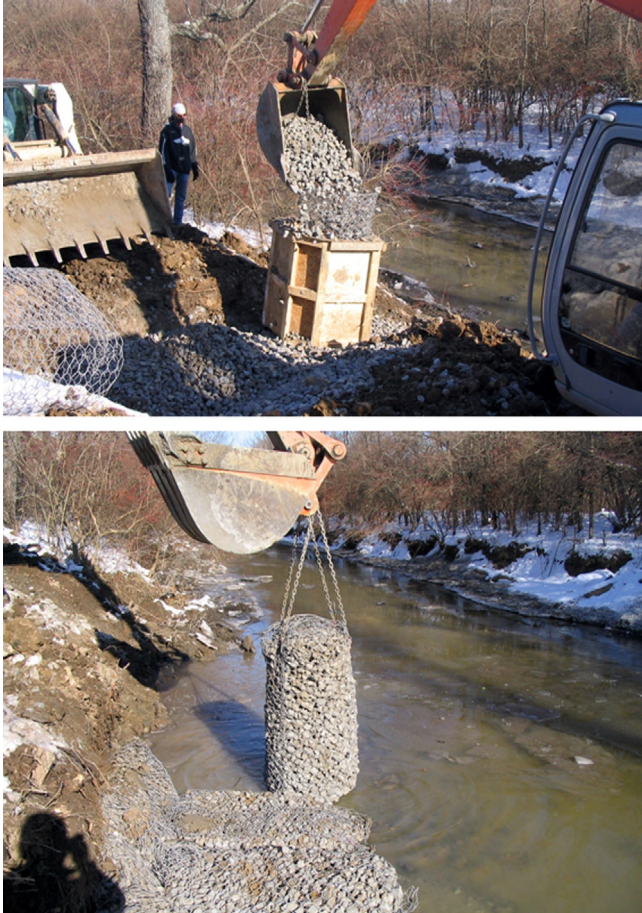
Figure 16.13 “Sack gabion” being filled and placed in water. Courtesy of Maccaferri, Inc.
