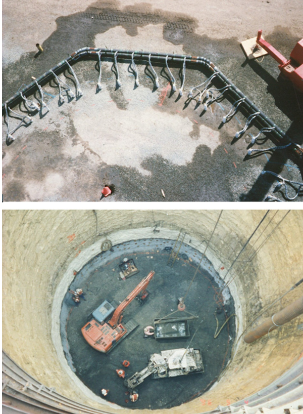
Figure 13.10 60 m (200 ft) deep, 18 m (60 ft) diameter shaft enabled by 90 m (300 ft) deep freezing, San Diego. Courtesy of Layne Christensen.
