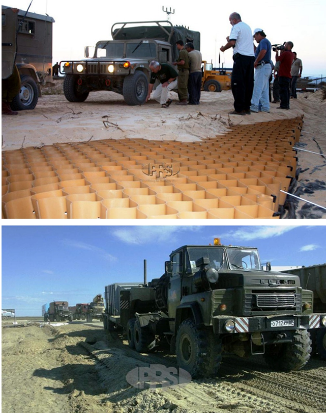
Figure 16.22 Geocells used in rapid road construction for military mobilization in desert environments. Courtesy of PRS Mediterranean Ltd.
