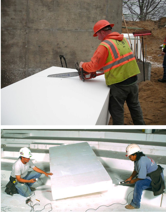
Figure 17.8 Cutting and shaping Geofoam blocks with a chainsaw (above) and hot wire saw (below). Courtesy of Atlas EPS.
