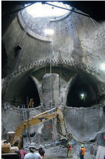
Figure 7.6 Application of deep wells to dewater for a deep shaft and tunnel excavation at Beacon Hill, WA. Courtesy of Moretrench.
