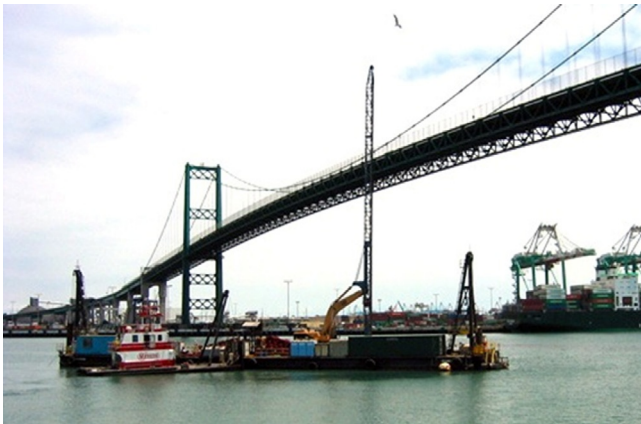
Figure 9.8 PVD install underwater (Port of Los Angeles). Courtesy of Hayward Baker/HB Wick Drains.
