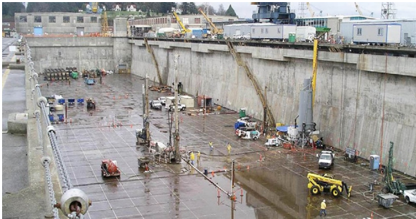
Figure 12.15 Re-leveling of the distressed floor slab of Puget Sound Naval Shipyard dry dock. Courtesy of Layne Christensen.
