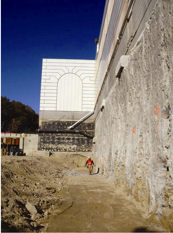
Figure 12.9 Continuous jet grout wall underpinning an existing building. Courtesy of Hayward Baker.
