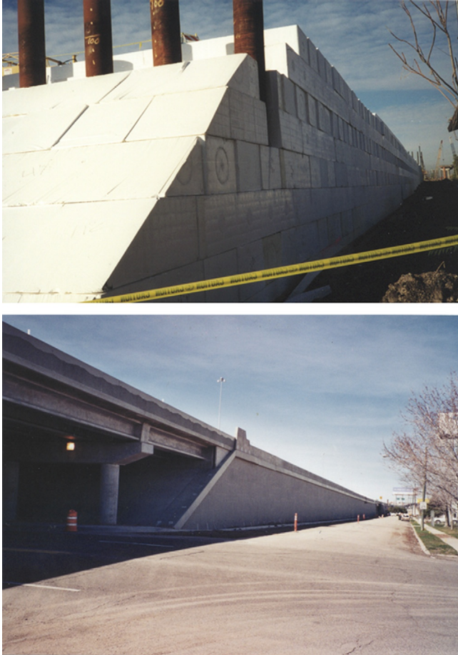
Figure 17.16 During and after construction of bridge abutment for I-15 project, Salt Lake City, UT. Courtesy of AFM Corporation.
