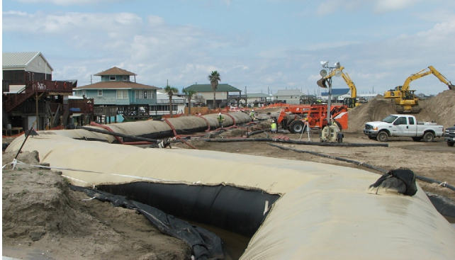
Figure 16.27 Construction of sand filled geotubes for a hurricane protection (storm surge) barrier. Courtesy of Infrastructure Alternatives, Inc.
