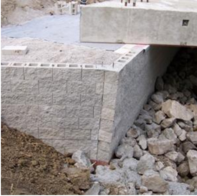
Figure 16.24 Geosynthetically reinforced wall with light concrete facing blocks. Courtesy of Federal Highway Administration.
