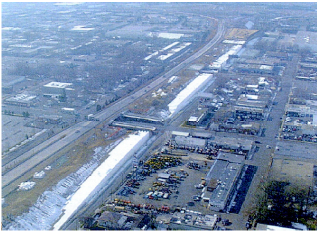
Figure 17.15 Aerial view of a portion of the I-15 project under construction, Salt Lake City, UT. Courtesy of AFM Corporation.
