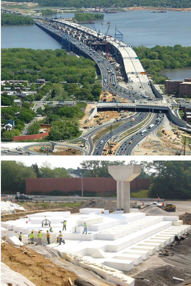
Figure 17.13 Construction of the new Woodrow Wilson Bridge, approach, and interchanges. Courtesy of FHWA.
