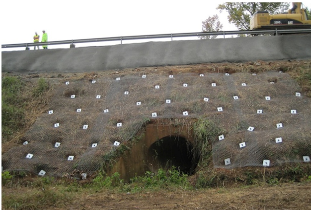
Figure 16.31 Slope stabilization incorporating anchored and tensioned netting to provide confinement. Top: After Koerner, 2005; Bottom: Courtesy of GeoStabilization International.
