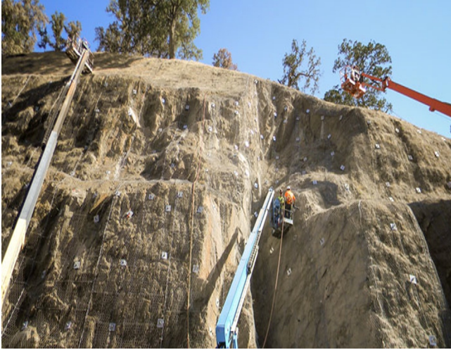
Figure 16.30 Confinement of weathered rock face with steel mesh and soil nails. Courtesy of GeoStabilization International.
