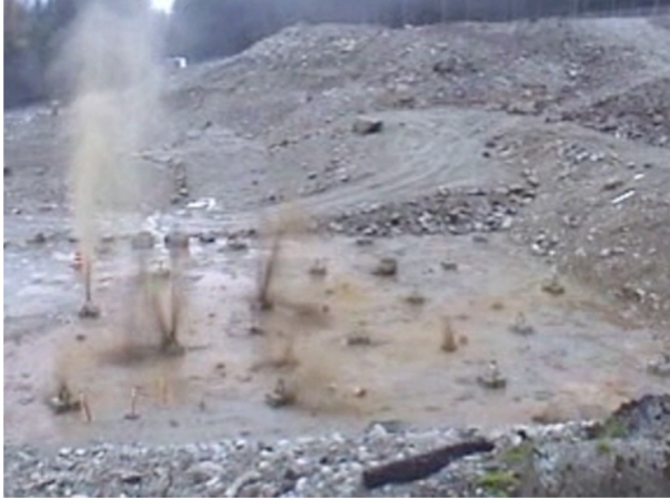
Figure 6.1 Example of field blasting showing expulsion of excess pore water. Courtesy of Explosive Compaction, Inc.
