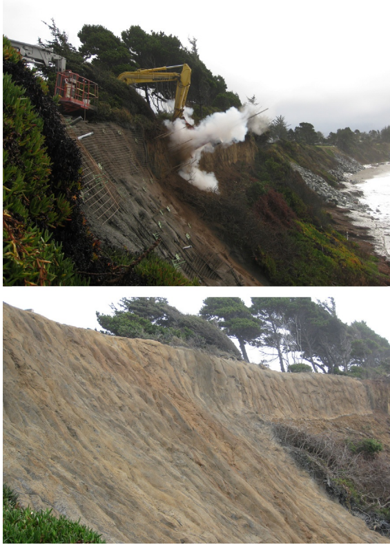
Figure 15.7 Stabilization of coastal bluff with fiberglass launched soil nails: Before and after stained shotcrete finish. Courtesy of GeoStabilization International.
