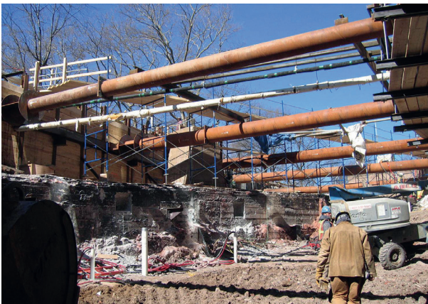
Figure 7.7 Application of ejector wells to dewater for a deep excavation at the South Ferry Terminal, NYC. Courtesy of Moretrench.
