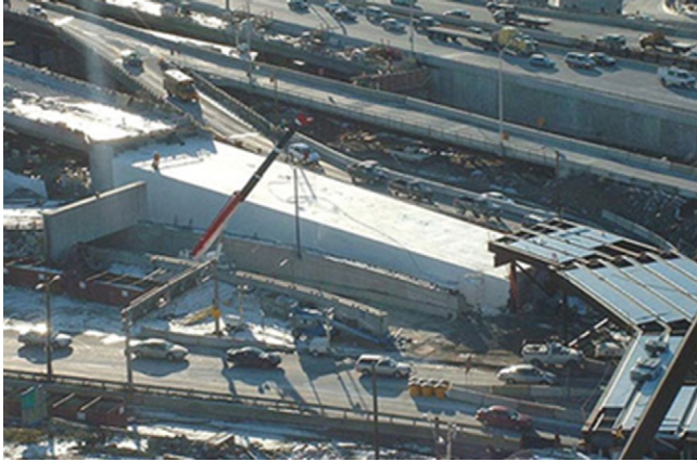
Figure 17.14 Use of Geofoam for a highway ramp as part of reconstruction of Boston's Central Artery ("Big Dig") project. Courtesy of FHWA.
