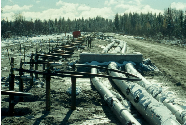
Figure 13.14 Ground freezing for (2.5 mi) perimeter barrier around the Aquarius Gold Mine, Timmins, Ontario, Canada. Courtesy of Layne Christensen.
