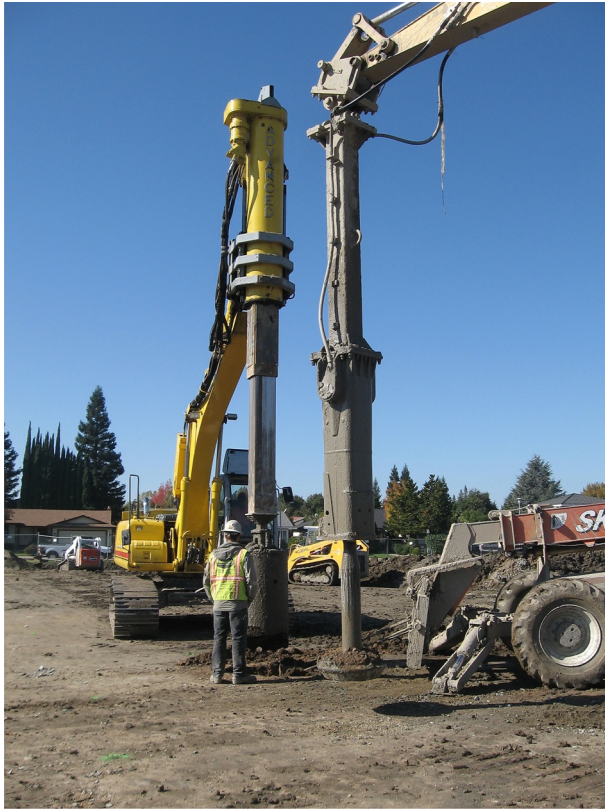
Figure 6.9 Equipment used for installation of a Rammed Aggregate Pier® system. Courtesy of Geopier Foundation Company, Inc.
