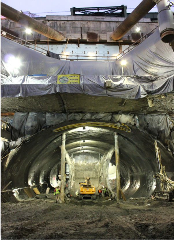
Figure 13.12 View of the complex conditions for tunneling through frozen ground beneath urban infrastructure. Courtesy of Moretrench.
