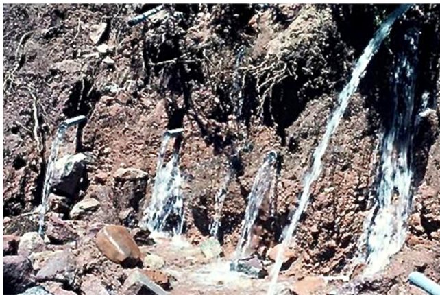
Figure 7.14 Drainage of a slope with closely spaced launched horizontal drains. Courtesy of GeoStabilization International.
