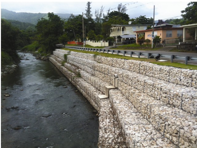
Figure 16.9 Gabion buttress walls for channel bank stabilization/protection. Top: Courtesy of Hayward Baker; Bottom: Courtesy of Maccaferri, Inc.
