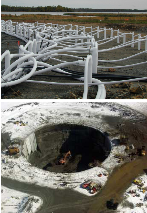
Figure 13.13 Shaft excavation in sensitive clay at Verglas mining project, Quebec, Canada. Courtesy of Layne Christensen.
