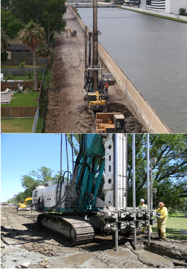
Figure 12.10 Triple axis jet grouting for rehabilitation of 17th Street levee in New Orleans, LA. Courtesy of Layne Christensen.
