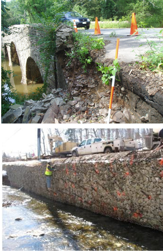
Figure 15.5 Rehabilitation of historic rock retaining walls with soil nails. Courtesy of GeoStabilization International.
