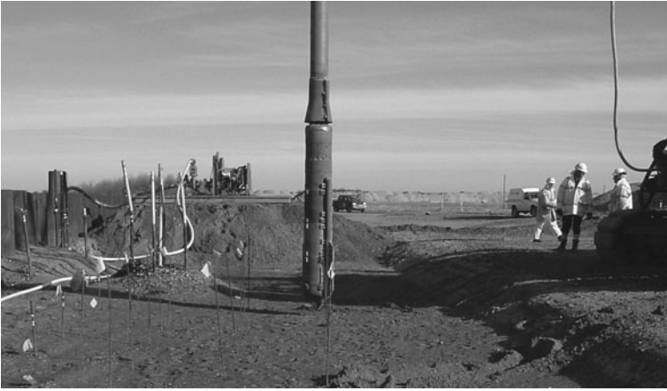
Fig. 7.22 Vibro probe used for installation of stone columns at the location in case study in Section 7.2.2.1
