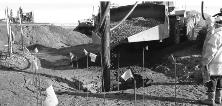
Fig. 7.23 Stone backfill about to be poured around a vibratory probe to create a stone column. The bars with flags mark positions of the stone columns yet to be placed
