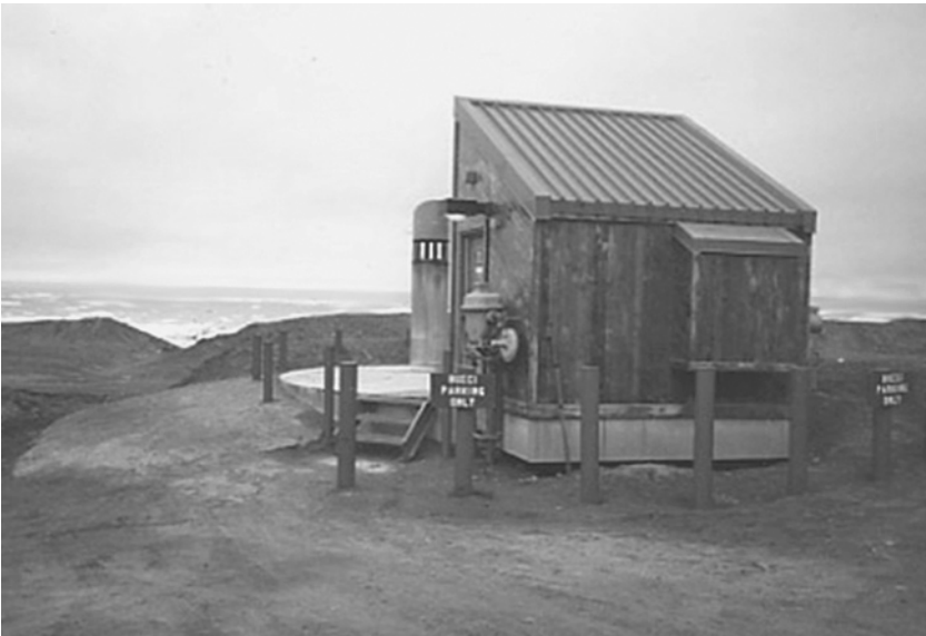
Fig. 3.11. Utilidor Pump Station No. 4 protected by temporary berms from the Arctic Ocean in the background. Photo: Ron Brunner.
