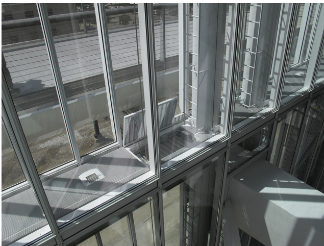
Figure 7.9 Glazed double-skin facade, interior view, Chicago Art Institute, RPBW, Chicago. Photo by the author.
