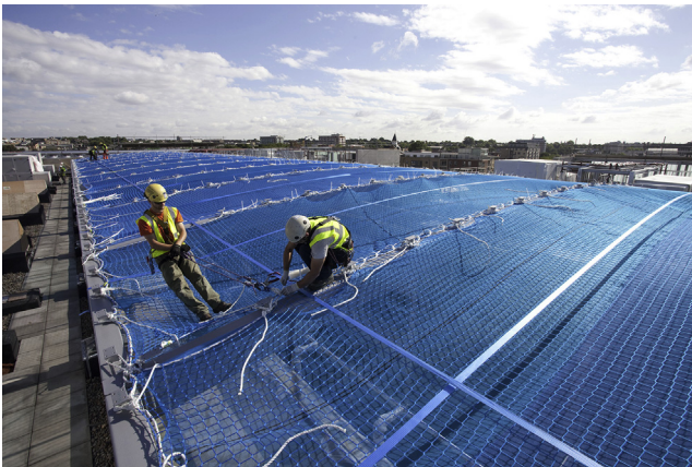
Figure 7.26 ETFE roof installation, King's Cross Station, London. Courtesy of John Sturrock/Vector Foiltec ©.
