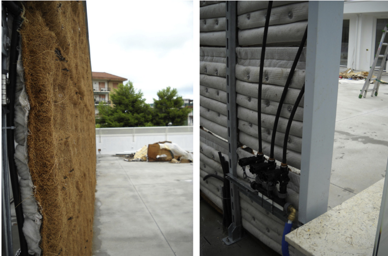
Figure 6.11 Living wall growing felt and irrigation system. Courtesy of Poliflor s.a.s.
