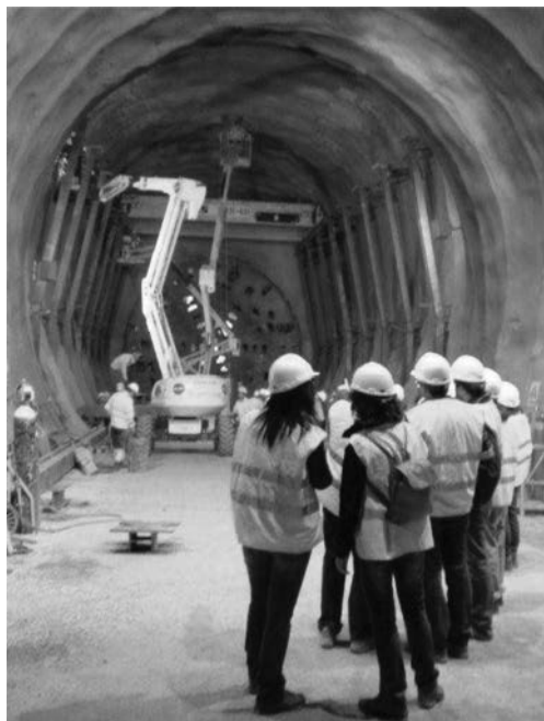
Figure 4. Illustration of disassembly operations of TBM inside the tunnel. The TBM cutting face is shown in the background; note the cavern excavated with dimensions slightly larger than the TBM diameter, and the auxiliary structure for the bridge crane.
