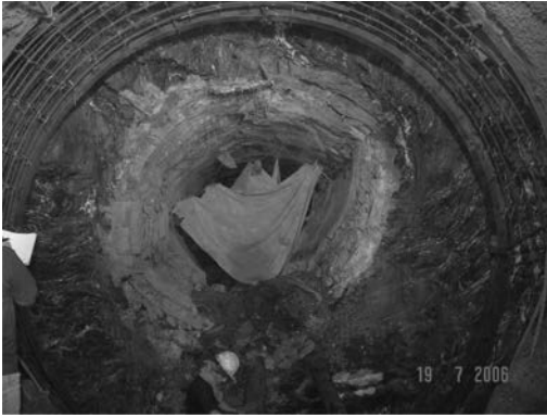
Figure 7. Large convergences at Yacambú-Quíbor tunnel. (Courtesy of Ing. V. Camejo.)
