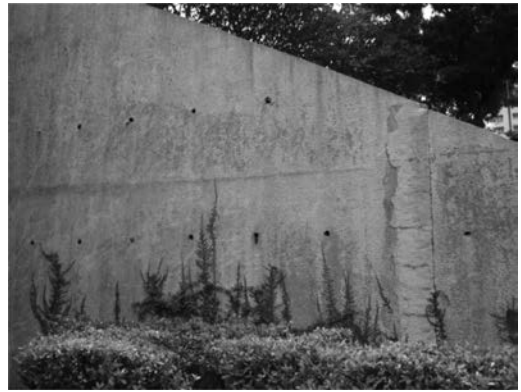
Figure 4. Photograph of a reinforced concrete cantilever retaining wall in campus taken by a student.
