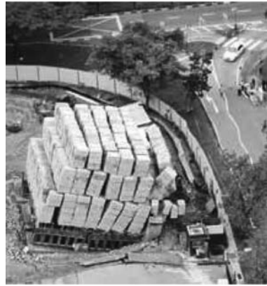
Figure 7. Photograph of failure of pile load test setup (Channel NewsAsia, 2010).
