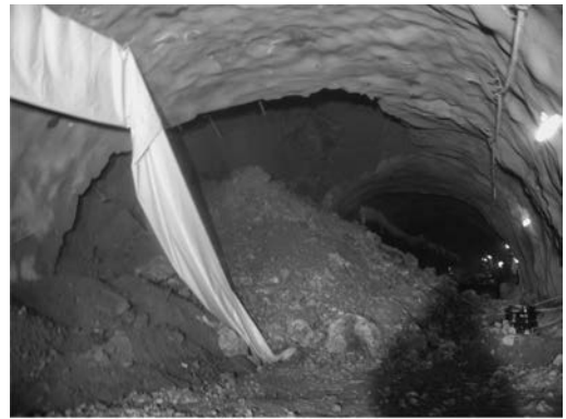
(a) Initial collapse
