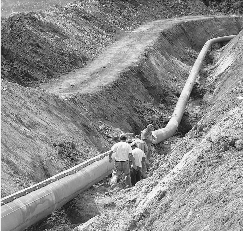
14.1 Continuous gas steel pipeline with welded joints (Glisic and Inaudi, 2007). (Source: Courtesy of SMARTEC.)
