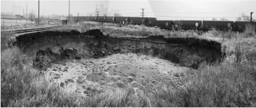
13.8 Sinkhole formation. (Source: Picture courtesy of Burns and McDonnell.)
