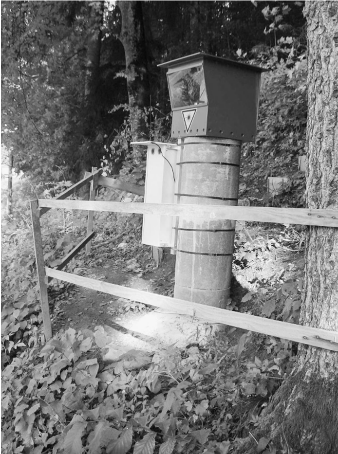
13.15 Robotic laser distance meter installed on a pillar. (Source: Picture courtesy SMARTEC SA and EPFL.)
