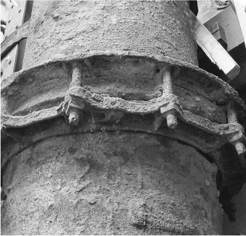
14.4 Externally corroded pipeline with flanged joint.
