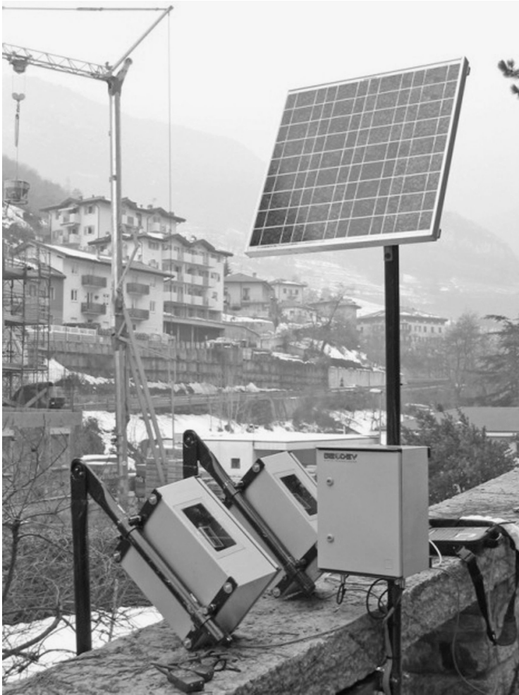
13.3 Laser distance meters, with protective housing, control system, and solar power supply. (Source: Picture courtesy SMARTEC SA.)
