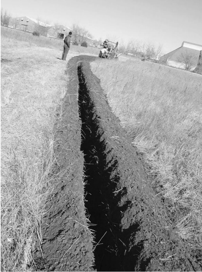
13.9 Digging of a trench to install the distributed sensing cable. (Source: Photo courtesy of SMARTEC.)
