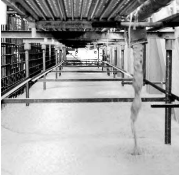
Figure 7.7 Multiple discharge points when casting SCC for anchorage blocks of the Akashi-Kaikyo bridge, Japan.
