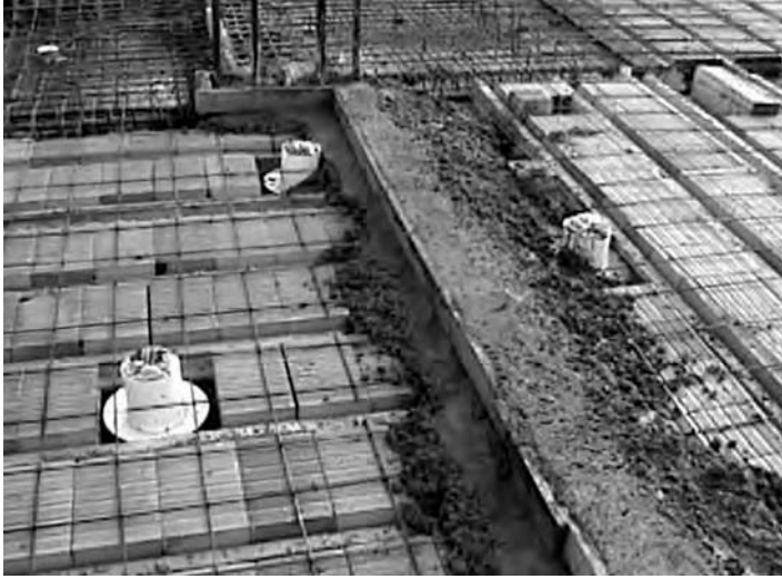
Figure 13.9 Low dividing 'wall' of TVC in order to prevent SCC flowing into the neighbouring section of the floor slab [4] .
