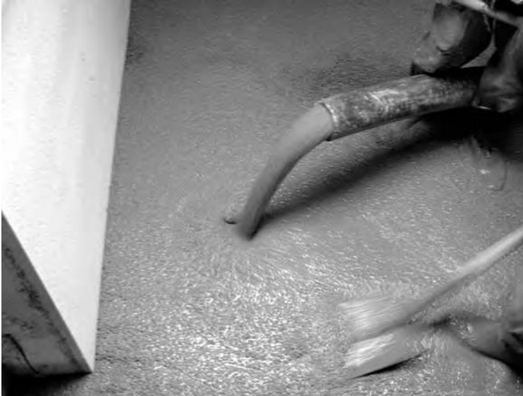
Figure 13.20 Casting of in situ LWSCC during renovation of an existing building. Note the ‘cohesion’ of the mix. (Reproduced with permission of R Hela and M. Hubertova.)
