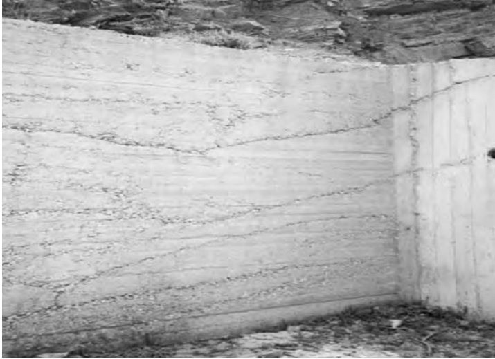
Figure 2.1 Honeycombing and many 'cold' joints. Poorly compacted concrete.
