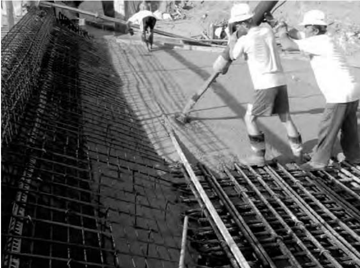
Figure 7.8 Casting of a heavily reinforced deep bridge deck using SCC. (Reproduced with permission of J.L. Vitek, Metrostav a.s.)
