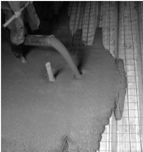
Figure 7.4 A typical case of one man placing SCC in situ. (Reproduced with permission of R. Hela and M. Hubertova.)
