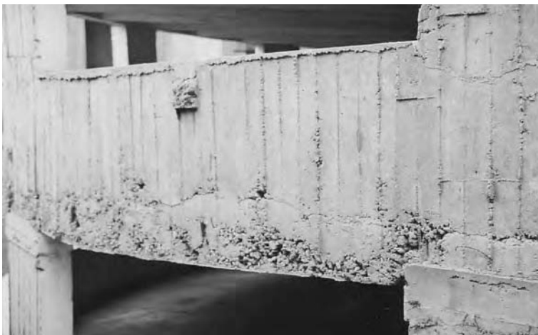
Figure 2.2 Poor compaction of the lower part of a reinforced concrete beam. Severe honeycombing is clearly visible. Bottom reinforcement is poorly protected against corrosion.
