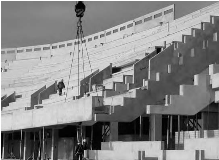
Figure 13.19 Erection of a stand at Wolfsburg using lightweight aggregate SCC. (Reproduced with permission of R Heila and M. Hubertova.)
