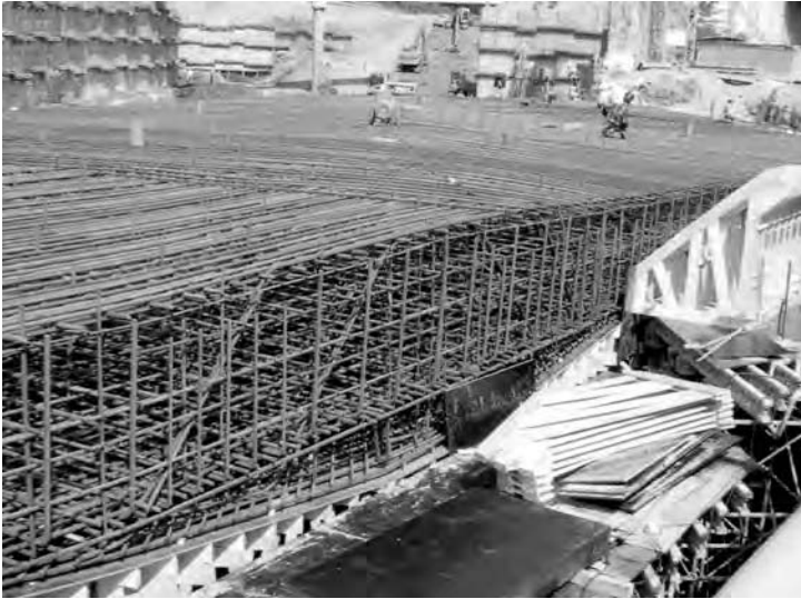
Figure 12.5 Heavily reinforced bridge deck: It was impractical to concrete it using TVC, SCC had to be used. (Reproduced with permission of J.L. Vitek, Metrostav a.s.)
