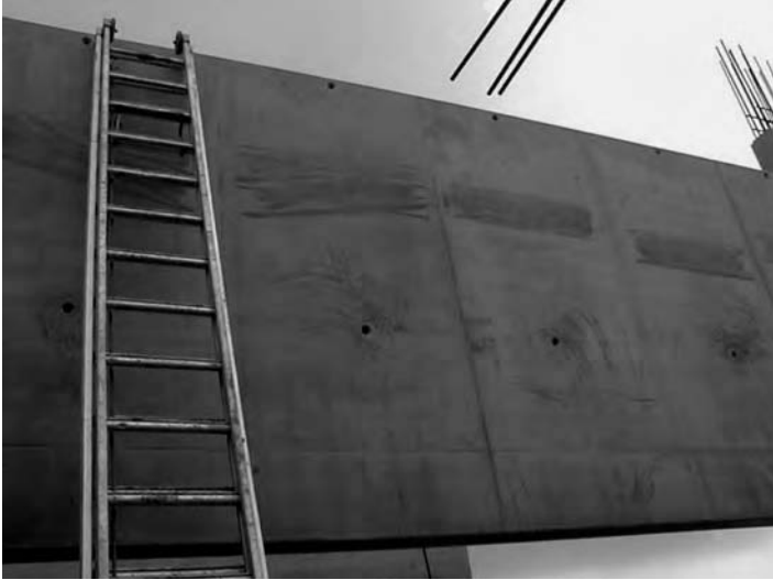
Figure 13.5 Finished surface, showing black traces due to magnetisation of the formwork linked to the use of fly ash in the SCC.
