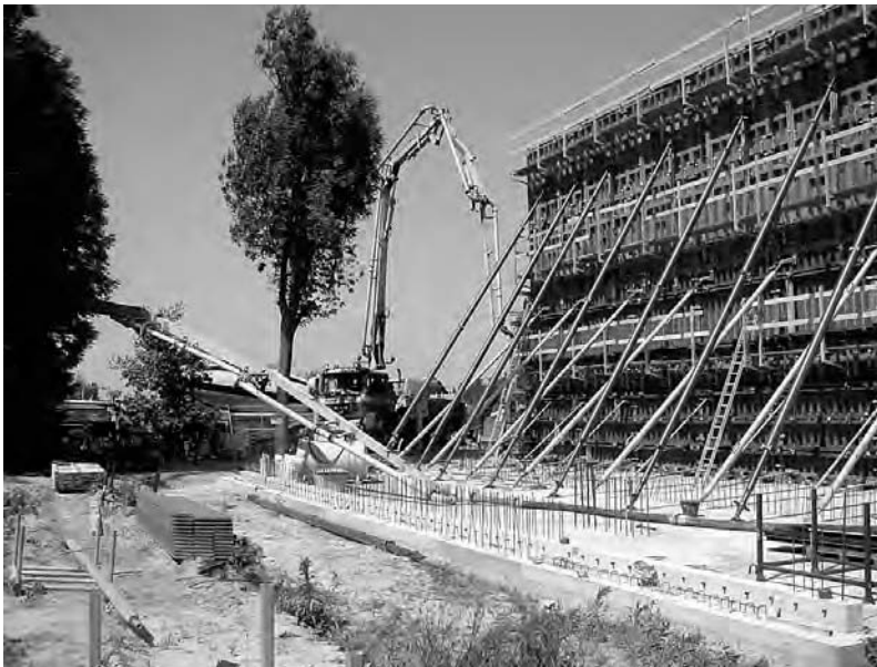
Figure 13.16 Filling the formwork from beneath, with two inlet points. (Reproduced with permission of Engineering Office Mouton, Ghent, Belgium.)
