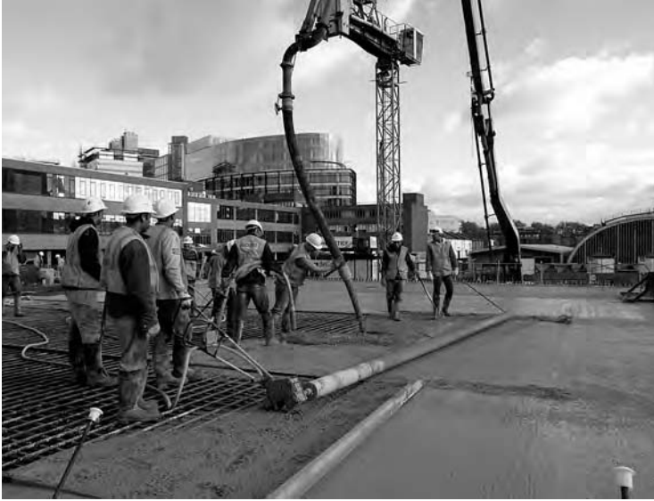
Figure 2.4 Placing and finishing of TVC (2004). (Reproduced with permission of The Concrete Society.)
