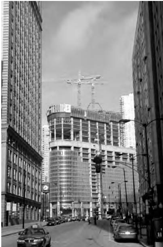
Figure 13.12 Progress in the construction of the Trump tower as of February 2007 [5] . (Reproduced with permission of Skidmore, Owings & Merrill LLP.)
