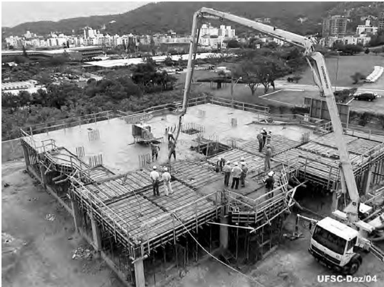
Figure 13.8 Application of SCC for slabs and beams of a building floor. Note that only two men are actually engaged in placing the SCC [4] .
