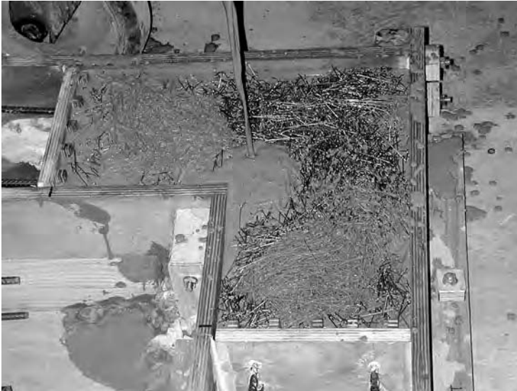
Figure 2.8 Pouring of a highly fluid but cohesive slurry to produce a ‘SIFCONised’ knee joint in a concrete frame without vibration. The rest of the frame was cast using ‘ordinary’ SCC (after Svermova et al. [8] ).
