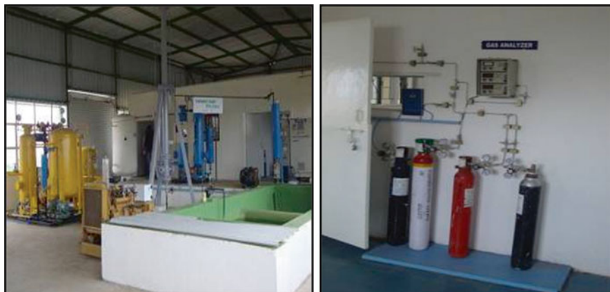
Fig. 10 Water scrubbing and PSA system ( Left ) and Gas analyser system at Nasik ( Right )
