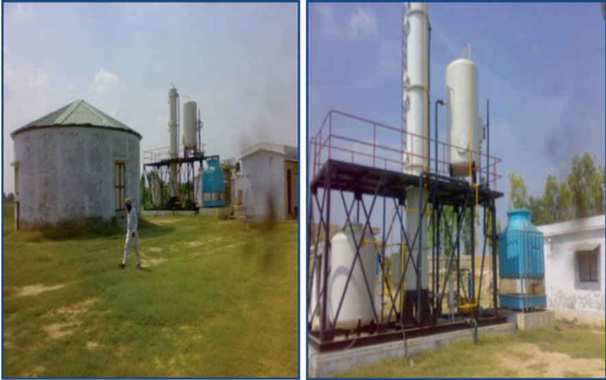
Fig. 11 Biogas plant ( Left ) and Upgradation plant at Abohar ( Right )
