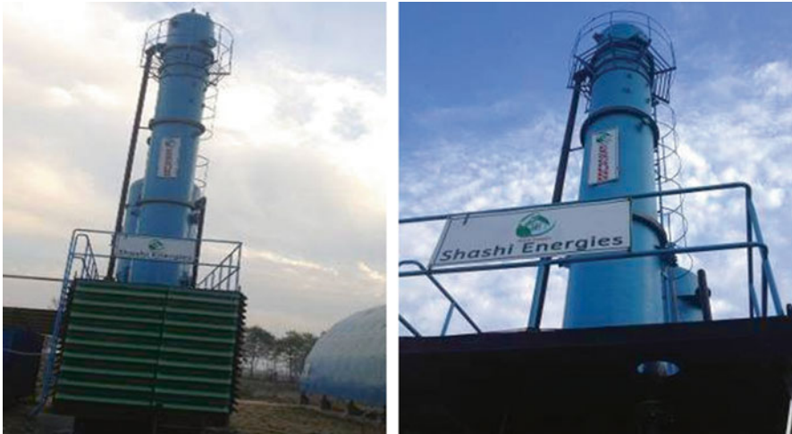
Fig. 12 50 m 3 /h low pressure water scrubbing tower
