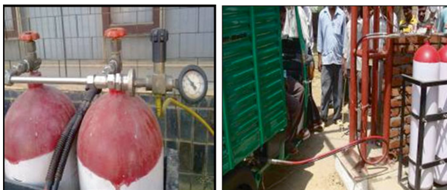
Fig. 8 Simple low cost upgraded biogas dispensing system
