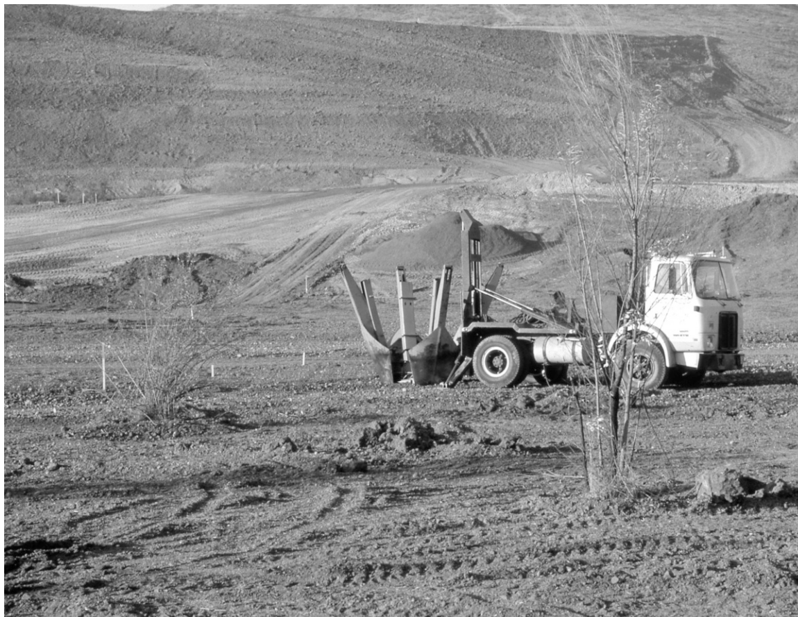
FIGURE 10-3. A “tree spade” digging a receiving hole for a willow tree. More than two thousand translocated willow and cottonwood trees were placed on this site with a less than 1 percent mortality rate; the trees were salvaged from a construction project upriver. (Photo by John Rieger.)
