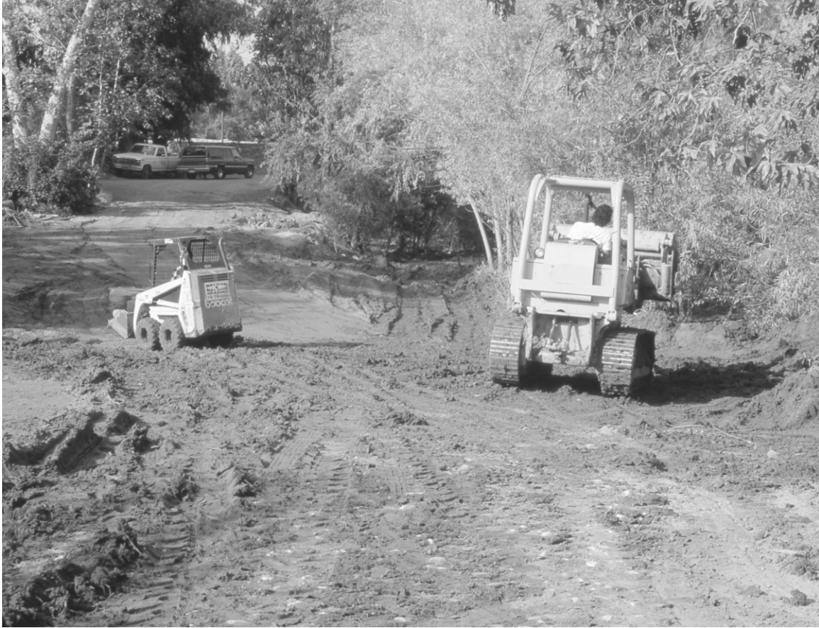
FIGURE 10-2. Small vehicles can be very useful in small areas requiring extensive earth moving. This is removal of sediment caused by illegal grading upstream. Orange County, California. (Photo by John Rieger.)
