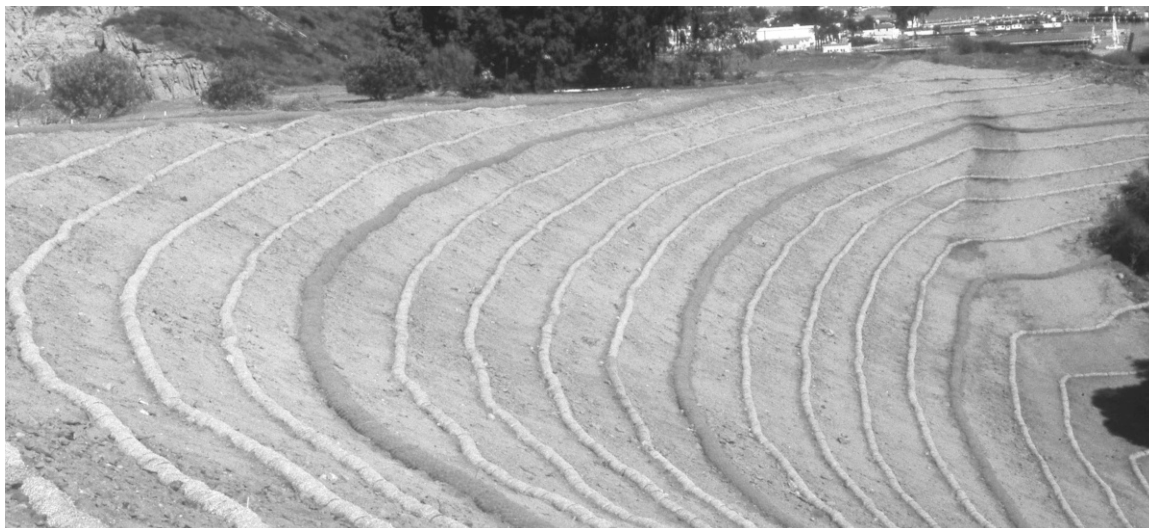
FIGURE 10-9. A site with freshly installed straw wattles and coconut fiber wattles (darker wattle) for stabilization. Coconut fiber wattles last much longer than straw. This approach was an insurance backup measure in case the initial seeding was not effective. Naval Base Point Loma, San Diego, California. (Photo by Mary F. Platter-Rieger.)
