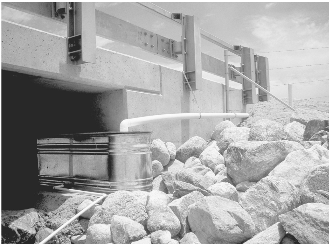
FIGURE 7-3. A storage and gravity distribution system provides water in the Colorado desert. A cattle trough has been placed under a bridge abutment to provide gravitational head. The water travels through PVC pipes to buried unglazed clay pots. (Photo by David A. Bainbridge.)
