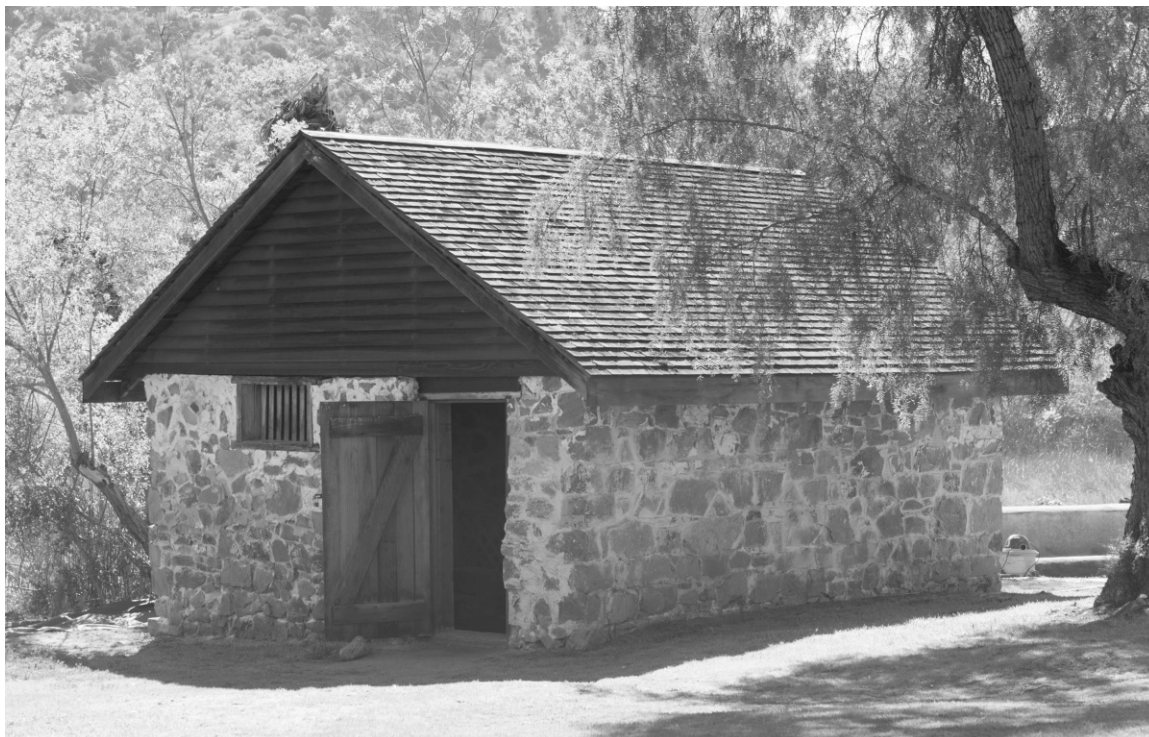
FIGURE 14-3. Now restored, more than forty volunteer palm trees were damaging the historic Spring House. Removal of these palm trees was a project requirement placed by the County Parks Department, San Diego, California. (Photo by Mary F. Platter-Rieger.)
