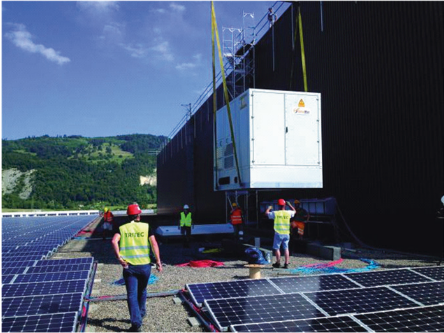
Fig. 1.7 A photograph of step-up transformer installation of Tritec 5.2 MW solar PV power plant [30]
