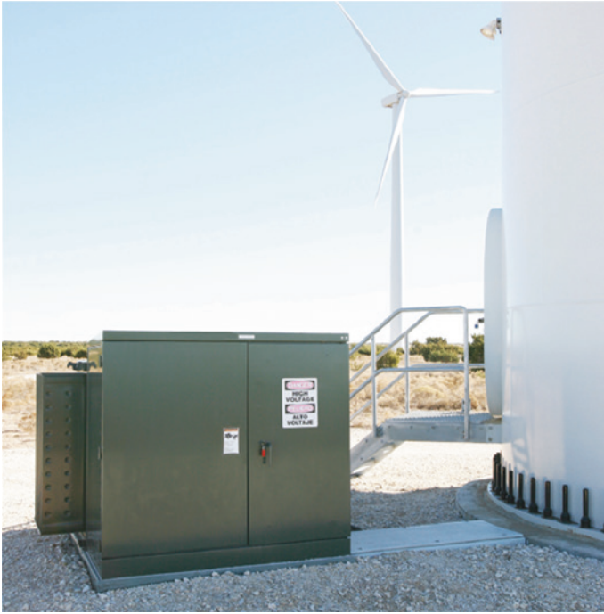
Fig. 7.16 Housing of liquid-filled transformer in onshore wind farm
