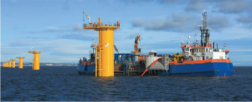
Fig. 1.4 A photograph of installation process of offshore wind power plant with the vessel Aeolus [24]
