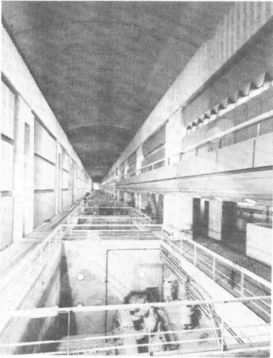
Fig. 5.6 Rance River plant power station: interior view
