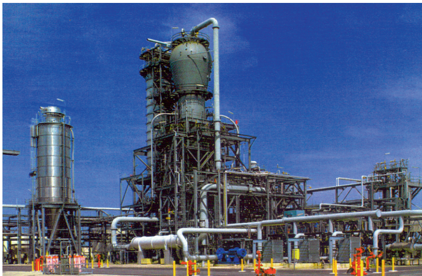
Figure 8.1. Unipol/Dow plant for the production of polyethylene. The key unit in the polyolefins plant is the Unipol reactor, which is the largest of its type in the world. Reproduced with permission from Univation Technologies, a Joint Venture between ExxonMobil Chemical and Dow Chemical.
