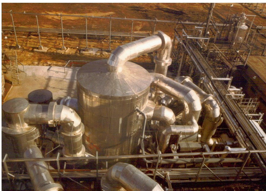
Figure 2.2. Modern sulfuric acid plant using the contact process.
