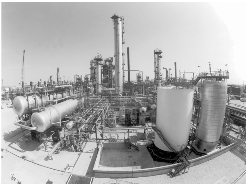
Figure 6.1. Alkylation plant near Port-Jérôme, France. Reproduced with permission from ExxonMobil Research and Engineering Company.
