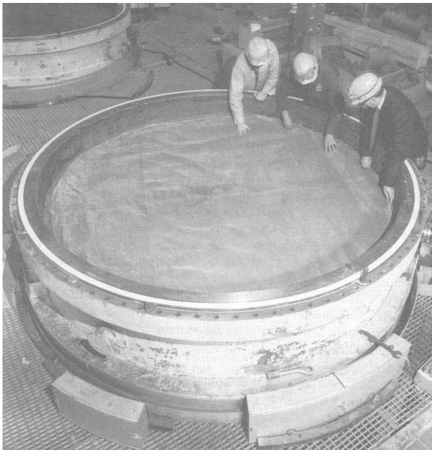
Figure 4.5. Installation of platinum gauze pad in a nitric acid plant—checking for wrinkles. Reprinted from Catalyst Handbook , 2 nd ed., by kind permission of M. Twigg.
