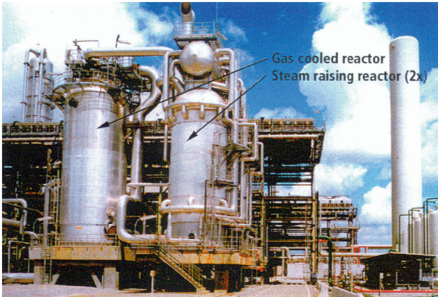
Figure 10.9. Lurgi reactor for a low-pressure methanol synthesis plant. Reproduced with permission from Lurgi Aktiengesellschaft.
