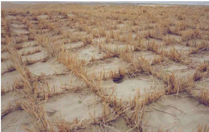
Fig. 8.7. The wheat straw checkerboard barriers equipped on either side of a road to protect it from sand-burying (photo by the author et al. in Dunhuang, China)
