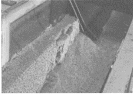
Figure 5. Bank erosion resulting from intermittent block failure.
