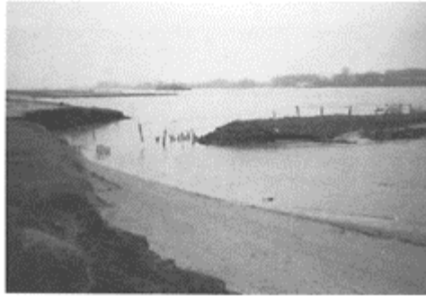
Photograph 1. Outflanked groyne in the Waal river.
