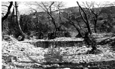
Figure 7. Existing sediment control drop structures in the mountainous area filled with sediment.
