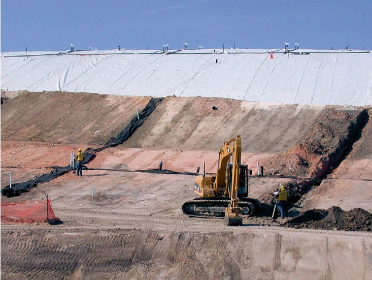
Fig. 13.21 Construction of surface trenches for gas collection to be placed under an exposed geomembrane cap
