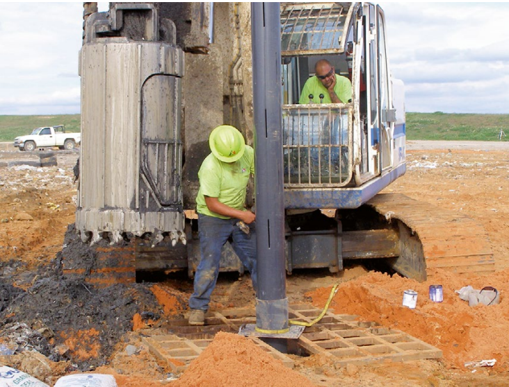
Fig. 13.4 Placement of slotted well pipe into excavated borehole (Photo courtesy of Jones Edmunds)
