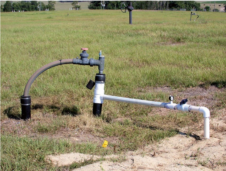
Fig. 6.8 Connection of liquids addition manifold to surface trench
