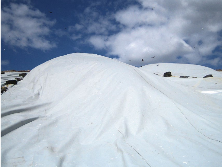
Fig. 13.11 Ballooning of geomembrane at the landfill surface as a result of gas pressure
