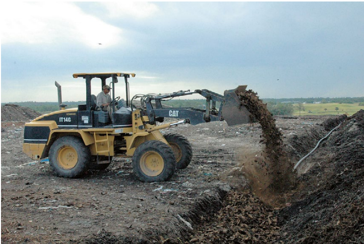
Fig. 9.5 Placement of shredded tires on top of HDPE liquids distribution pipe in horizontal trench
