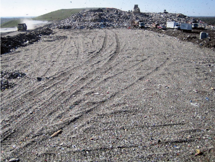
Fig. 9.16 A horizontal drainage blanket of crushed glass installed on a landfill lift
