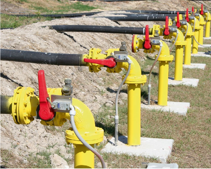
Fig. 6.7 Hydrant system for delivering liquids to specific addition devices in a landfill
