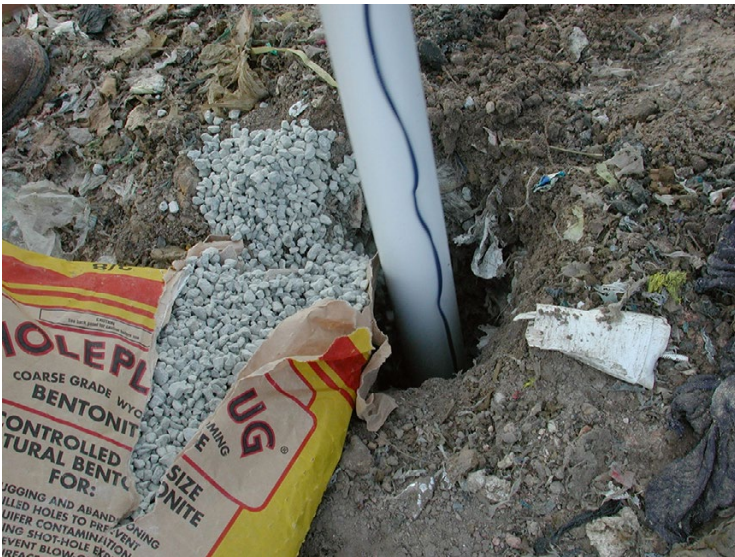
Fig. 8.10 A collar of bentonite (clay) being added to the annulus at the surface of a recently constructed liquids addition well
