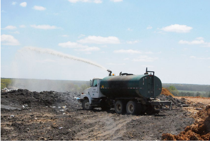
Fig. 7.2 Spray application of leachate at the landfill surface using a tanker truck (Photo courtesy of John Schert)
