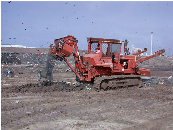
Fig. 9.13 Trenching machine used for installing horizontal injection pipe into the surface of a landfill lift
