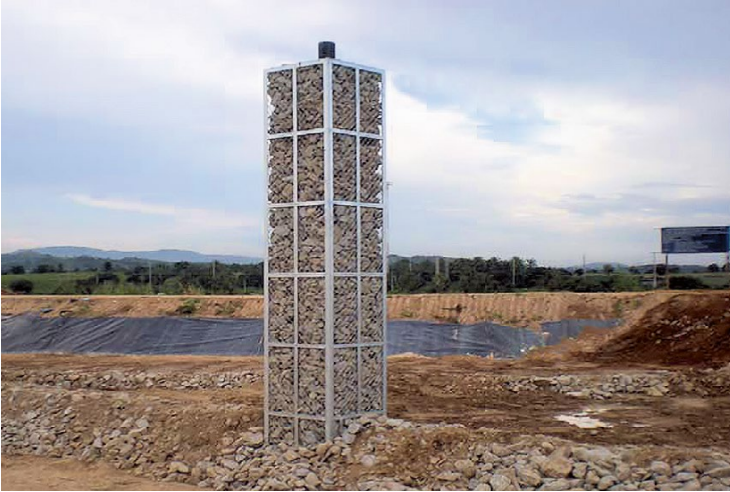
Fig. 14.12 Vertical vent of a semi aerobic landfill after construction and before waste filling
