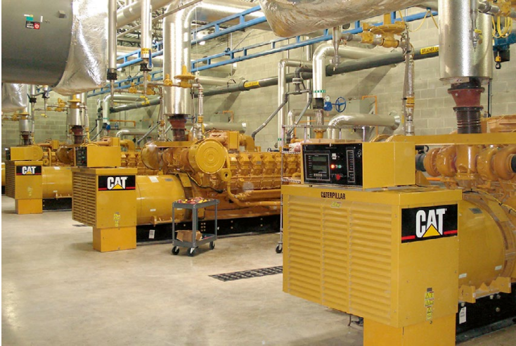
Fig. 19.2 Internal combustion engine for converting landfill gas to electricity
