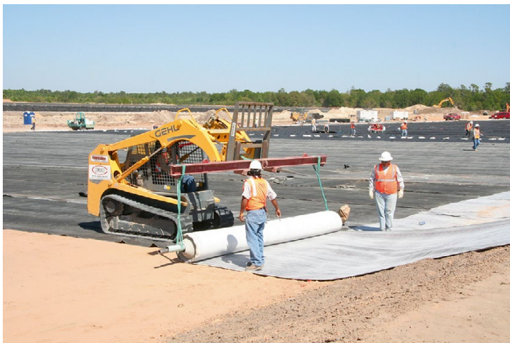
Fig. 1.7 A barrier layer being placed as part of the construction of a landfill liner and leachate collection system
