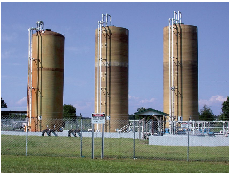
Fig. 11.15 Fiberglass leachate storage tanks surrounded by secondary containment system
