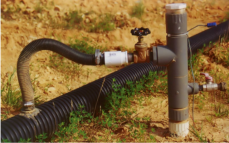
Fig. 14.18 Distribution manifold and air addition well for an aerobic landfill in the Southeast US
