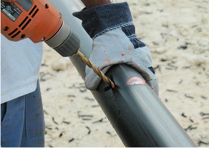
Fig. 9.11 Drilling orifices in HDPE liquids injection pipe
