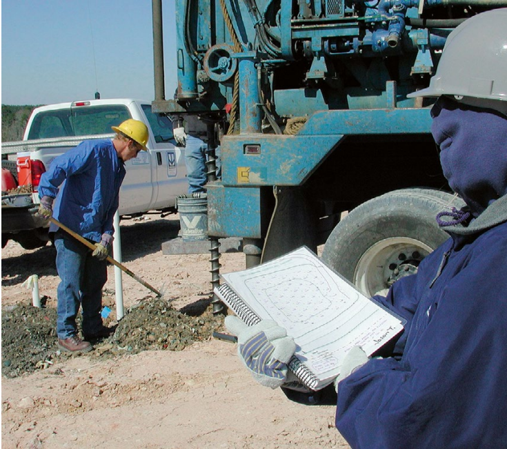
Fig. 8.9 Careful recording of auger depth into the landfill is critical to avoid damage to the bottom liner system
