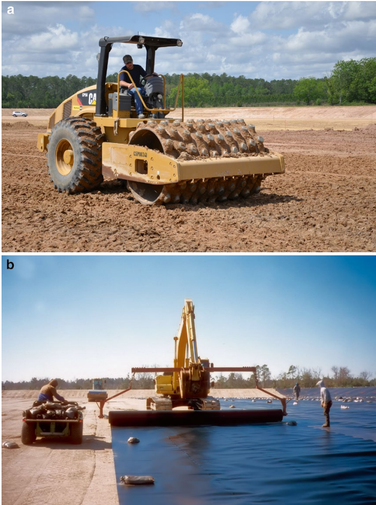
Fig. 2.6 (a) Construction of compacted earthen liner. (b) Geomembrane liner panels. (c) Thermal fusion welding of geomembrane panels. (d) Thermal extrusion welding of geomembrane (Photo courtesy of Jones Edmunds)
