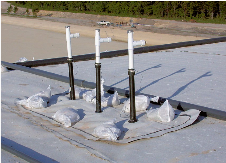
Fig. 4.12 Cluster of vertical wells at NRRL after construction and prior to liquids or air addition
