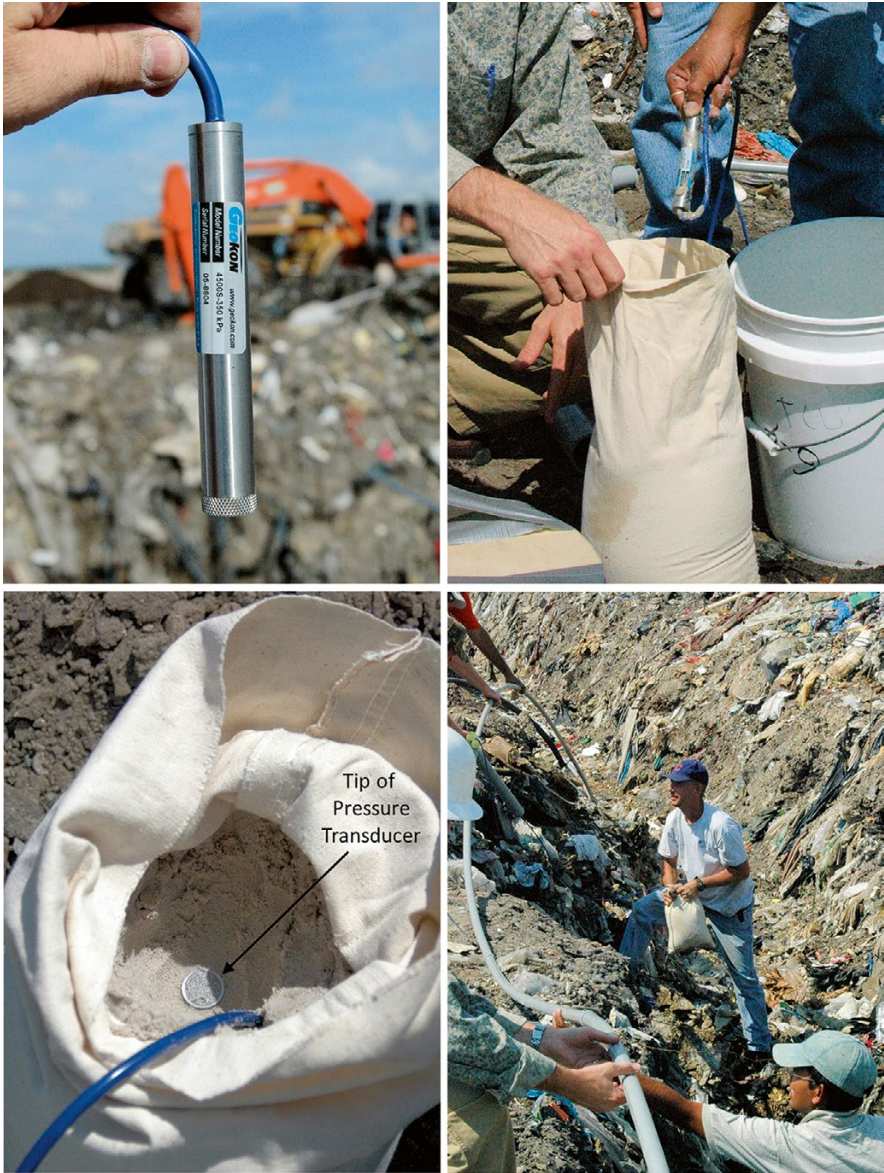
Fig. 16.19 Pressure transducers for measuring internal landfill pore pressures installed by burying in sand-filled bags within the waste as filled
