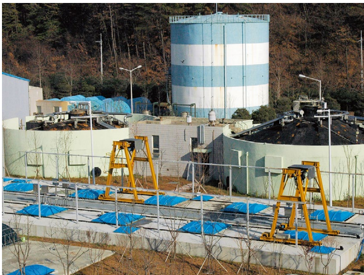
Fig. 11.17 On-site leachate treatment plant consisting of multiple biological and physical treatment operations
