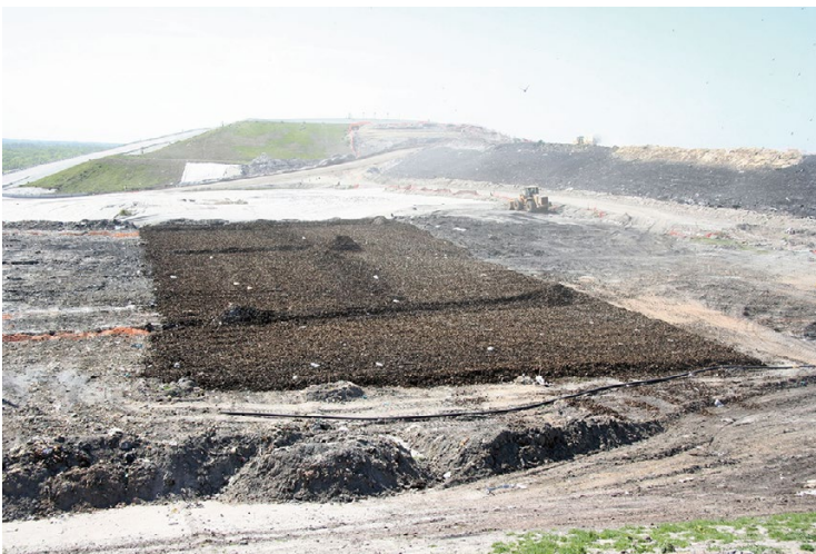
Fig. 9.17 A horizontal drainage blanket of shredded tires installed on a landfill lift
