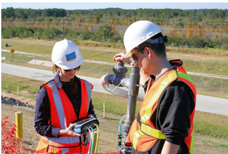
Fig. 15.5 Collecting gas data as part of GCCS operation
