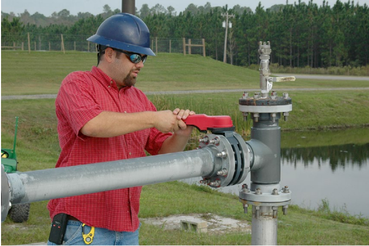
Fig. 15.2 Adjusting valves as part of liquids addition system operation
