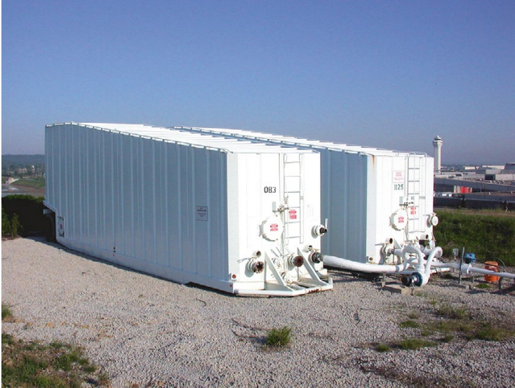
Fig. 6.6 Tank container chassis used for the storage and gravity discharge of leachate to a liquids distribution system on top of a landfill
