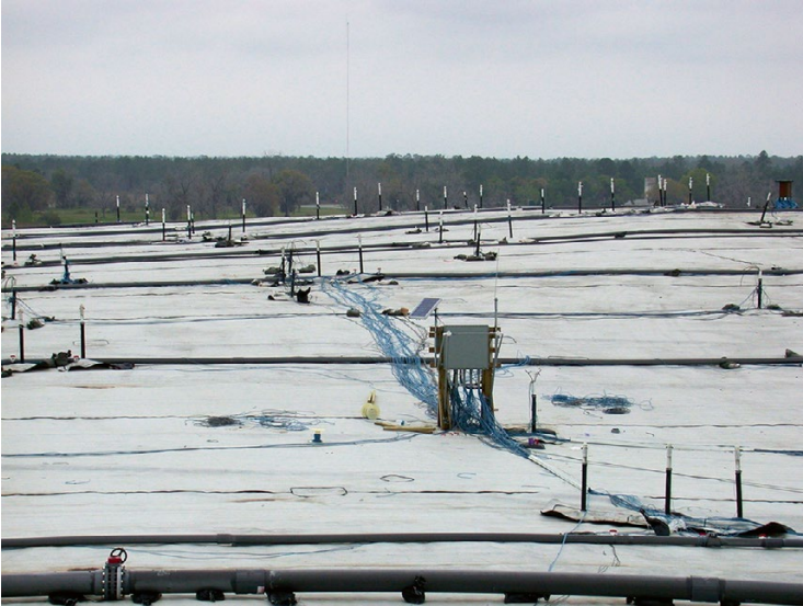
Fig. 4.13 Vertical well field at NRRL
