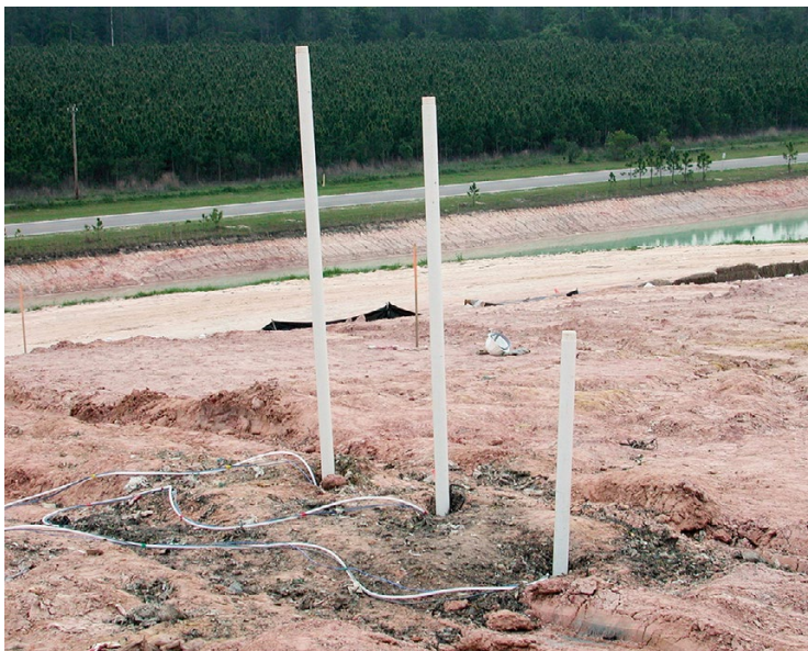
Fig. 4.14 Recently augered cluster of boreholes with instruments placed at bottom of borehole. Each instruments bundle was temporarily attached to the end of a pipe
