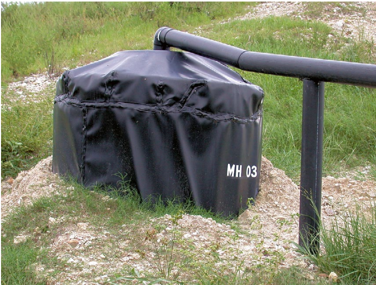
Fig. 13.16 Manhole of LCRS sealed with HDPE geomembrane and plumbed for gas collection
