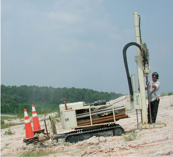
Fig. 8.5 Direct push rig installing vertical wells at the surface of a landfill
