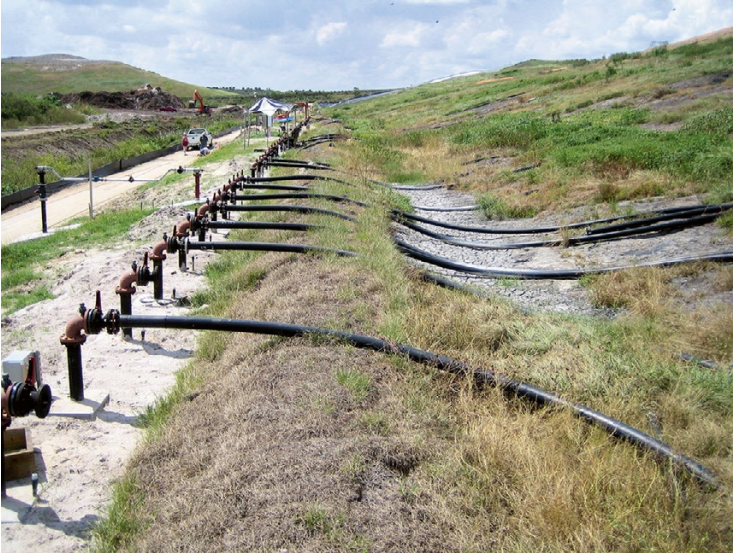
Fig. 4.23 Delivery pipes transmitted liquids from manifold system to individual horizontal trenches at PCNCL
