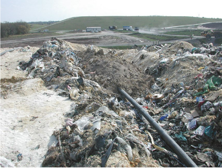
Fig. 9.15 Clay seepage collar construction at the end of a horizontal injection trench where pipe perforations start
