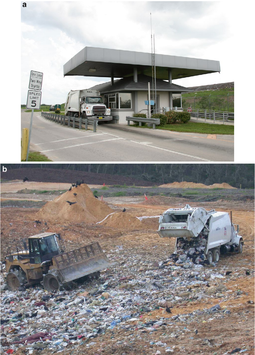
Fig. 2.10 (a) Trucks carrying waste that enter the site for disposal are first weighed using scales and appropriate information is recorded for billing. (b) Waste vehicles directed to dedicated disposal areas within the waste containment unit. (c) Spotting incoming waste. (he ) Monitoring the gas system
