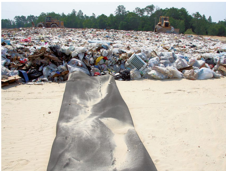
Fig. 13.20 Horizontal gas collector (perforated pipe blanketed in a geocomposite) placed on top of the LCRS drainage blanket
