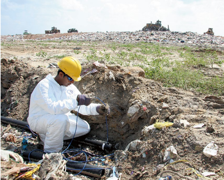
Fig. 4.18 Installation of a vibrating wire pressure transducer into a buried vertical well at NRRL
