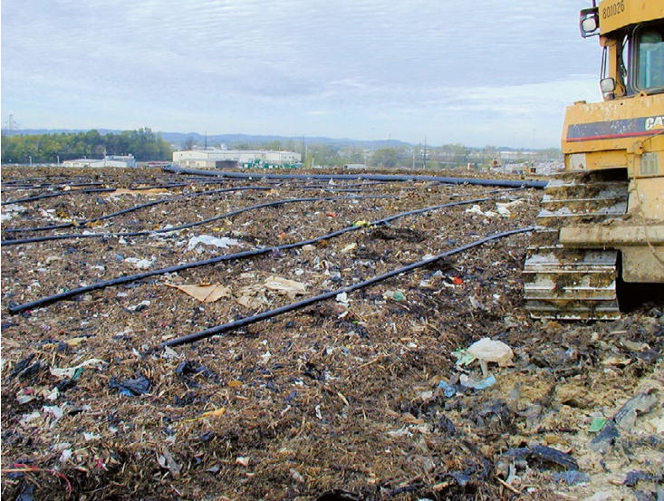
Fig. 7.4 Drip irrigation piping for liquids distribution at the landfill surface (Photo Courtesy of Waste Management Inc.)
