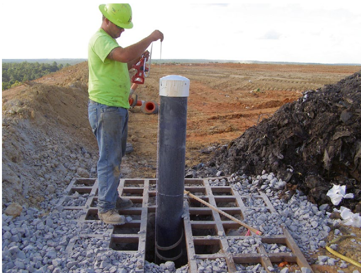
Fig. 13.5 LFG well under construction, including protective grate and well pipe; the contractor is measuring the depth of the granular fill surrounding the pipe (Photo courtesy of Jones Edmunds)
