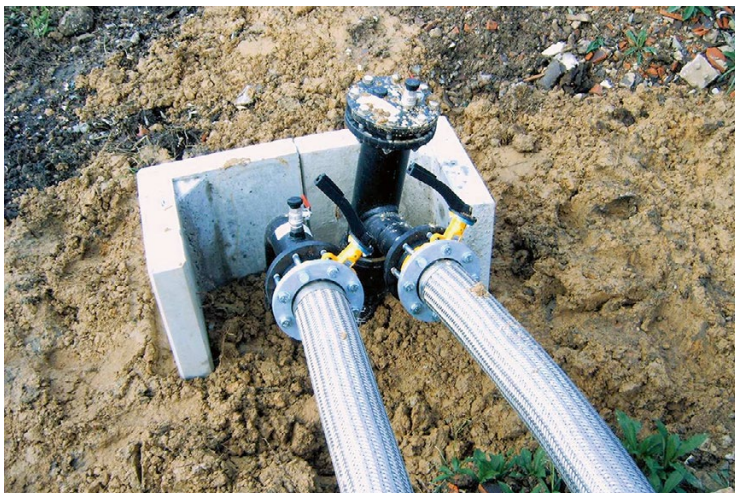
Fig. 14.13 Inlet point for air addition and gas extraction at a closed landfill undergoing aerobic treatment (Photo courtesy of Marco Ritzkowski)
