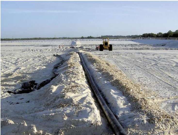
Fig. 13.19 Horizontal gas collection trench (perforated pipe bedded in stone) installed on top of the LCRS drainage layer (Photo courtesy of Jones Edmunds)
