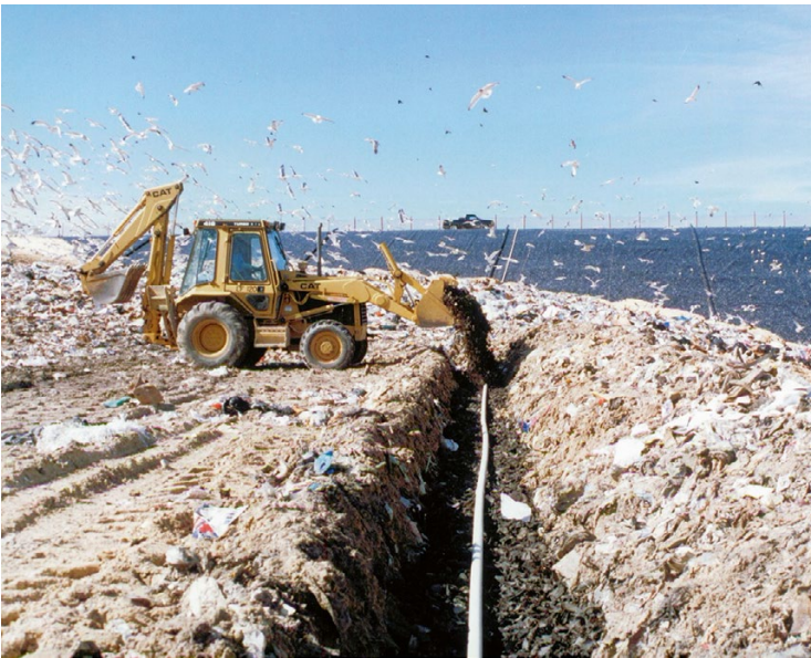
Fig. 9.10 Placement of shredded tires in liquids addition trench on top of PVC pipe
