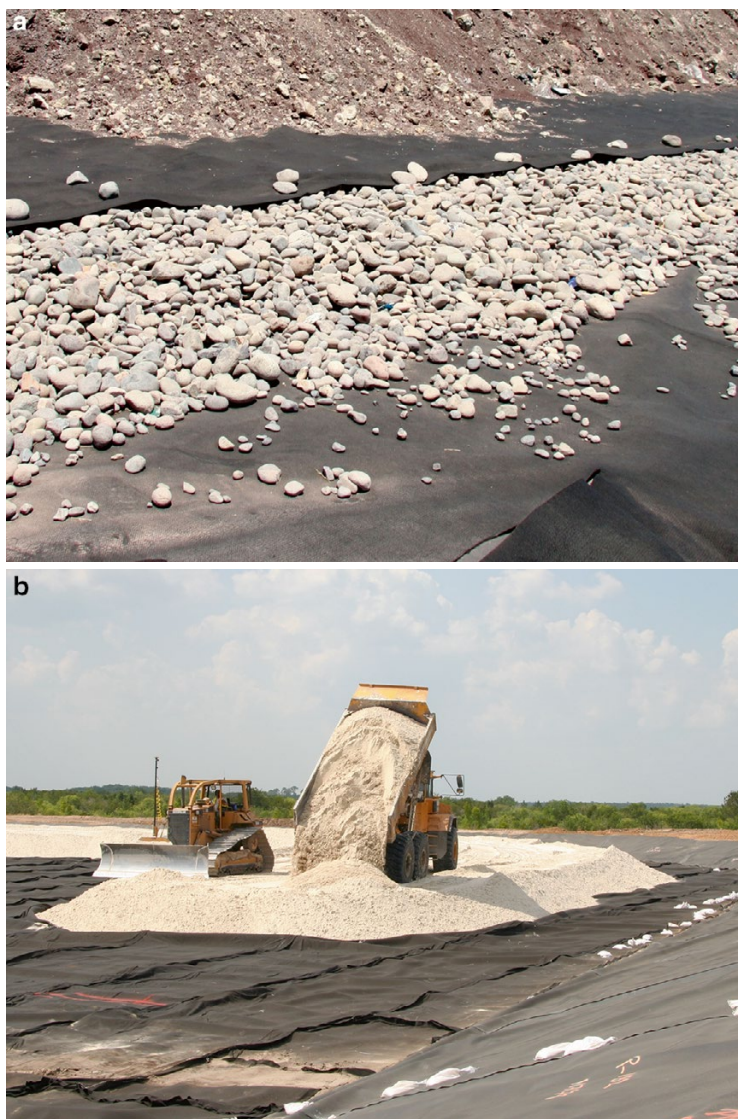
Fig. 2.7 (a) Rounded stone used as LCRS drainage material. (b) Sand placement for LCRS. (c) Geonet installation in LCRS. (d) Leachate pump station
