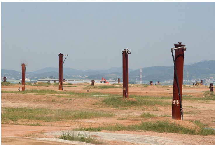
Fig. 13.23 Example of vertical gas well constructed from the LCRS and extended upward as waste depth increases
