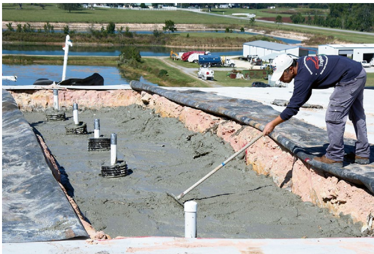
Fig. 8.18 Installation of a concrete collar around a nest of vertical injection wells
