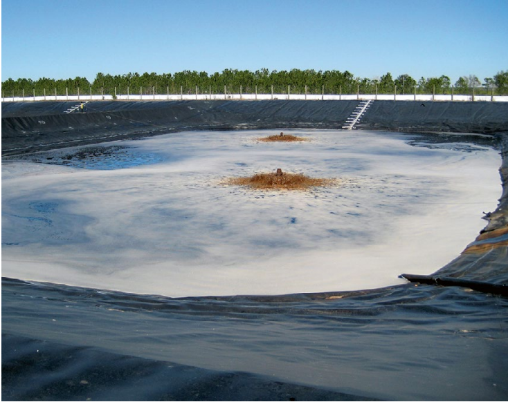
Fig. 11.13 HDPE lined leachate storage pond equipped with floating aerators
