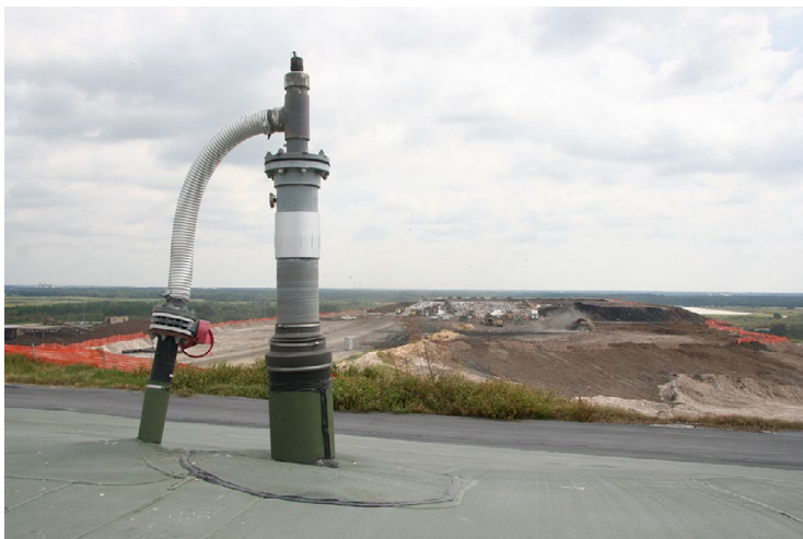
Fig. 1.8 In foreground, a gas collection well is used to extract and control landfill gas for older waste, while in the background, new waste disposal continues
