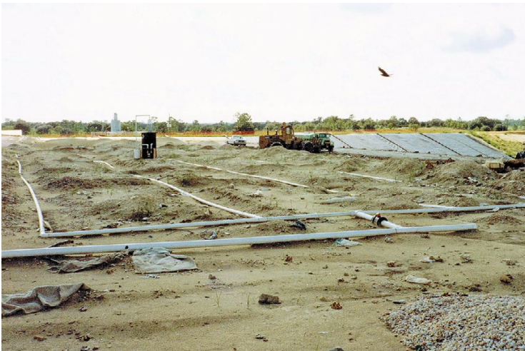
Fig. 4.2 Original surface drip irrigation system at ACSWL
