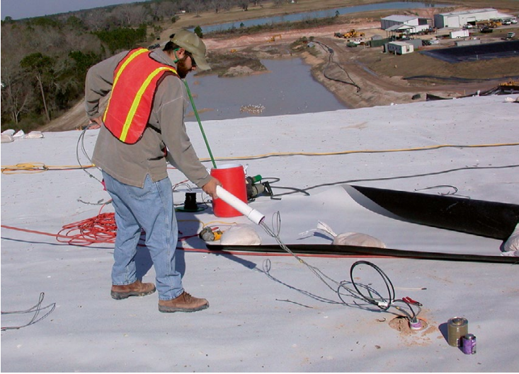
Fig. 4.16 Instrument cable routing through the geomembrane
