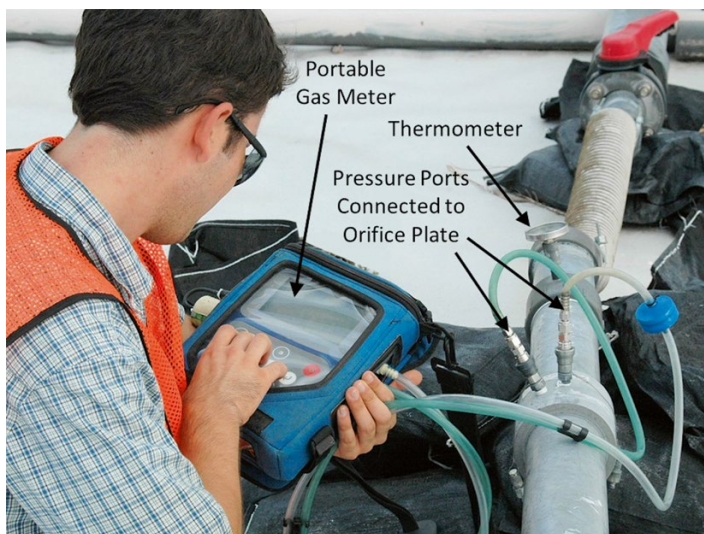
Fig. 16.7 Measurement of landfill gas flow rate as a wellhead using a portable meter
