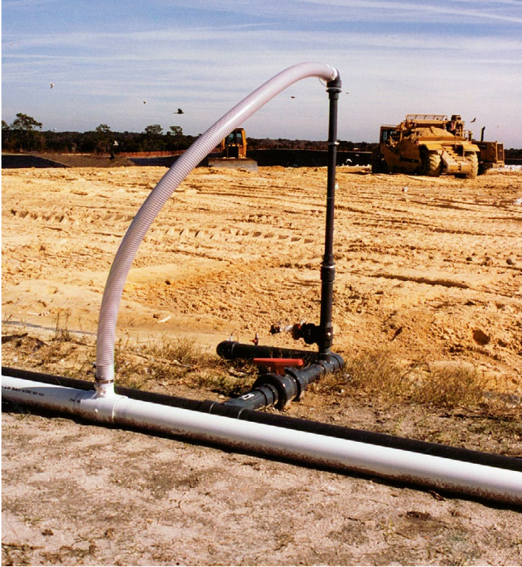
Fig. 4.6 Combined liquids addition and gas extraction system connected to horizontal trenches at ACSWL (white pipe is gas extraction manifold and gray pipe is liquids addition manifold)
