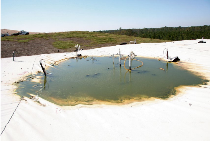
Fig. 8.19 Differential settlement around a cluster of vertical liquids addition wells that resulted in ponding of stormwater
