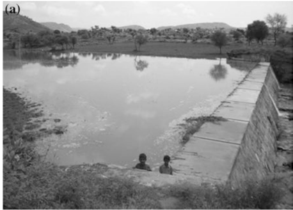
Fig. 4 a–c Example rainwater harvesting (RWH) structures present in the Arvari River watershed, a Bandh, b Johad, c Anicut
