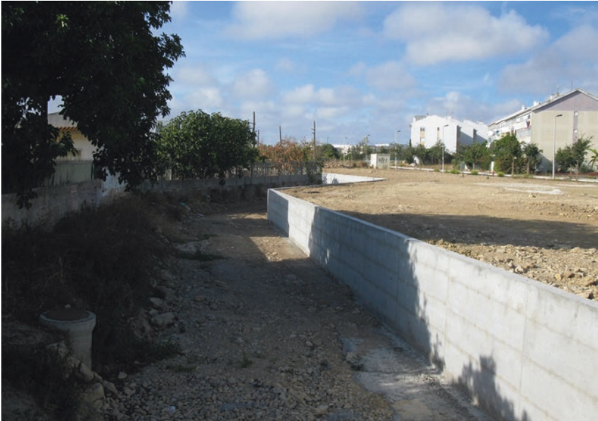
Fig. 6 Concrete walls canalizing the Sassoeiros stream. Such monumental structures neither protect the residential areas from flooding nor offer a habitat for the riparian fauna and flora. Photograph Smaniotto (2013)
