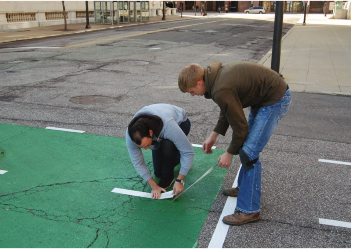
Kent State Urban Design Collaborative Students apply traffic tape as part of the Pop-Up Rockwell project. (Kent State Urban Design Collaborative)
