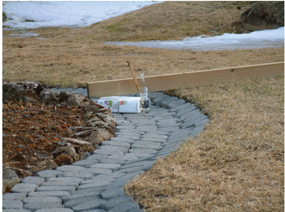
Fig. 10.3 Frost heaving. In summer, the grass surface is level with the stone-path, which has ‘frost free’ material under it. In winter, the grass lawn is heaved while the stone-path is not lifted except at the boundary to the grass. There is ample water in the soil under the grass in winter, enhancing the frost heave by water transfer to the freezing front
