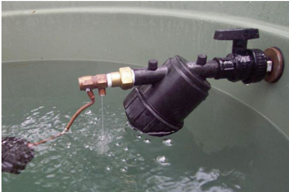
Fig. 23.8 Trickle feed system for a 500 L household water supply tank designed to limit demand by supplying a fixed daily volume of water to meet the assumed daily household demand. The system failed due to removal of the trickle feed by householders
