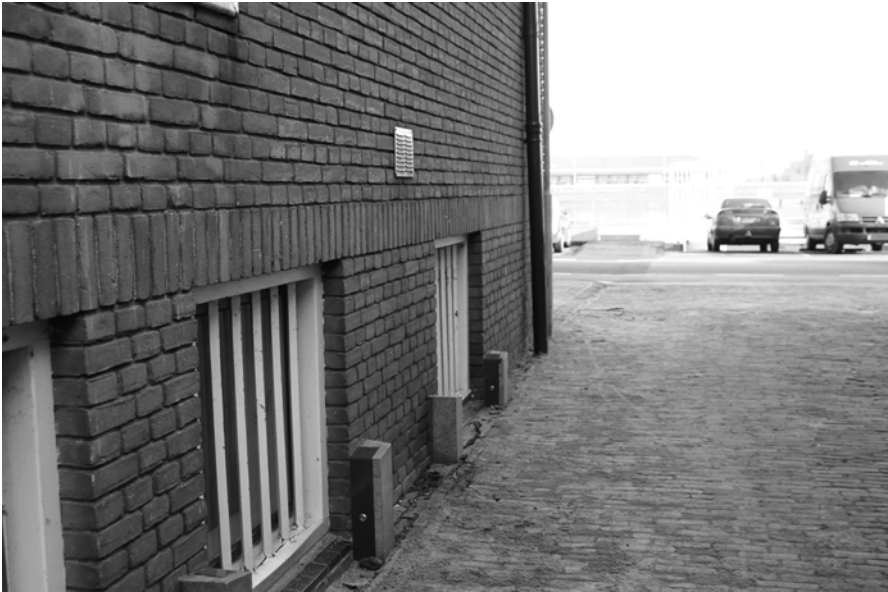
Fig. 25.5 Placeholders for demountable barriers in front of basement windows in the city of Kampen
