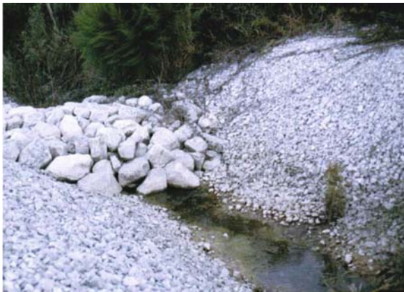
Fig. 7.16 A 1980 photograph showing a rock-constructed dam in the draining system leading away from the former Herbicide Orange Storage Site on the NCBC (Photograph courtesy of A.L. Young)
