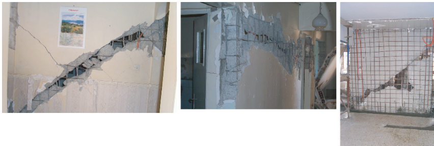
Fig. 3.4.3 Details of the structure. Crack on the longitudinal shear-wall at first floor (left), horizontal crack on the longitudinal shear-wall at first floor (center) and steel reinforcement of longitudinal shear-wall jacket (right)
