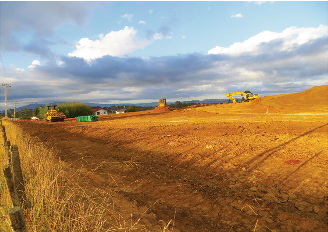
Fig. 8.25 Recontouring of land for urban housing development in New Zealand changes the topography and soil materials on a site. The recontoured site is designed to provide good foundations to support roads and buildings but often leaves the soil less suitable for supporting plant growth
