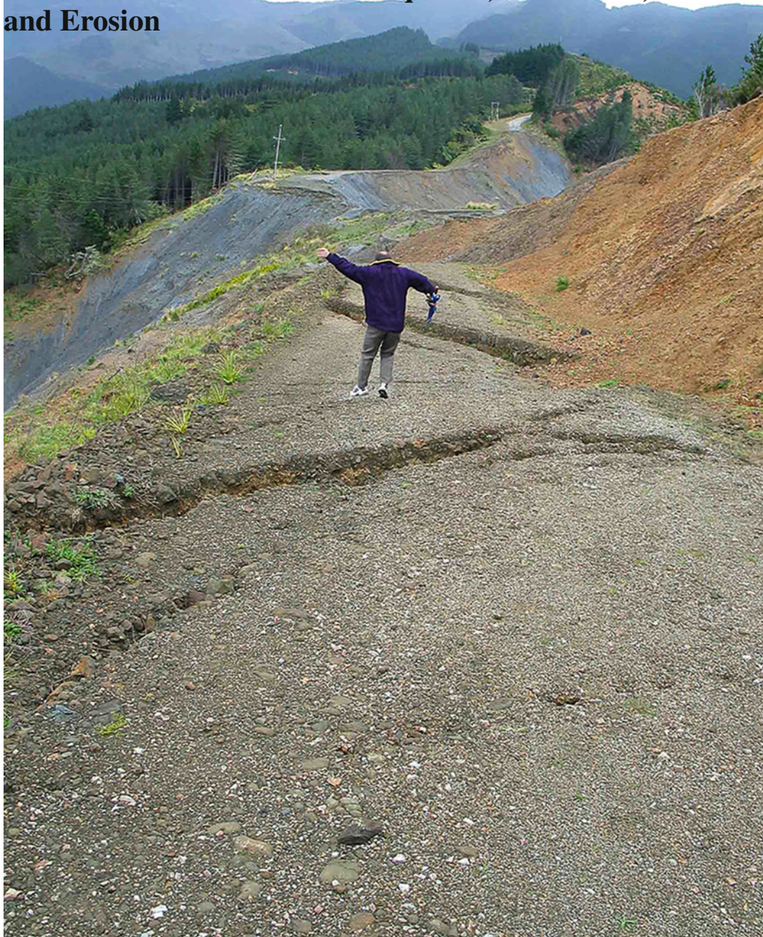
A person negotiates a road that has been repeatedly damaged by landslide activity
