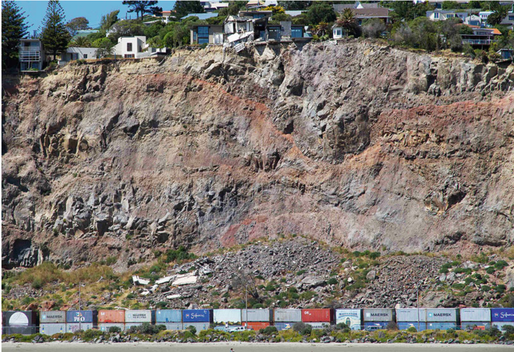
Fig. 7.11 A cliff face in Christchurch, New Zealand, from which large rocks were dislodged by earthquakes in 2011, leaving several houses teetering on the edge. Containers at the bottom protect the road from falling rocks dislodged by aftershocks
