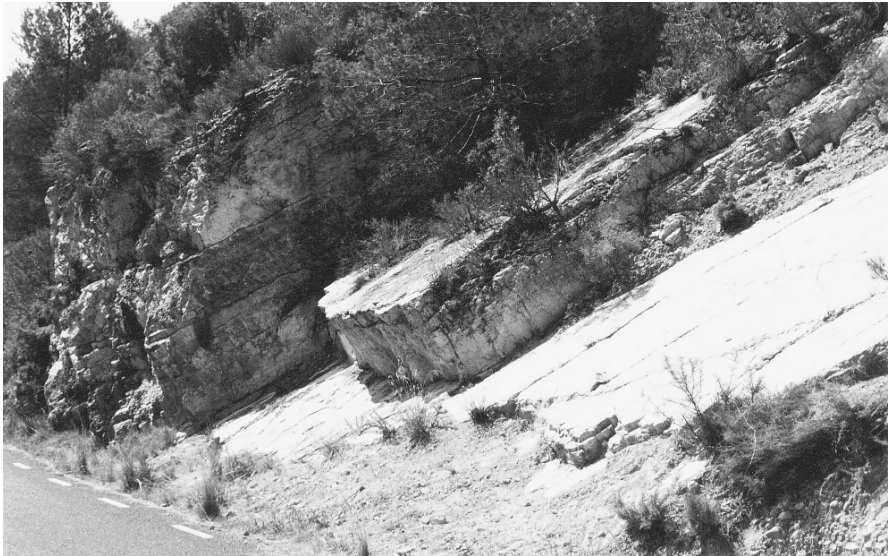
Fig. 3.1. Bedding planes as mechanical discontinuity planes causing failure of a slope in limestone
