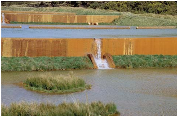
Fig. 91. Mine water overflowing the Pelenna II/Wales system. The hydraulic head is too low to drive the water through the compost (24 March 2000).
