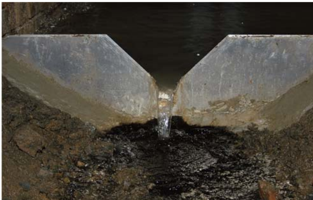
Fig. 55. A V-notch weir in the Felsendome Rabenstein/Germany underground visitor mine showing that the sharp-crested side has to be at the upstream side of the weir.
