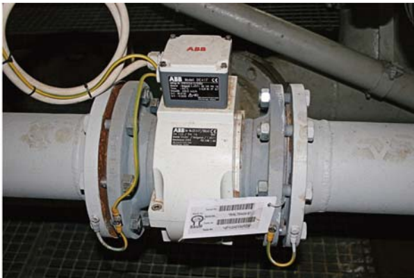
Fig. 60. Magnetic-inductive flow meter in the Schwarze Pumpe /Germany mine water treatment plant.
