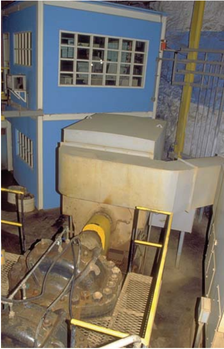
Fig. 28. Mine dewatering pump and mine water scheme control room in the Vazante/Brazil underground zinc-mine.
