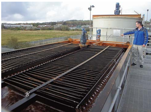
Fig. 87. Lamella clarifier at the Horden/United Kingdom HDS mine water treatment plant (photograph courtesy Andrea Berger).
