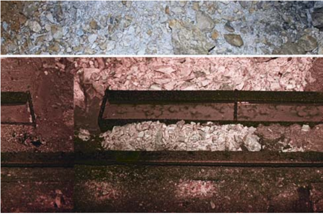
Fig. 50. Badly maintained channel for flow measurements in an underground mine. The channel inflow is not laminar and the channel itself is filled with sediment.
