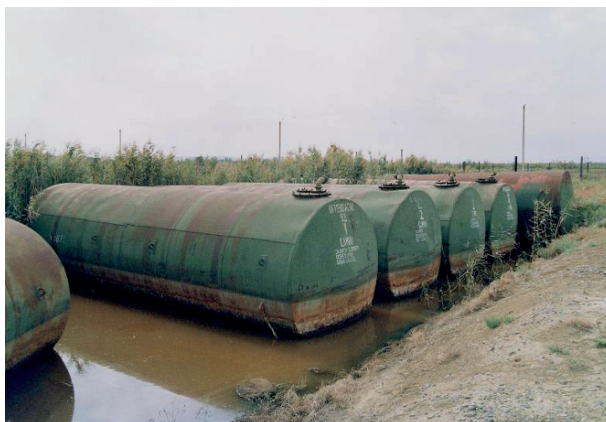
Figure 2. Tanks in contact with groundwater.
