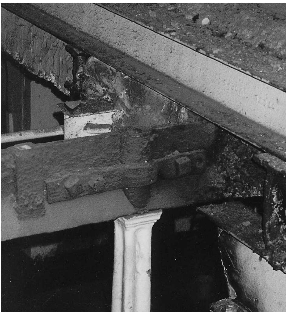
Figure 4.5 Inverted T-section cast-iron beams. As exposed in the 1797 Marshall, Benyon & Bage Flax Mill in Shrewsbury. Some beams are cracked where continuous over an intermediate column and a splice repair has been made using bolted wrought-iron straps. (Stuart Millns)
