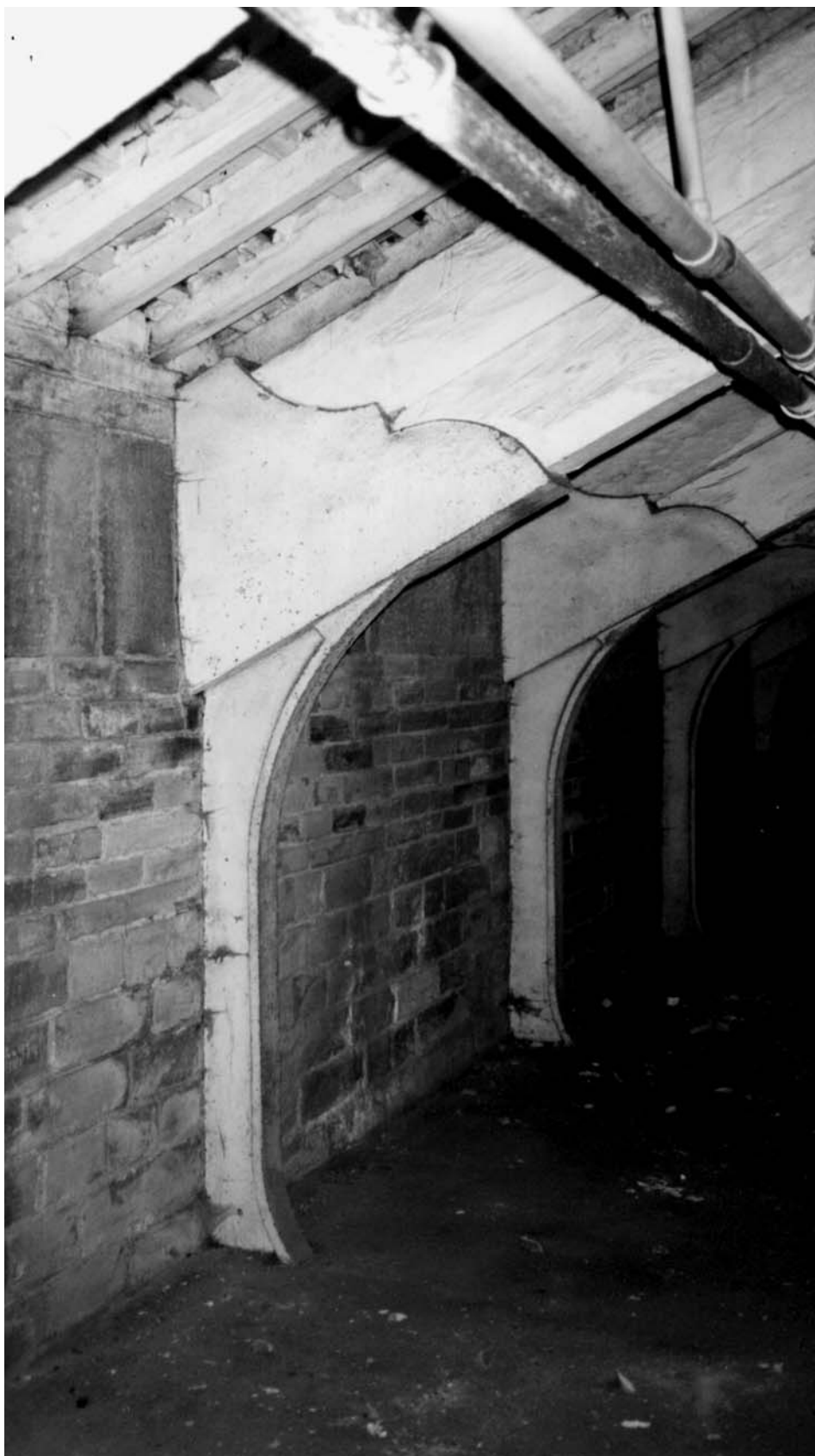
Figure 2.28 Timber roof with cast-iron knee braces. Garden Street Mill, Halifax (c. 1860). The brackets are fixed to the cast-iron floor beams and have a second leg within the wall. In this case there was no evidence of roof spread. (Stuart Millns)
