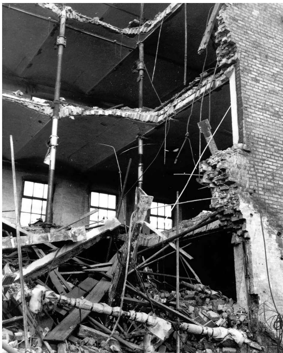
Figure 3.7 An iron-framed building during demolition in 1970. Fairbairn's block at Bean Ing Mill, Leeds (1823-4). (John Goodchild, reproduced with permission)
