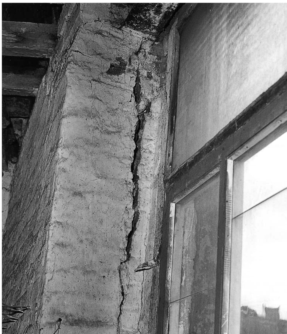
Figure 4.3 Separation of inner leaf brickwork from outer leaf stonework, due to the combined effects of low strength brickwork, poor bonding and settlement. (Stuart Millns)
