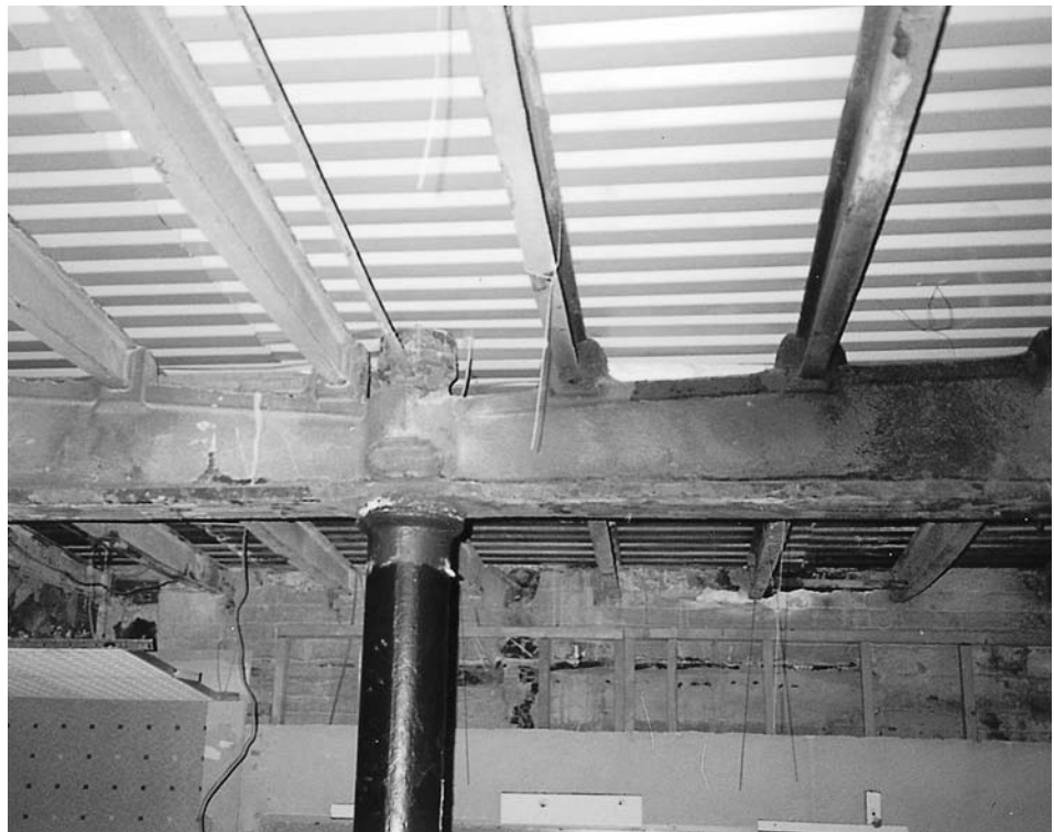
Figure 2.21 Bowling Mill, Dean Clough, Halifax (c. 1840). Hog-backed cast-iron beams and fish-bellied cast-iron joists which formerly supported stone slabs over the boiler house. (Stuart Millns)
