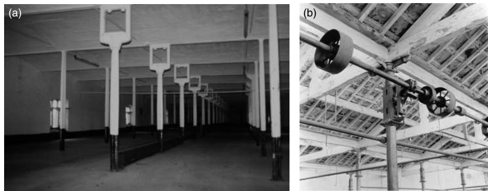
Figure 2.14 (a) Provisions for line shaft support – modified cruciform columns in the 1797 Marshall, Benyon & Bage Flax Mill, Shrewsbury. (b) Line shaft support brackets fixed to bolting faces on a hollow circular cast-iron column. James Walker blanket mill, Mirfield. (Ron Fitzgerald)
