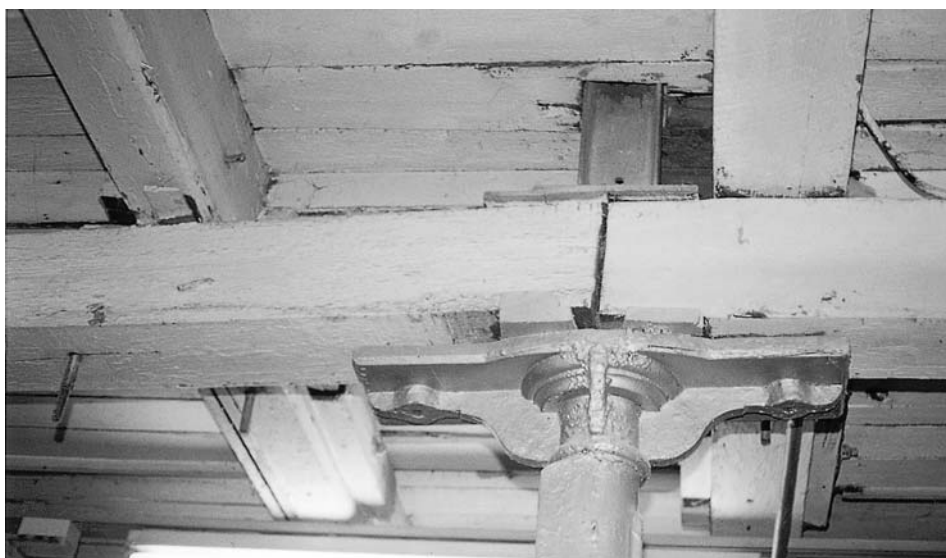
Figure 4.11 A structural alteration to a mid-nineteenth century warehouse and workshop showing gross lack of fixity. Note the absence of any bolts or coach screws and the very poor packing between the column end plates and the beam ends.
