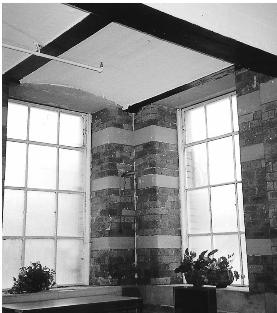
Figure 2.19 Manningham Mills, Bradford (1871). End bay showing change of direction to cast-iron beam and jack arch floor. Note the good quality of the through stones, lintels, cills and padstone into backing brickwork. (Stuart Millns)
