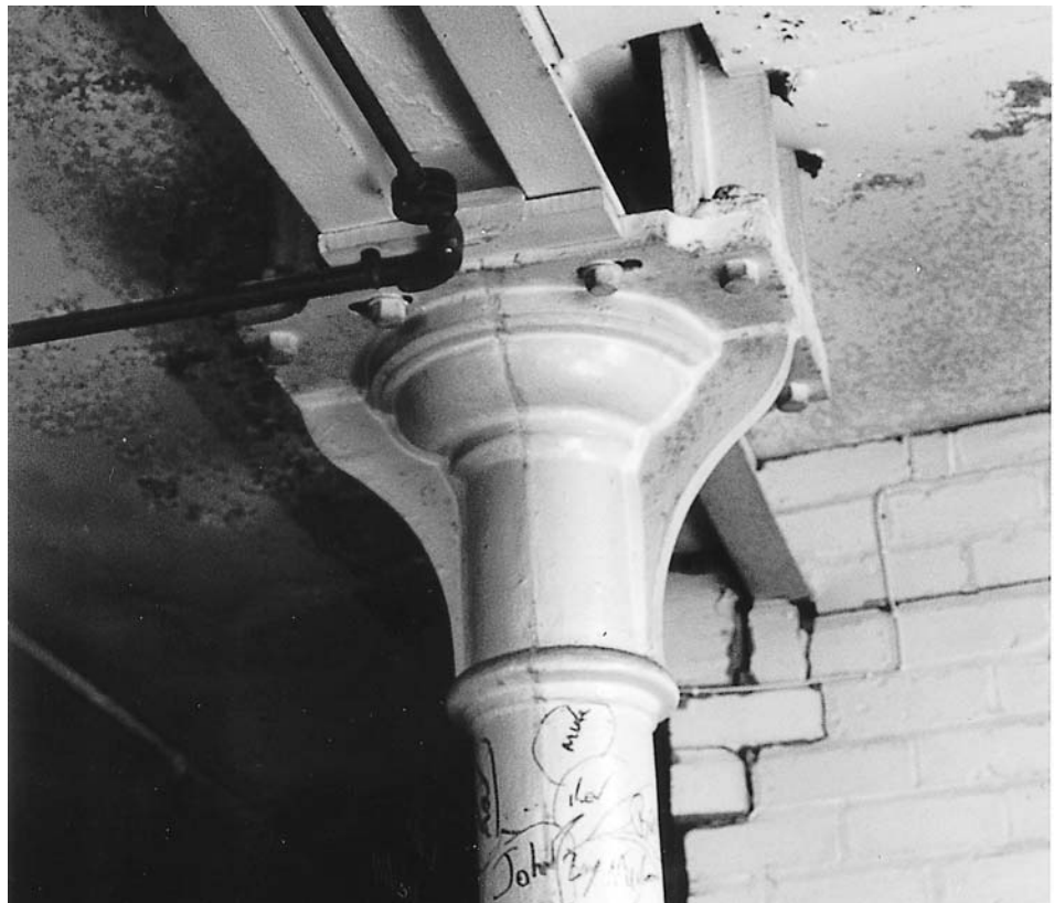
Figure 2.34 Floor supports in Murray's New Mill, Manchester. Built in c. 1804, with two lines of cruciform columns to continuous timber beams, the building was modified c. 1900. The original columns were replaced with a single line of hollow circular cast-iron columns and the floors supported by channels placed either side of the original timber beams.
