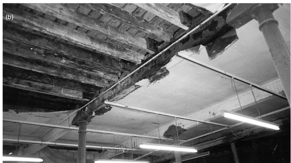
Figure 2.16 (a) Wrought-iron tongues between thick floorboards (e.g. Havelock Silk Mill, Manchester, c. 1830). (b) Wrought iron sheet fire protection to a timber beam and joist floor in the 1855 Canal Mill, Botany Bay, Chorley.
