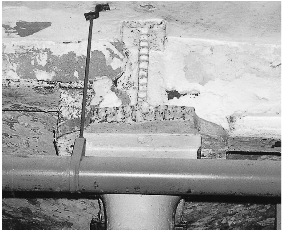
Figure 4.12 Replacement floor details. An arch floor removed and cast iron beam cut away at Manningham Mills, Bradford, and replaced with a reinforced concrete slab. Note the unsymmetrical cross-section of the beam and the means of cutting by a series of drilled holes. (Stuart Millns)
