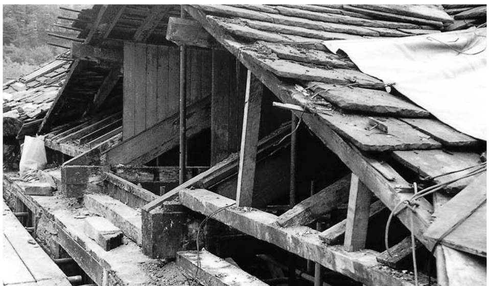
Figure 4.13 Remedial work to timber roof in progress. The roof to Greenup's Worsted Mill, c1791, Sowerby Bridge Mills. Lack of maintenance to gutters and eaves masonry often leads to rapid deterioration of mortar, requiring rebuilding of masonry, replacement of timber wall plates and remedial work to timber truss bearings. (Stuart Millns)
