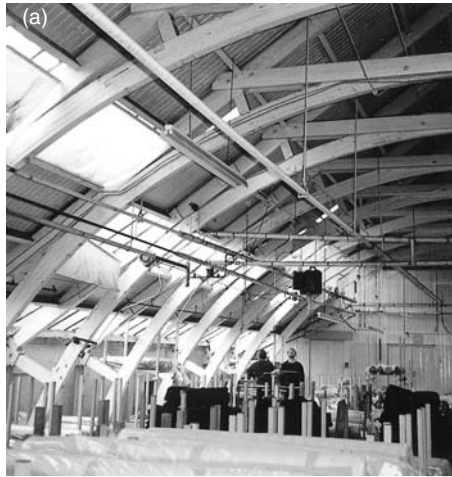
Figure 2.30 (a) Laminated timber roof arches with cast-iron wall brackets. Lumb Lane Mills, Bradford (1856). Up to six timber planks were screwed together with through-bolted truss connections (Stuart Millns). (b) Similar timber arches and floors seen during demolition of a mill. (Ron Fitzgerald)
