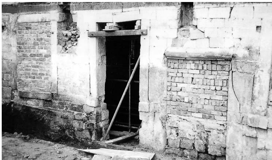
Figure 4.2 Poorly carried out structural alterations to a wall. Bricking up of openings prevented early collapse of this 1830s mill with cast-iron columns and timber floors. Complete rebuilding of the wall was required. (Stuart Millns)
