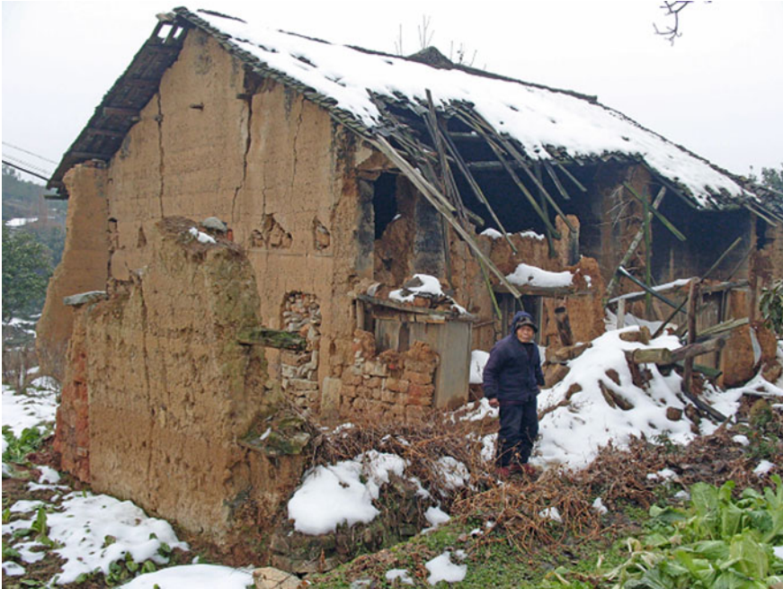
Fig. 7.1 In Liaojialin Village, Xiaoxita Town, Yiling District, Yichang, Hubei, farmer Zhengfu Huang's house collapsed due to the snow disaster. (Junfeng Liu/Imaginechina)
