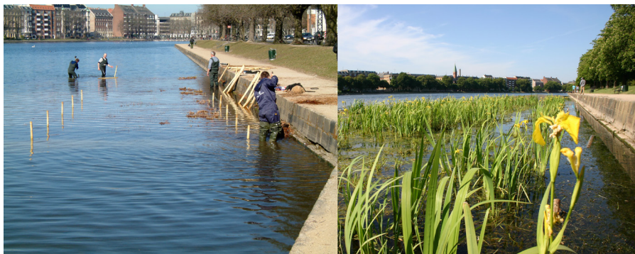
FIGURE 10.4 Introduced vegetated areas in Northern basin of Lake Sortedam, Copenhagen, Denmark during construction in March/April 2005 (left) and a year after establishment (July 2006). (Photos by Søren Berg and Christian Skov)
