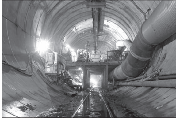
Figure 5. Elevated deck for construction of the adit from the Main Spine Tunnel
