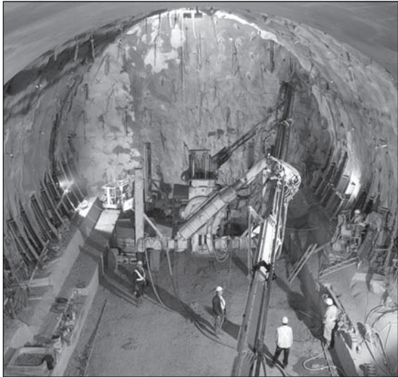
Figure 30. Tartaguille tunnel: Installation of fiberglass elements in the core. Notice the kickers and the final invert against the face. After Lunardi (2008).
