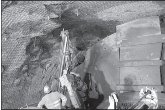
Figure 20. Excavation support in L1 of the TBE (with spalling above the cutterhead)
