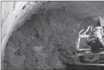
Figure 15. Extruding mud in the Power Tunnel crown
