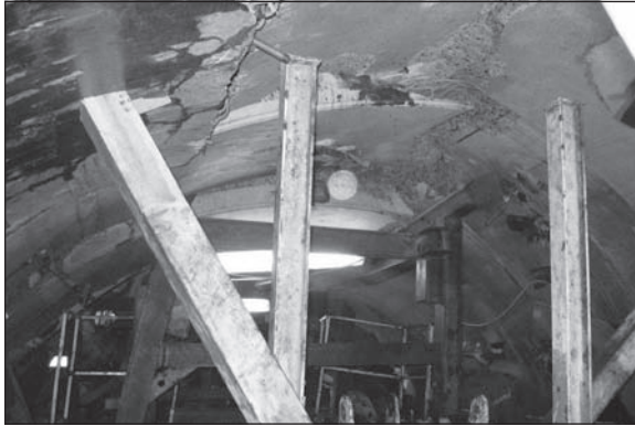
Figure 4. Lining segments moved and severely damaged
