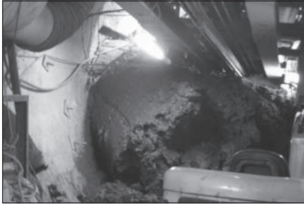
Figure 13. Extruding mud in the Power Tunnel
