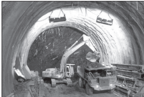
Figure 20. Raticosa tunnel for the Bologna-Florence high-speed railway: Full face excavation under 500 m of cover in highly squeezing scaly clays. After Lunardi (2008).
