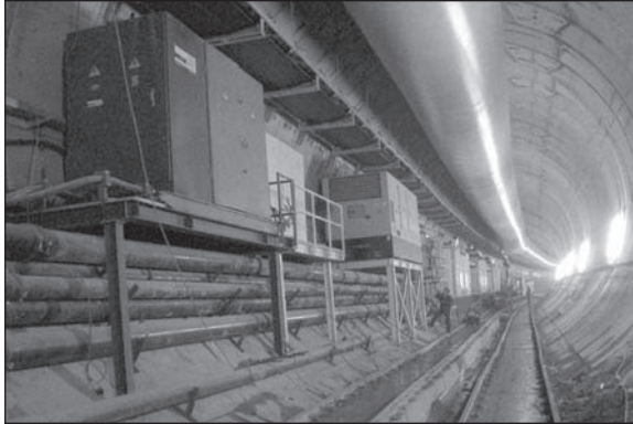
Figure 17. Intermediate dewatering pump station comprising: 3 water tanks, 1,000 kVA transformer, 1,000 kVA in generator sets and water pumps
