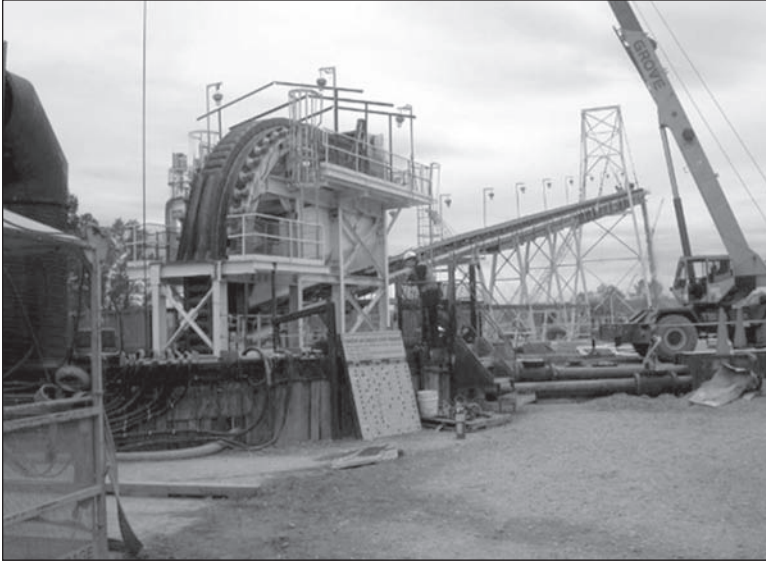
Figure 1. Vertical muck conveyor
