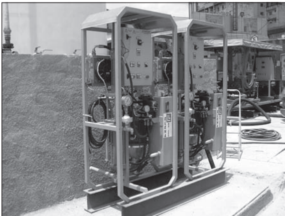
Figure 17. Component B—sodium silicate—pumping station
