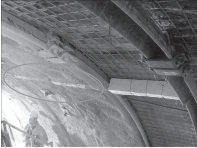
Figure 17. Injected convergence slots in the L1 area
