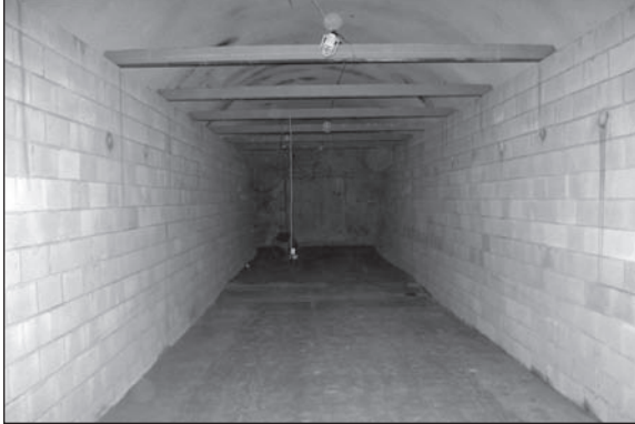
Figure 12. Tryon Street seepage area
