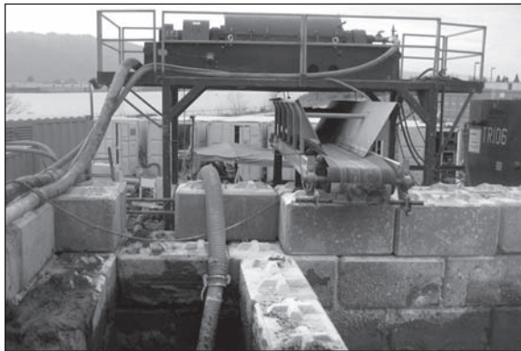
Figure 5. Centrifuge with discharge conveyor
