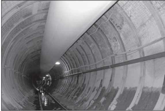
Figure 13. Steel set support at Fault F7
