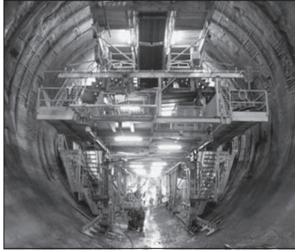
Figure 16. TBE back-up equipment
