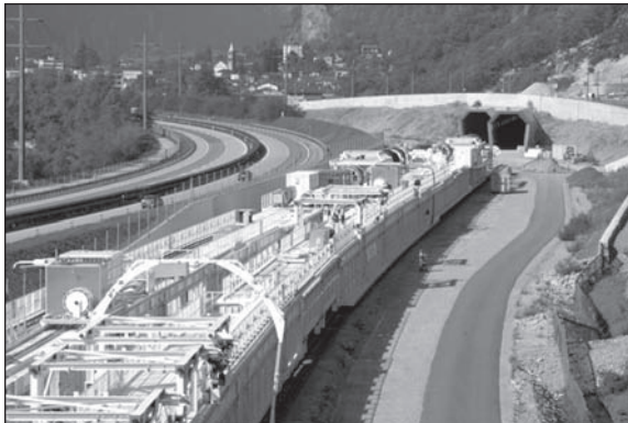
Figure 16. Portal Bodio, inner lining equipment before moving through the opencast constructed tunnel
