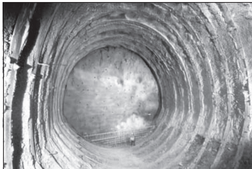
Figure 21. Raticosa tunnel for the Bologna-Florence high-speed railway: Preparing for pouring the final invert under 500 m of cover in highly squeezing scaly clays. After Lunardi (2008).
