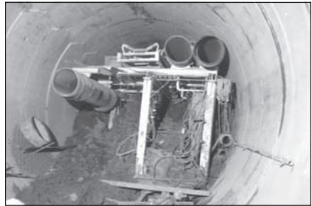
Figure 16. Consolidated mud filling the Power Tunnel
