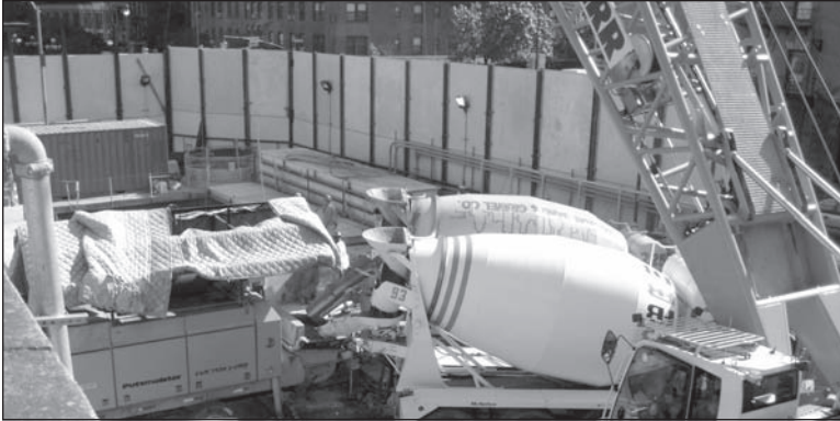
Figure 7. Shaft 33B (adjacent to Queensboro Bridge at the corner of East 59th St. and 1st Ave.) looking east at concrete pump while shaft is also being constructed
