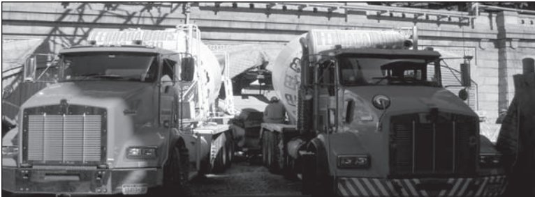
Figure 8. Shaft 33B (adjacent to Queensboro Bridge at the corner of East 59th St. and 1st Ave.) looking north at concrete pump while shaft is also being constructed
