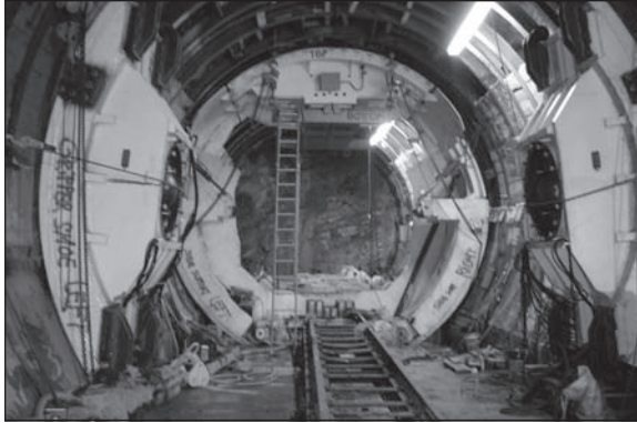
Figure 6. View shows Robbins Assembly Chamber with front shield built and gripper shoe hung waiting on TBM to arrive. TBM will drive through front shield.
