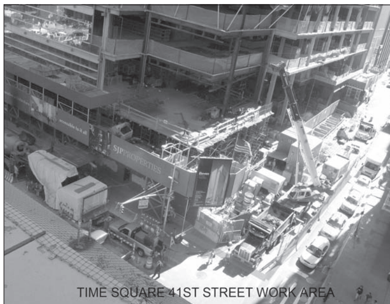
Figure 4. Top of material access shaft and muck removal compound at West 41st Street and 8th Avenue
