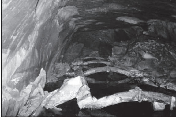
Figure 3. Photo of collapsed tunnel
