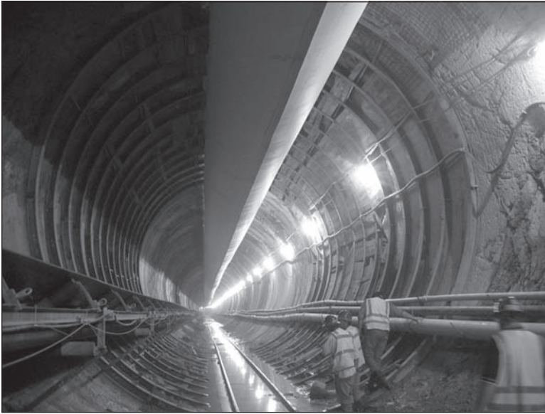
Figure 2. Atlanta West CSO tunnel steel rib supports
