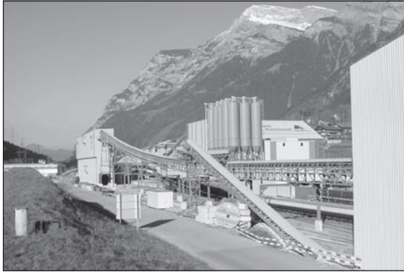
Figure 20. Construction site at Amsteg, encapsulated plants and conveyors belt systems reduce noise
