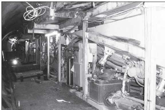
Figure 5. Obstructions (trailing gear) block 30 to 40% of the cross-section in small size TBM tunnel B (diameter 2.8 m, cross-section 6.15 m 2 )
