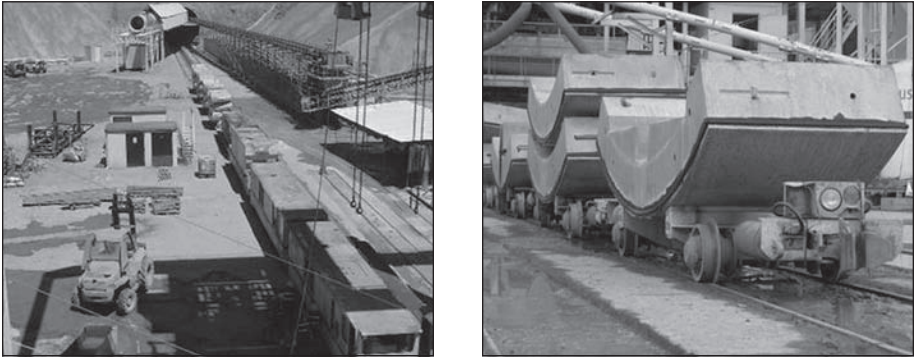
Figure 19. Train at the portal (left) and precast concrete segments in cars (right)
