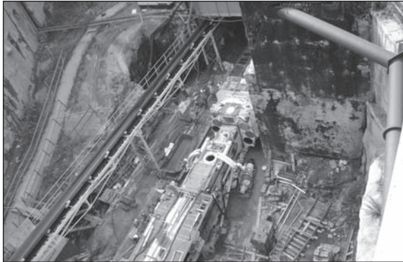
Figure 7. View showing the building of the Robbins TBM at the Queens shaft included
