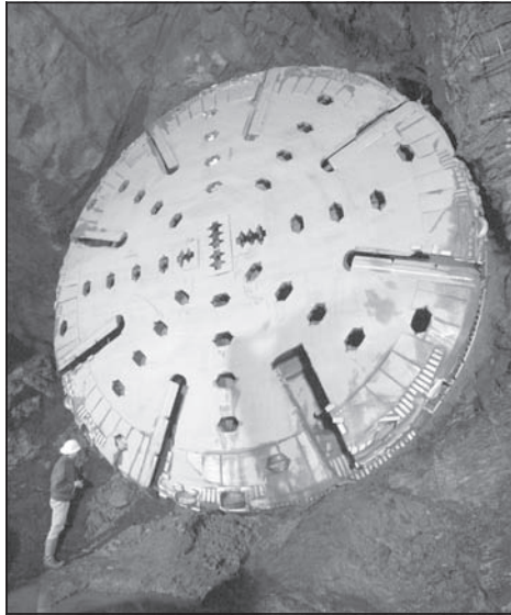
Figure 3. TBM cutterhead following hole-through at the Foundry shaft (photo by Sue Bednarz)
