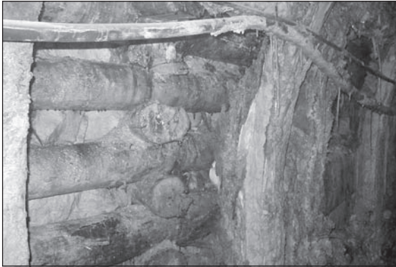
Figure 5. Steel sets before rehabilitation
