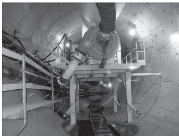
Figure 9. Booster pump station in the tunnel
