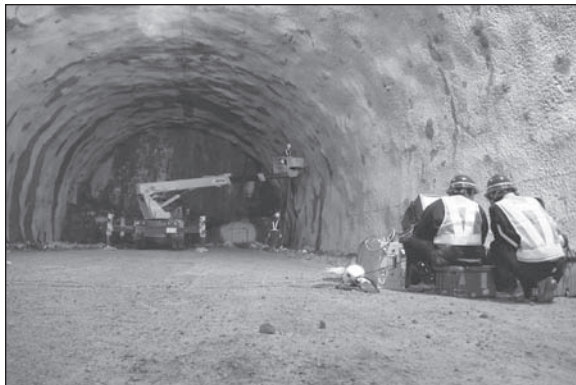
Figure 4. No significant obstructions for radio communications in large cross-section NATM tunnel A (cross-section 80 m 2 )
