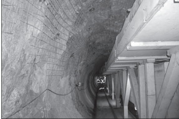
Figure 6. Overstressing and fall out
