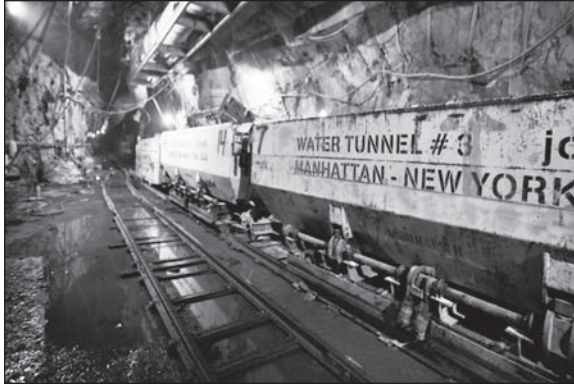
Figure 1. Starter tunnel (dill and blast) area at bottom of shaft 26B looking south
