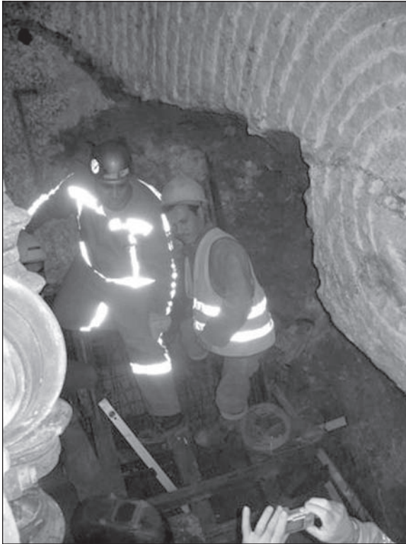
Figure 9. Large karstic cavity in a fracture zone at Chainage 1+578 m. The cavity was filled with clay and breccia boulders of various sizes, which caused a major recovery problem and delay to TBM excavation.
