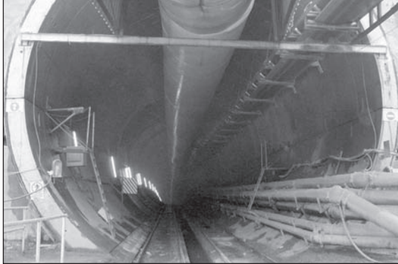
Figure 16. Tunnel portal with the main service lines and services: ventilation, conveyor belt, electrical power, light, water in and dewatering lines
