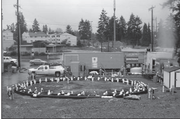
Figure 3. Installed and operating ground freezing system
