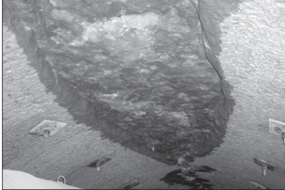
Figure 5. Example of slabbing after scaling was performed
