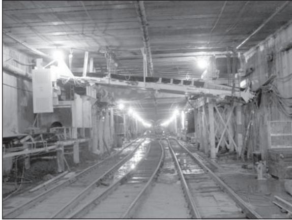
Figure 4. View shows York Avenue existing tunnel. We have 2 belt storage units for EB and WB TBM tunnels and transfer conveyor to feed fixed tunnel conveyor.
