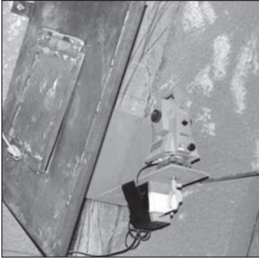
Figure 8. Motor laser in side-wall gallery with blasting protection
