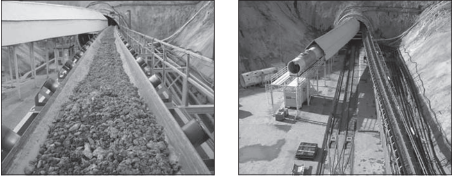
Figure 20. Main conveyor belt with its band extensor at the portal
