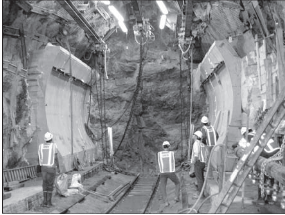
Figure 5. View showing started tunnel for SEL1 with gripper wall, poured invert and monorail hoist for assembly
