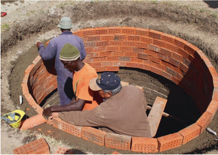
Fig. 4.7 Use bricks as mold for casting the concrete wall of water cellar
