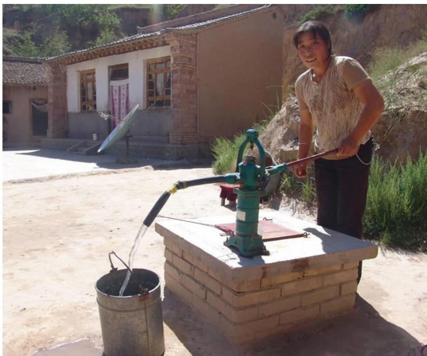
Fig. 1.6 A typical household 1-2-1 Rainwater Catchment Project
