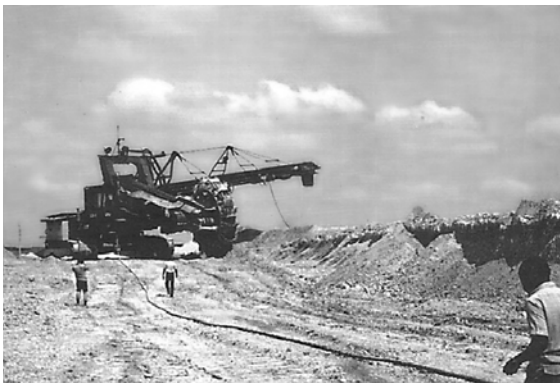
Fig. 373 Excavation of overburden and phosphate ore of Eocene age by bucket-wheel excavators at Hahotoe-Akoumape in southern Togo
