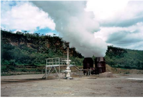
Fig. 176 A geothermal energy producing field at Olkaria near Lake Naivasha
