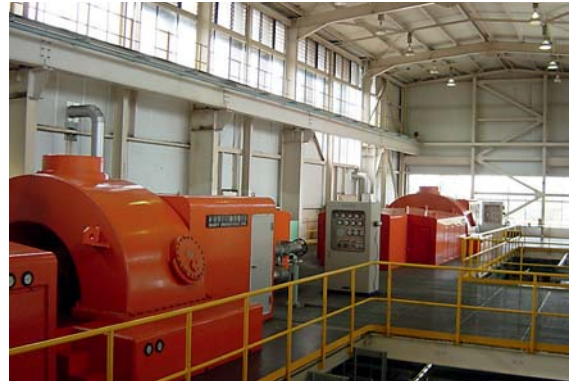
Fig. 178 Turbine house at Olkaria geothermal power plant
