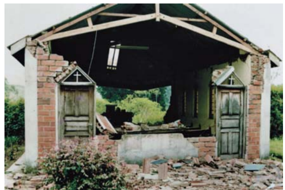
Fig. 396 A church hit by the Fort Portal earthquake of 5 February 1994 in western Uganda
