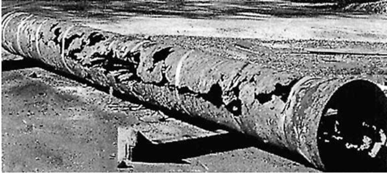
Fig. 2 Heavily corroded underground steel pipe (Courtesy of Utah State University Buried Structures Laboratory)
