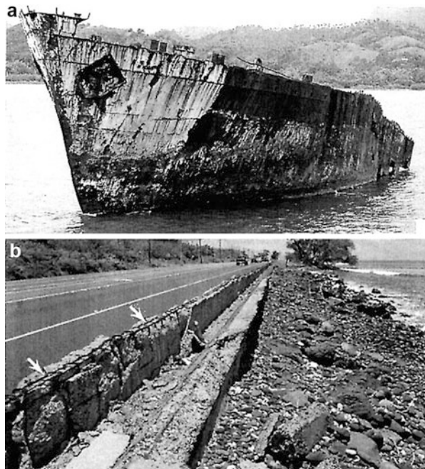
Fig. 3 Salt-aerosol-related steel structure corrosion. (a) Steel ship hull. (b) Steel rebar – reinforced concrete structure showing rebar corrosion and concrete spallation due to corrosion product expansion. (Courtesy Concrete Construction. Net). Arrows show exposed, corroded rebar
