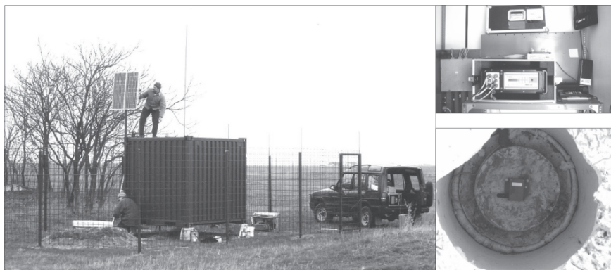
Figure 3 The SP field stations each consist of a three component short period seismometer located in a pit, with a digital recorder and time signal receiver housed nearby in a heat insulated steel container building
