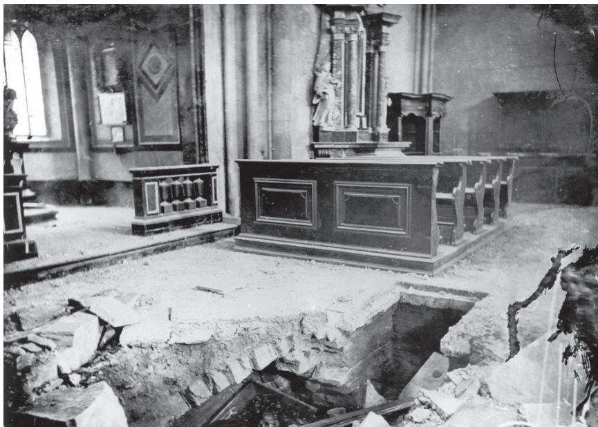
Figure 4 Damages of St. Stephen's Cathedral situated in the center of Zagreb after the great Zagreb earthquake in 1880
