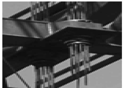
Figure 4. The spreaders arranged on the down chord.
