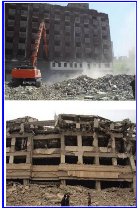
Figure 1. A large number of abandoned concrete demolition and earthquake disaster.
