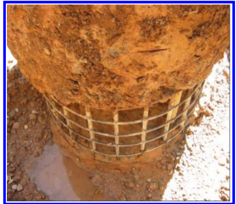
Figure 5. Mud-clamping of defective position.
