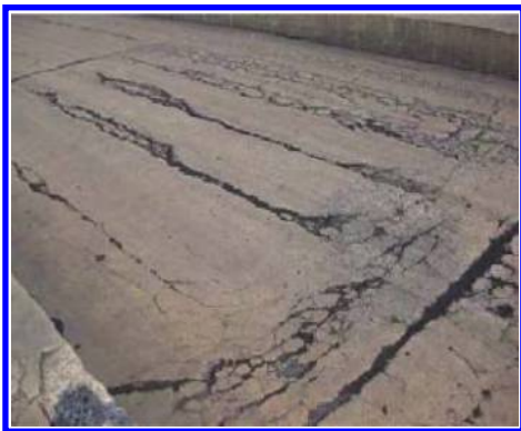
Figure 1. Hollow hinge joint of one bridge in China.
