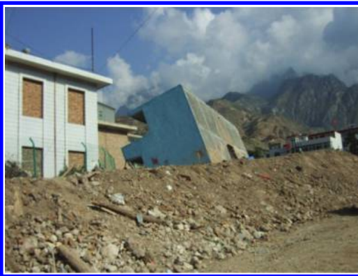
Figure 2. Global overturning of masonry structure.
