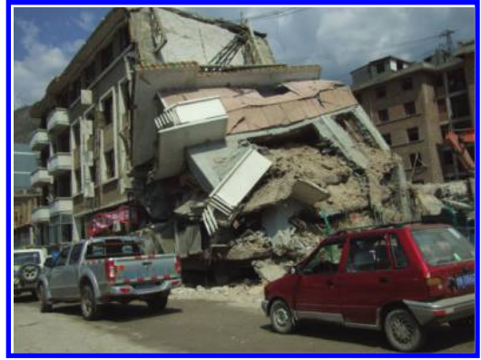
Figure 3. Partial collapse of masonry structure.
