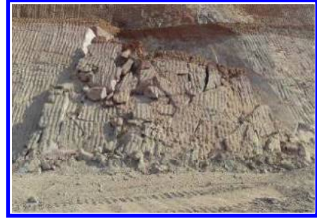
Figure 7. Failure slope on site.
