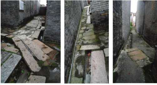
From left to right: The tilted stone relate to the path of the people. The drainage is in the centre of the road. The direction of stone imply the entrance of building.
