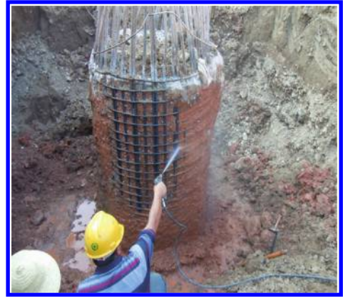
Figure 3. Leakage tendon of the defective position.
