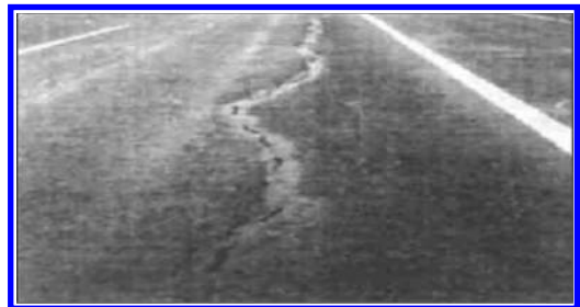
Figure 1. Pavement settlement and crack.
