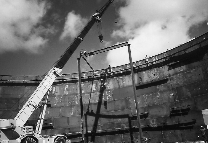
Figure 4-4. Workers Not Wearing Safety Harnesses at Oil-Tank Reconstruction in St. Croix
