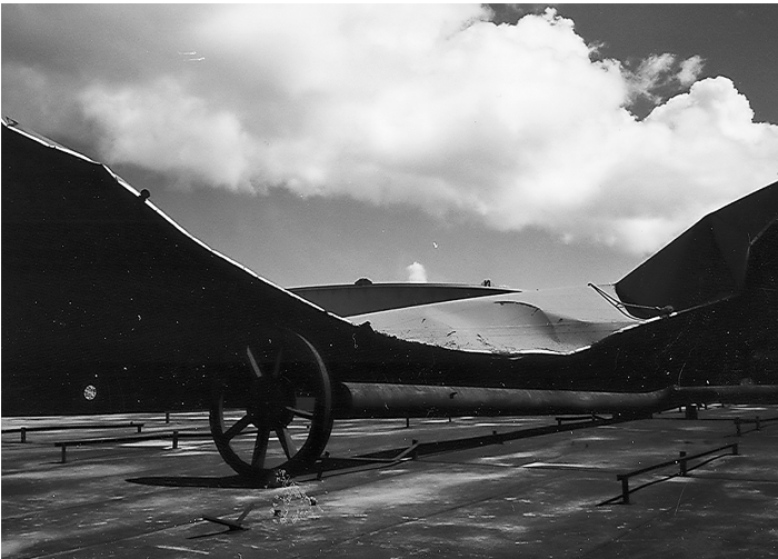
Figure 4-7. Oil-Tank Destruction by Hurricane in St. Croix
