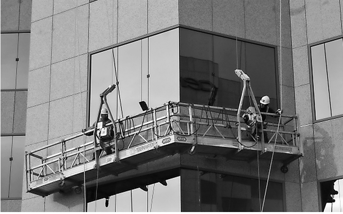
Figure A-14. Type 1 Platform with Platform Extension for Type B Edge Bays
