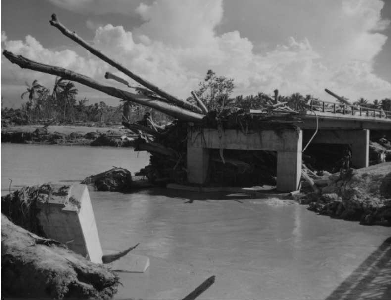
FIG. 10.13. Bridge over the Ngalimbiu River on Guadalcanal island in Solomon Islands, wrecked by floodwaters and sediments during Tropical Cyclone Namu on 18–19 May 1986. Photo courtesy of the Department of Mines and Energy, Solomon Islands.
