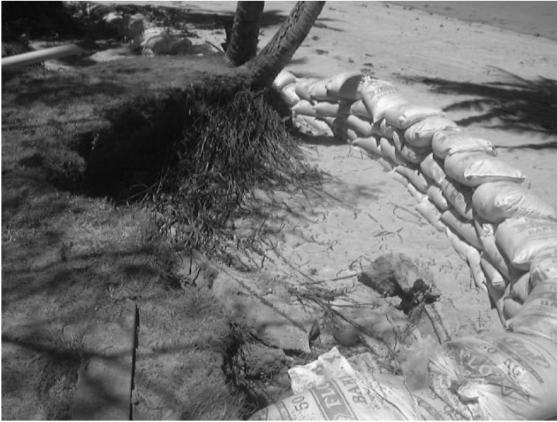
FIG. 7.3. Sandbags installed as a (belated) temporary-protection measure for beachside coconut palms at the Shangri-La Fijian Resort in southern Fiji. The beach was eroded several days earlier during Tropical Cyclone Paula on 4 March 2001.
