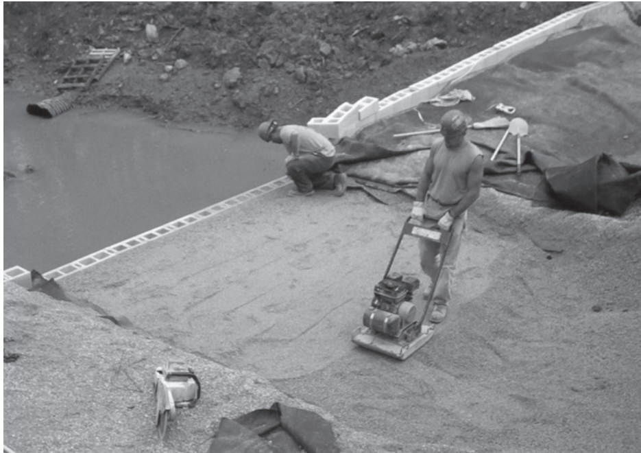
Figure 13.34 Construction of a retaining wall with geotextile reinforcement (Courtesy of Jonathan T. H. Wu, University of Colorado at Denver, Denver, Colorado)
