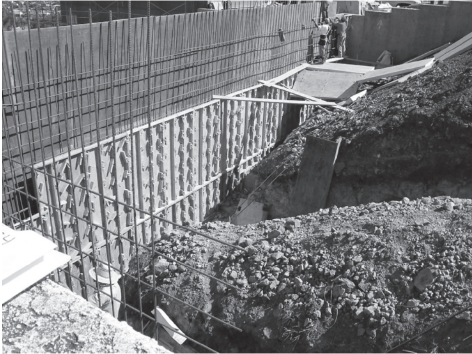
Figure 13.31 A cantilever retaining wall under construction (Courtesy of Dharma Shakya, Geotechnical Solutions, Inc., Irvine, California)
