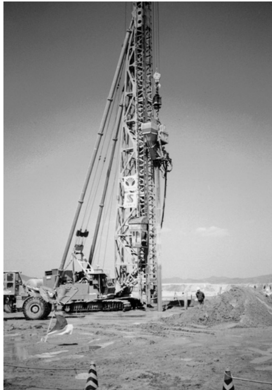
Figure 11.39 Sand drain installation in progress (Courtesy of E.C. Shin, University of Incheon, South Korea)
