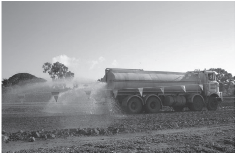
Figure 6.19 Spraying of water on each lift of soil before compaction in the field (Courtesy of N. Sivakugan, James Cook University, Australia)
