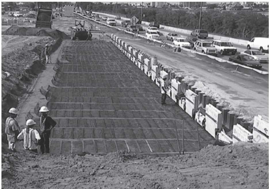
Figure 13.35 HDPE geogrid-reinforced wall with precast concrete panel facing under construction (Courtesy of Tensar International Corporation, Atlanta, Georgia)
