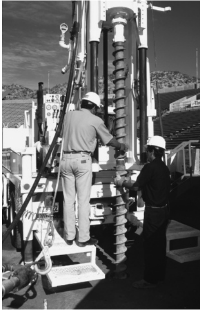
Figure 17.2 Drilling with flight augers (Courtesy of Danny R. Anderson, PE, of Professional Service Industries, Inc., El Paso, Texas)
