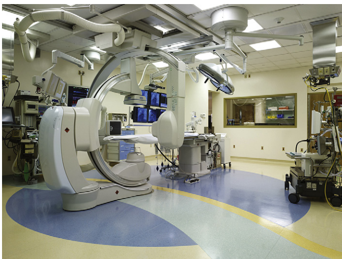
FIGURE 24-22 View of hybrid cardiovascular operating room. The cardiopulmonary bypass circuit is on the far right with its own boom. The operating table is in the middle of the picture, with a floor-mounted, fixed biplanar C-arm to the left. (From Kaplan JA, Reich DL, Savino JS. Kaplan's Cardiac Anesthesia: The Echo Era . 6th ed. Philadelphia: Saunders; 2011.)
