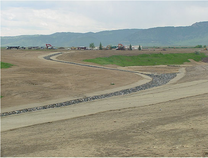
Fig. 9 The reconfigured Walnut Creek basin functional channel shows the heavily armored channel and extensive erosion-control measures on stream banks. The measures included straw bales, wattles, and crimping; silt fences; mats; hydromulch and Felxterra TM , and rip-rap (rock) lining of drainage channels
