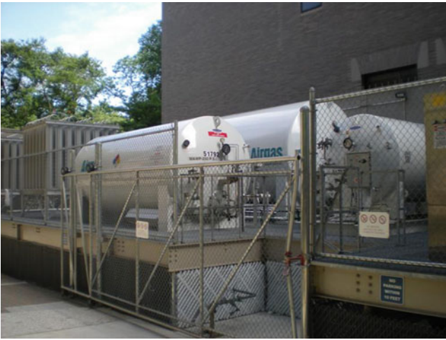
Fig. 6.1 Bulk liquid oxygen storage vessels
