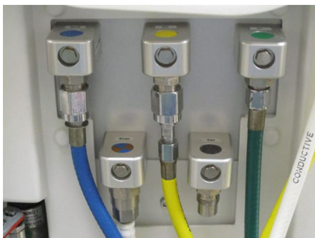
Fig. 6.7 Diameter-indexed safety system (DISS) gas connectors in back of anesthesia workstation. Green =oxygen; yellow =air; blue =nitrous oxide; white =vacuum
