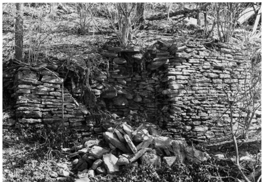
Fig. 3.3. Broken old stone wall on colluvium-covered hillside shows long-term influence of creep, Walker Street, Cincinnati, Ohio
