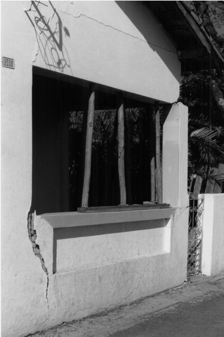
Fig. 9.18. Settling of a house wall on collapsible, tropical oxisoil in Rio Claro, Sao Paulo, Brazil. Note cracks in wall and wooden supports in windows
