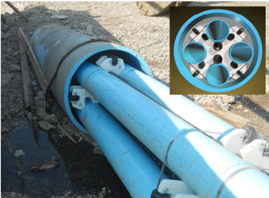
Figure 2. Final conduit bundle assembly, showing the (4) 8-inch FPVCP conduits, the (4) potential 2-inch HDPE conduits (only two used), the (2) 3-inch HDPE grout tubes, as well as the casing spacers and how the configuration was banded together.
