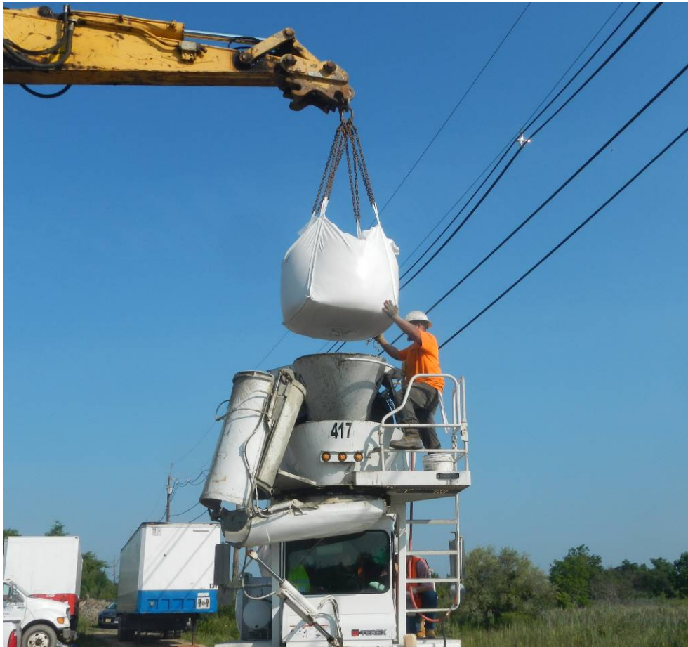
Figure 6. Addition of sand on-site as part of the hybrid grout batching arrangement for the project.
