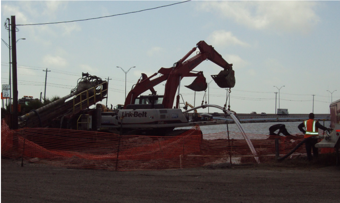
Figure 5. Insertion of the 200 mm (8-inch) Steel gas line into the Laguna Madre HDD section.
