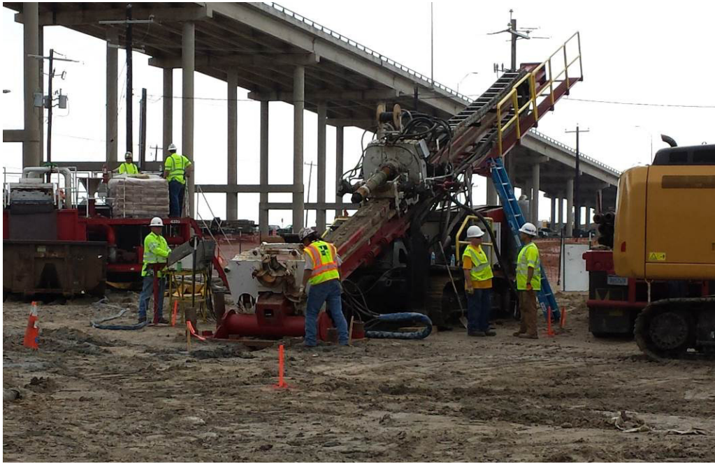
Figure 3. Drill rig set up for the first bore of the GIWW crossing.
