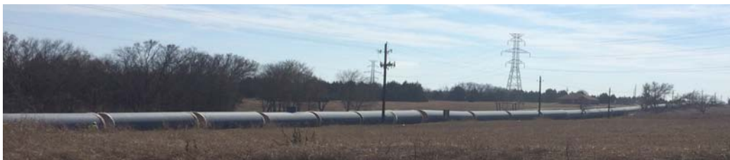
Figure 4. Southwest Pipeline Material Storage
