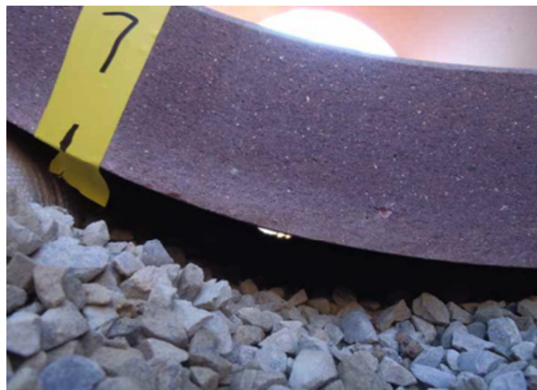
Figure 7: In testing, daylight was visible on the other end of a 7.0' pipe section.
