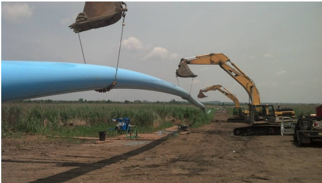
Figure 4. Typical 30-inch FPVCP casing insertion shown with aerial support provided to guide the FPVCP into the required angle of the drill exit.
