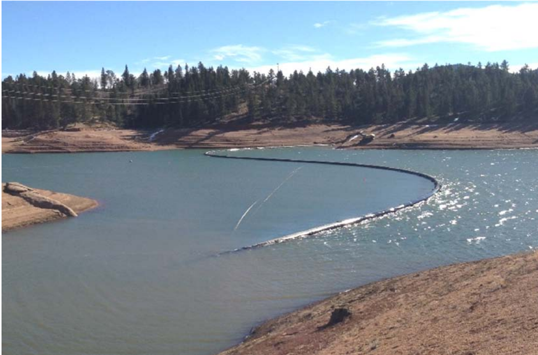
Figure 8 - HDPE Transfer Pipe at the start of the sinking process, floating on the reservoir surface over its eventual alignment
