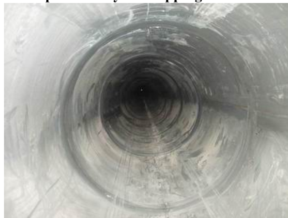
Figure 5. Stainless steel liners after insertion into the host pipe (from BAODING JINDI SCIENCE&TECHNOLOGY DEVELOPMENT CO., LTD)
