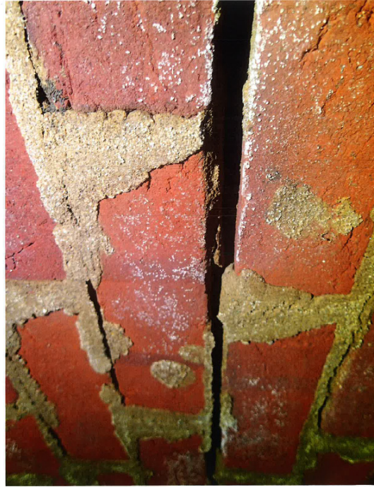
Figure: 13 - Crack at crown (+/-12 O Clock position)
