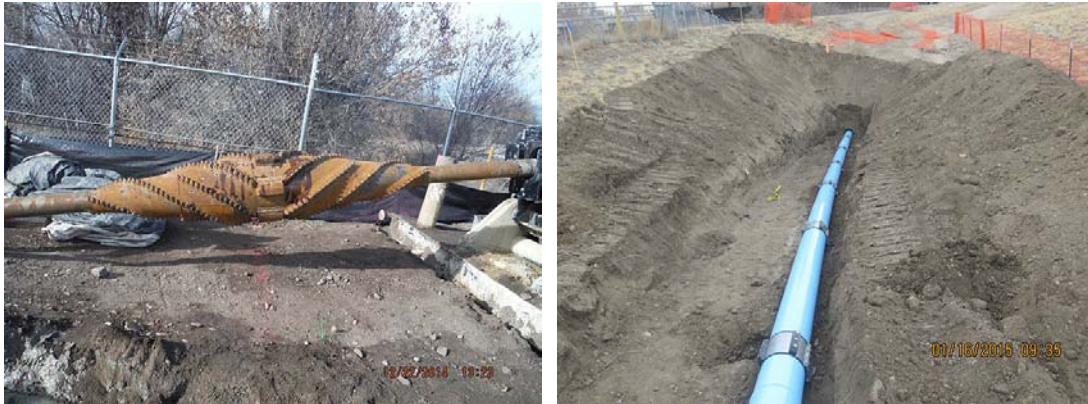
Figure 5. 24-inch Fluted Reamer (Left) / 10-inch Fusible PVC with Casing Spacers Pushed into the 16-inch Steel Casing Installed via HDD (Right).
