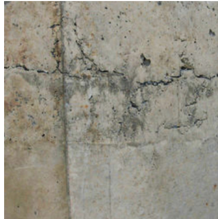
Figure 3: Typical Cement Cold Joint
