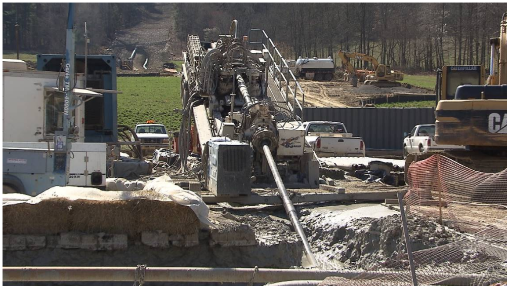
Figure 3. The largest directional drill rig used for the project, an American Augers DD1100.
