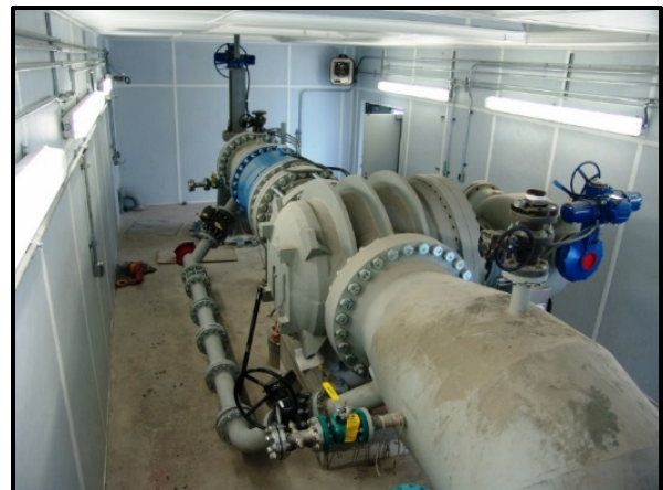
FIGURE 3. Hobbble Creek Station valve room. The sleeve valve is below floor at the back of the photo.
