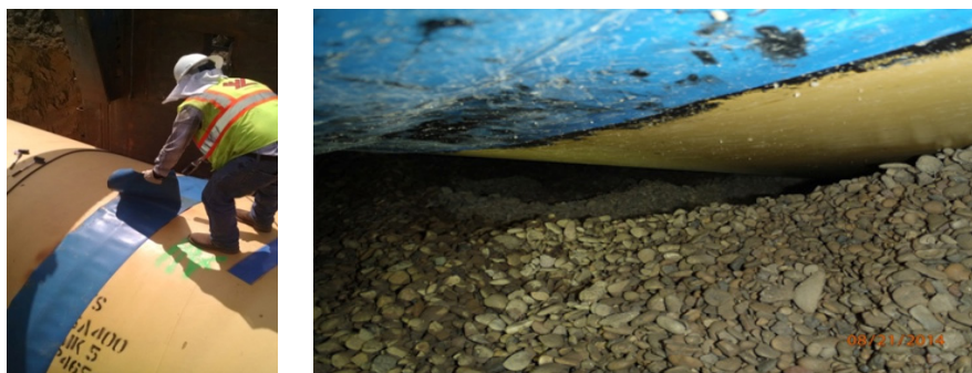
Figure 14a, b: Application of Heat Shrink Sleeve, Voids in Bell Holes after Completion of Backfilling
