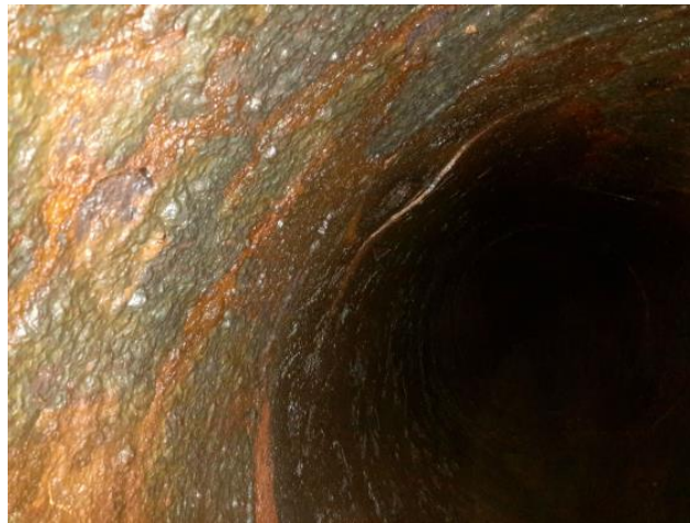
Photo 2. Exposed Steel Cylinder at Joint
