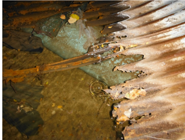
Figure 3. CMP invert deterioration with water piping.
