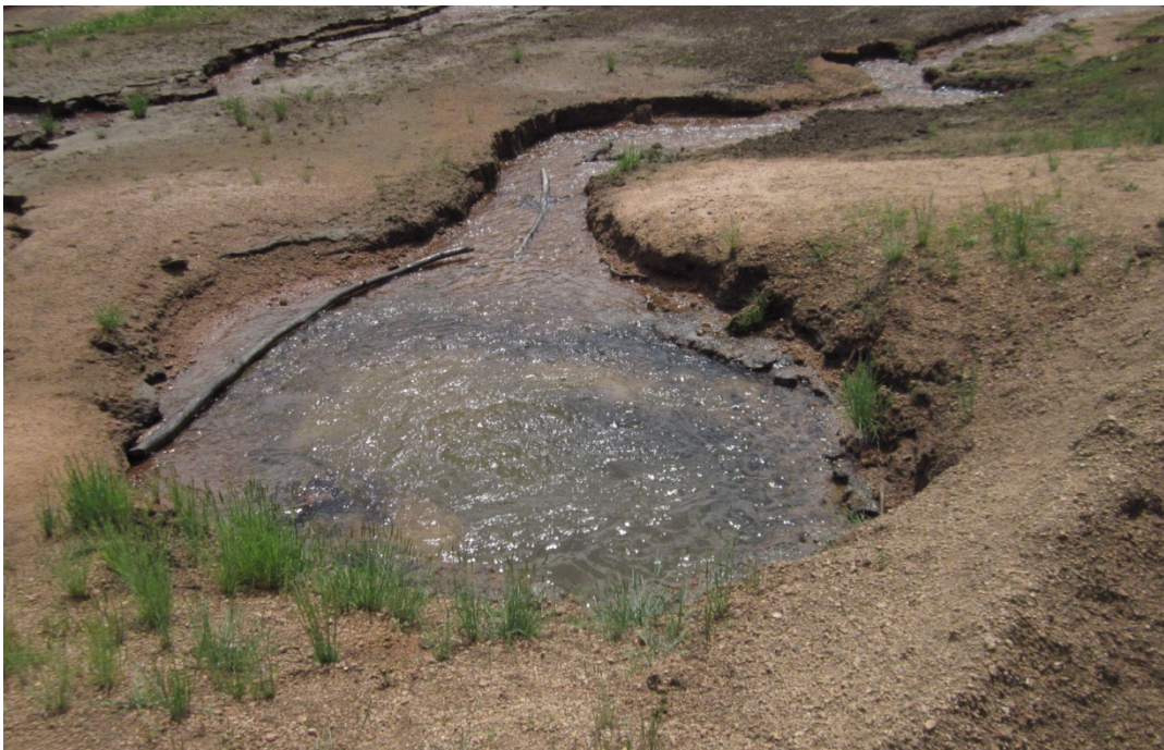
Figure 2 – Flowing water from sinkhole created by leaks in Transfer Pipe
