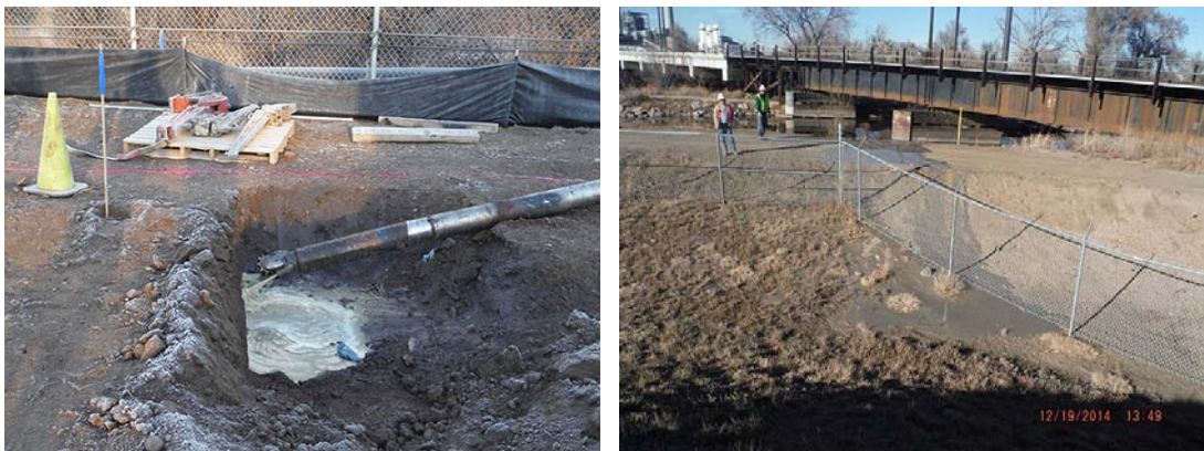
Figure 4. Pilot Jetting Assembly with Mill Tooth Bit (Left) / Inadvertent Drilling Fluid at Pothole Location (Right).
