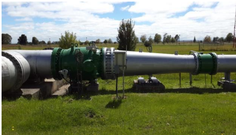
Figure 4: Kriel Reservoir inlet control valve
