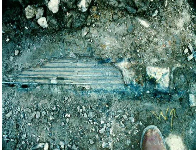
Figure 4. Joint lip shear failure in 108-inch AFM during WMATA tunneling
