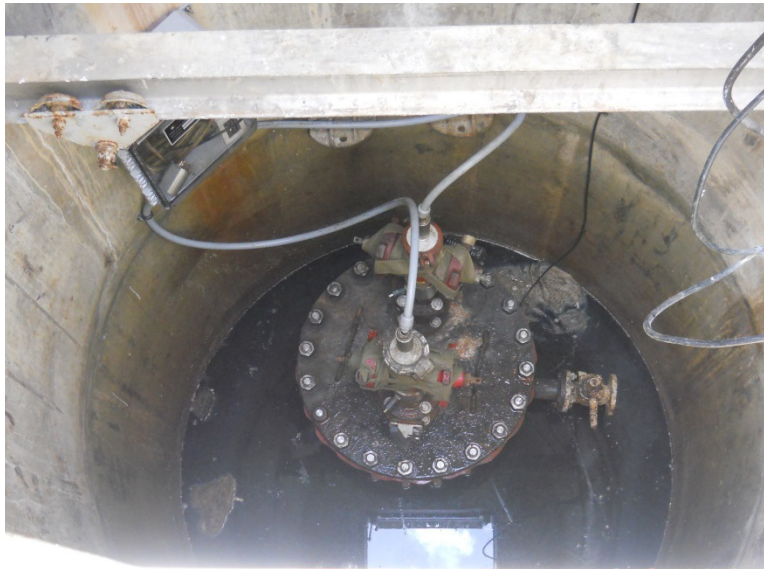
Figure 2b. External AFO Splice Point at MCUA
