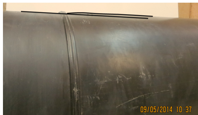
Figure 4. Pipe bulge near middle joint.
