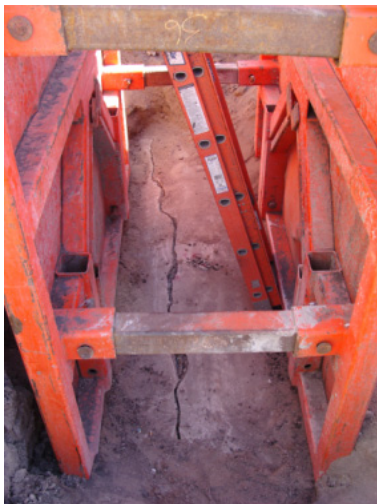
(a) Up to 1.5 in. wide crack along pipe
