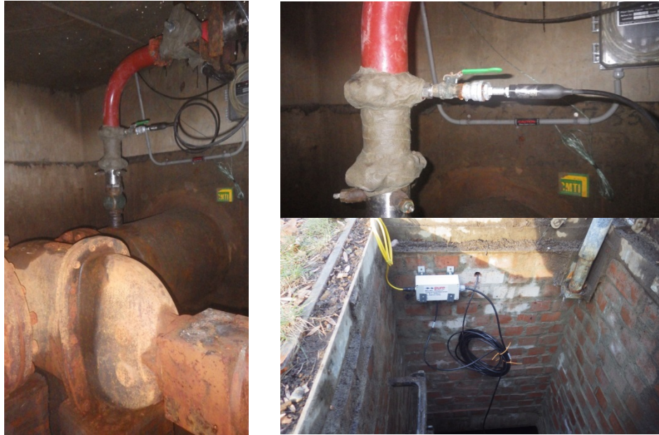
Figure 2. Telog PR-32iv Wireless Transient Pressure Monitor Installation.
