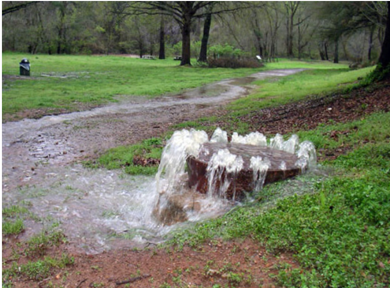
Figure 1. Sanitary sewer overflow frequently caused by undetected blockages
