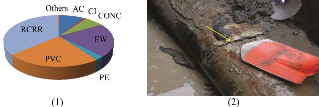
Figure 1. (1) The proportion of the Christchurch sewerage system classified by pipe materials; (2) physical damage to AC sewer pipes caused by the earthquakes.
