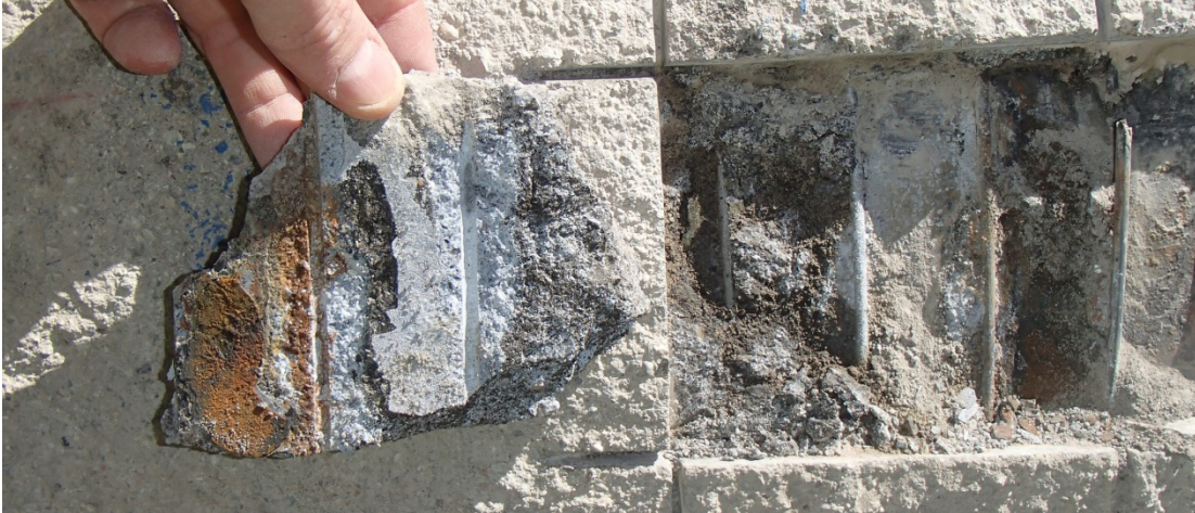
Figure 2 - Corrosion product and poor bond and steel cylinder surface of Pipeline A.
