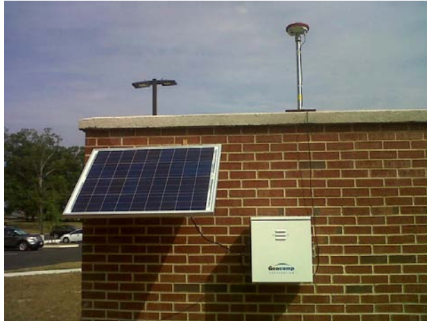
Figure 2. Solar Powered GPS Settlement & Vibration Monitoring System
