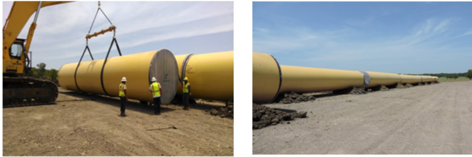
Figures 11a, b: Nylon Straps and Spreader Bar to Move Pipe, Earthen Berms for Pipe Placement
