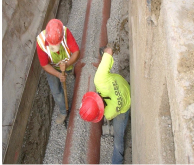
Figure 5: Shovel-slicing the bedding material into the haunches of the pipe is essential.
