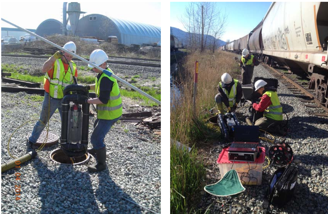
Figure 2. Deployment of and data collection with the second generation SewerVUE Multi-sensor Pipe Inspection System on a railway right-of-way in Abbotsford, BC, Canada.
