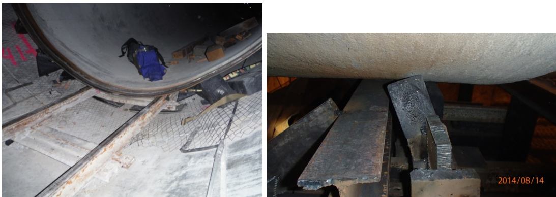
Figure 14a and b Pipe Elevation Change and Pipe Deformation
