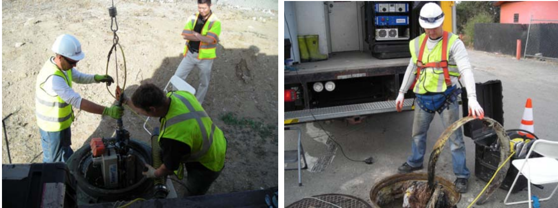
Figure 4a. Deployment of the SewerVUE Surveyor at the Del Norte Trunk Sewer, Stockton, CA. 4.b separated liner.
