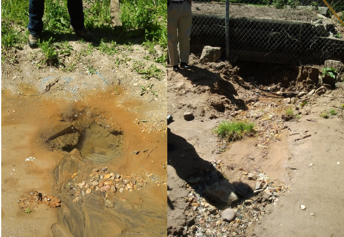
Figure 2. Pipeline leaks that surfaced near the Oak Lane Pump Station
