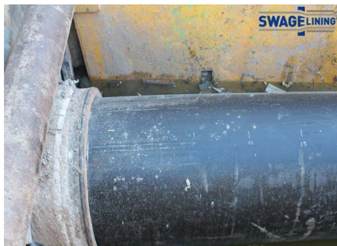
Figure 7: Tight compressive fit of HDPE after reversion.
