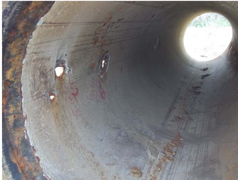
Figure 9. Pipe Section with Multiple Corrosion Spots
