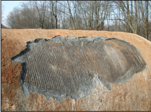
Figure 10 – Wide Spread Corrosion
