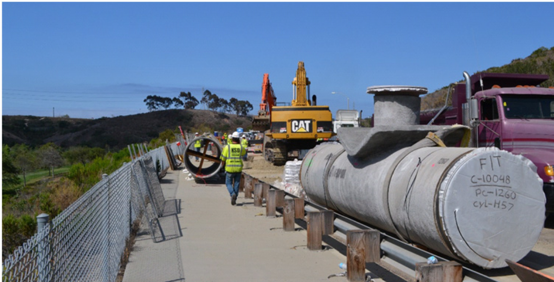
Figure 1. Construction Activity near the Startup of the Pipeline. A 54-inch diameter pipe section with 30-inch diameter outlet and single-plate crotch plate reinforcement is ready for installation.
