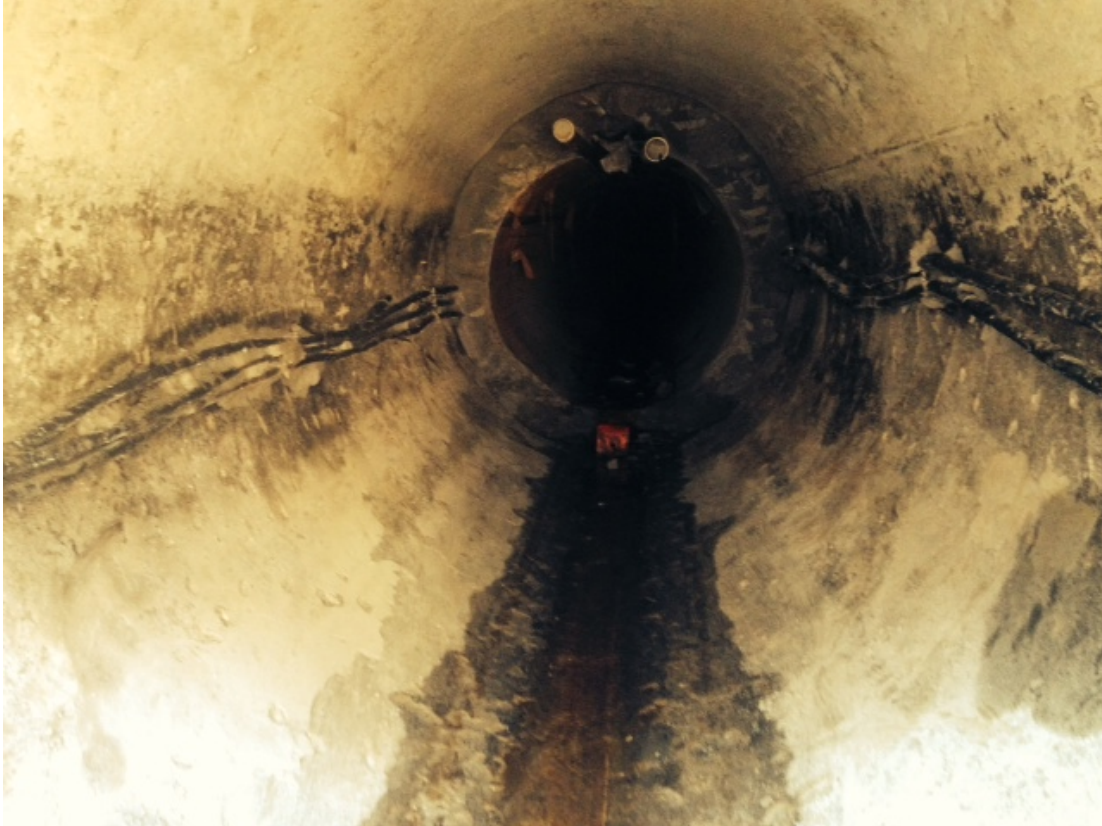
Figure 1. View inside 48 inch RCP after removal of HDPE liner and annular grout
