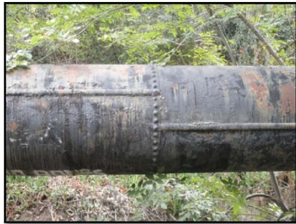
Figure 5. Exposed sections of El Capitan Pipeline lock-bars, riveted joint, and coal tar enamel coating.
