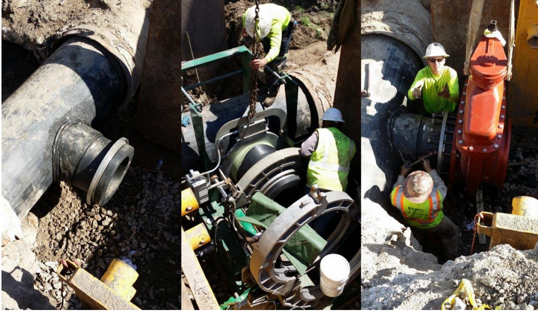
Figure 3: Left and middle picture of 24-inch stub out by sidewall fusion with Flange Adapter connected by downhole butt fusion. Right picture of 24-inch Gate Valve bolted on to Flange Adapter.
