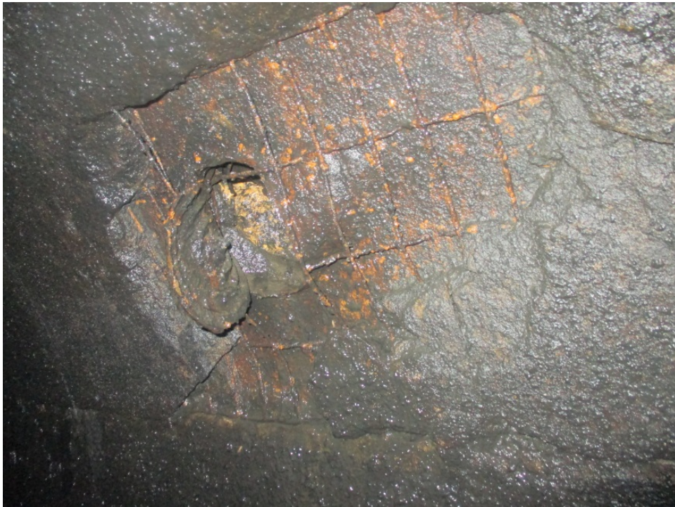
Figure 3. Hole in steel elbow pipe section
