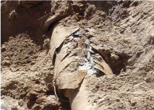
Picture 1. Fractured AC pipe resulting from pipe bursting as it will remain in the ground.
