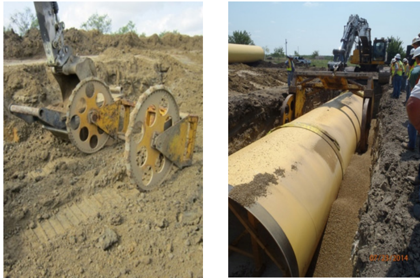
Figures 13a, b: Compaction Wheels, Application of Bedding Material in Haunch Zone in Lifts and Using Compaction Wheels
