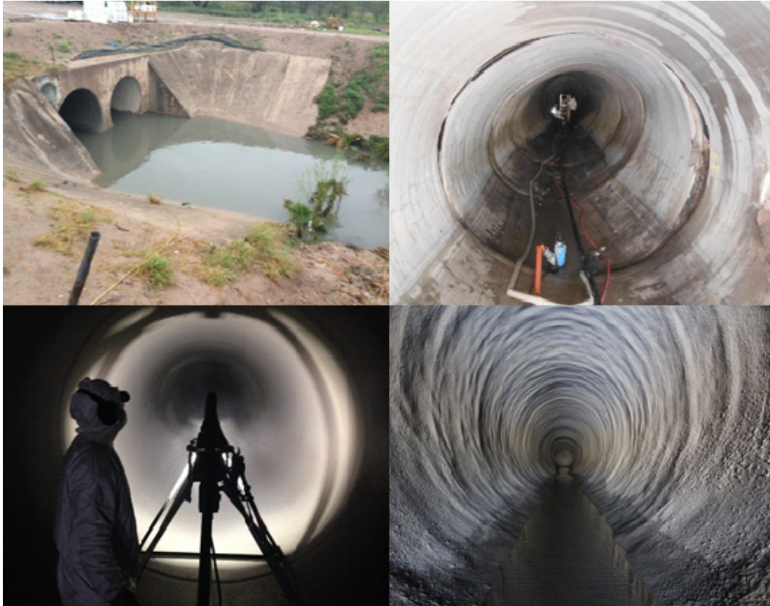
Figure 9: Images from the jobsite for the Rado Storm Drain in McAllen, TX
