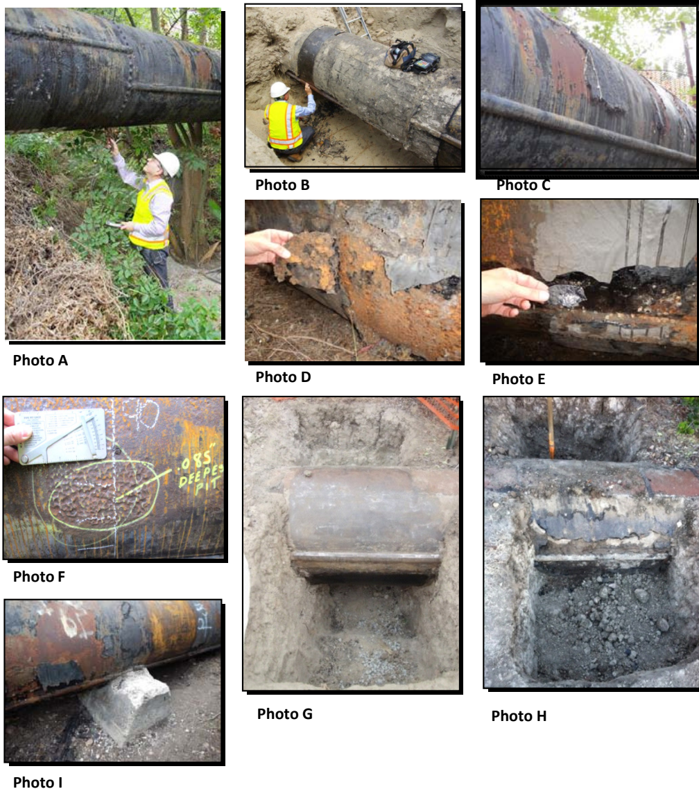
Figure 6. Photos of external examination and pit depth measurements.
