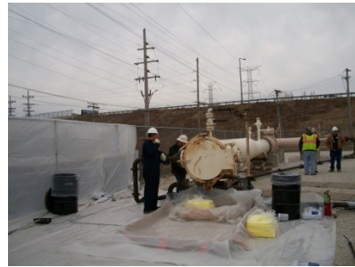
Figure 18 Environmental Containment at Receiver
