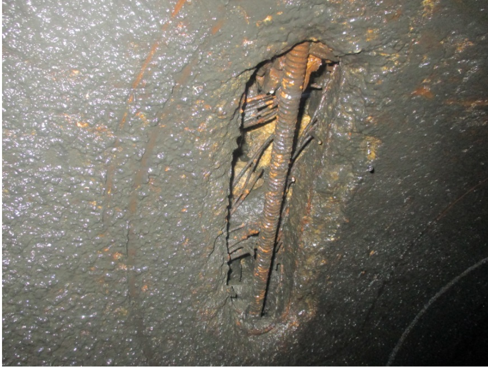
Figure 2. Soil nail going through pipe wall
