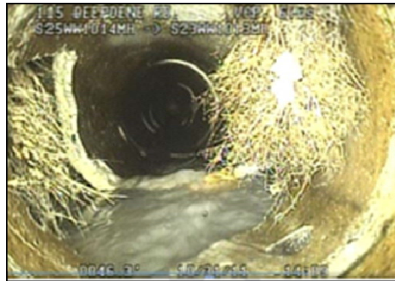
Figure 2: Typical root-intrusion in 6-inch main
