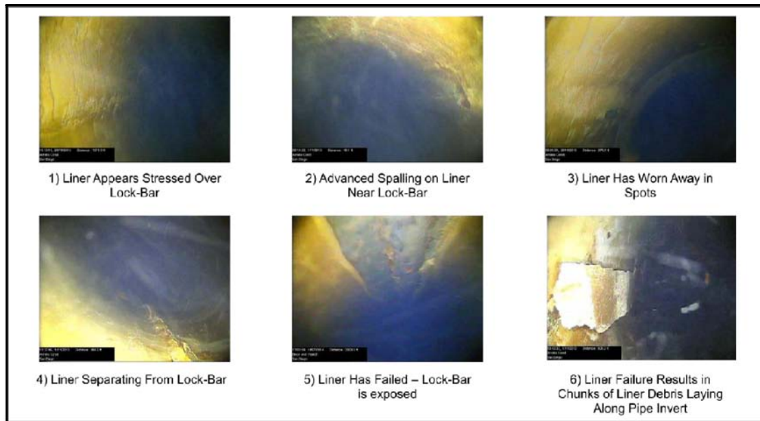
Figure 13. Six stages of lock-bar pipe liner failure.
