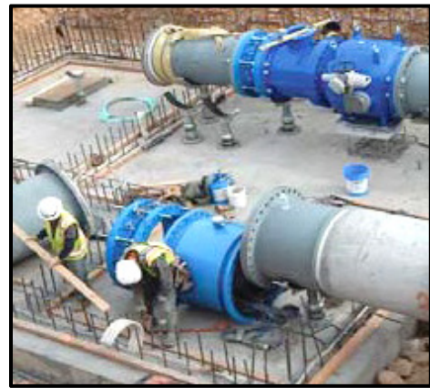
FIGURE 4. Above right is Upper Hobbble Creek Station valve room being built with 36-inch process lines. The plunger valve discharges up to 120 cfs discharge to a low head basin.
