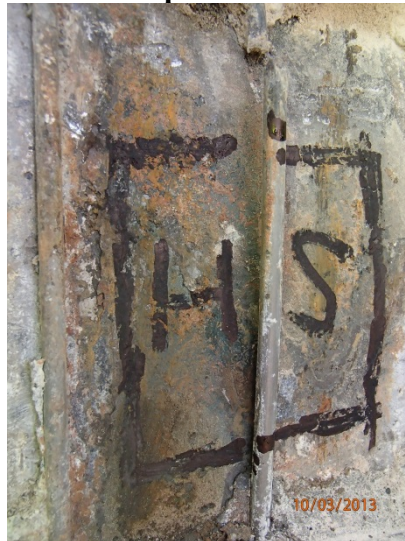
Figure 3 - Brittle broken prestressing wire and 2 in. by 2 in. hollow sounding area of steel cylinder behind wire break in Pipeline A.
