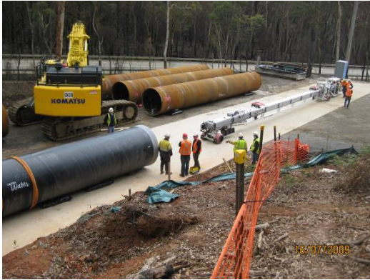
Figure 10. (left) presents a view of the pipe carrier located at the Retrieval portal.
