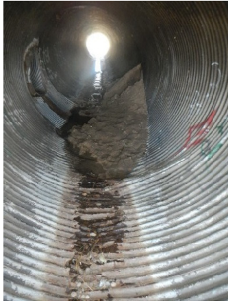
Figure 2. CMP joint failure.
