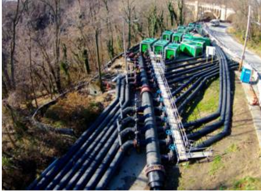
Figure 1. By-pass system installed for the SWDS Project
