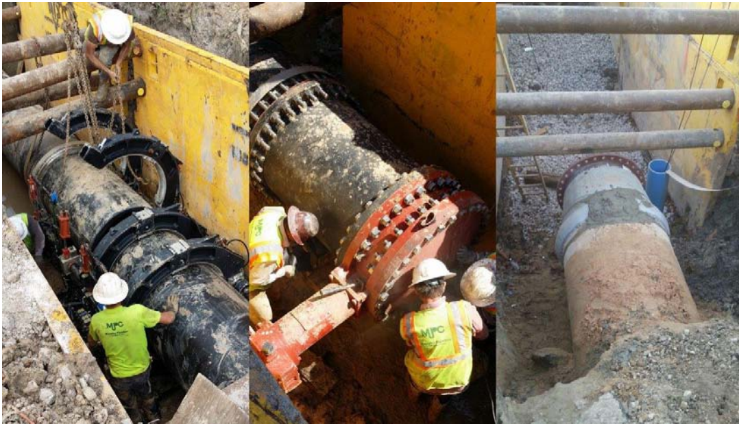
Figure 4: Left picture of downhole butt fusion connecting HDPE in receiving pit. Middle picture of 36-inch side actuated butterfly valve. Right picture of 39-inch by 36-inch PCCP flange reducer.
