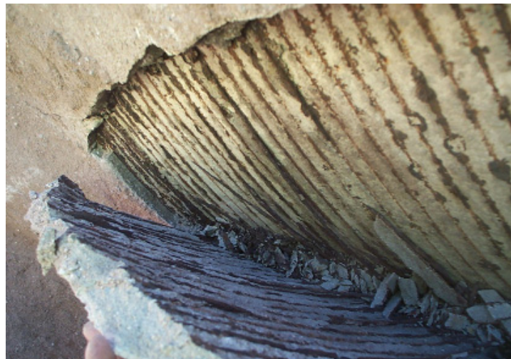
(b) Wire impressions left on concrete core after wires were fully corroded away
