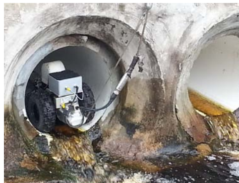
Figure 3: Photograph showing the robot entering storm drain rehabilitated by slip lining method.
