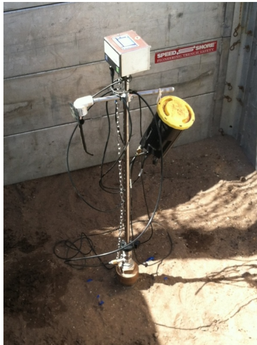
Figure 3. Finished Water Meter Testing using a Temporary Insertion Flow Meter.
