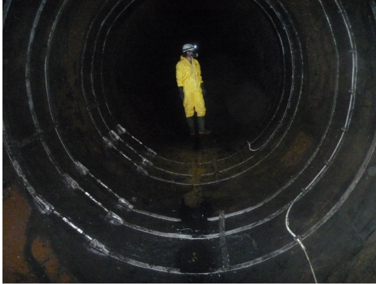
Figure 2a. Internal AFO Splice Point at MCUA
