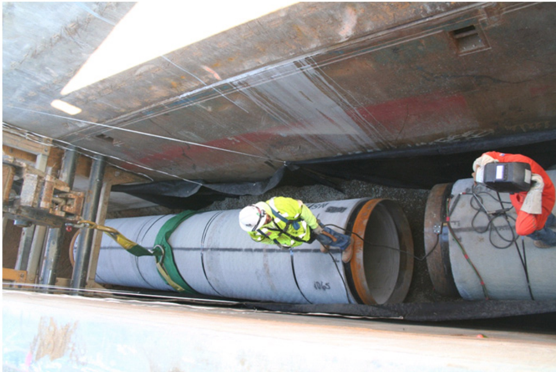
Figure 4. Lap Joint Assembly. The pipe section on the left hand side is being positioned opposite the already installed pipe section for lap joint assembly and welding.
