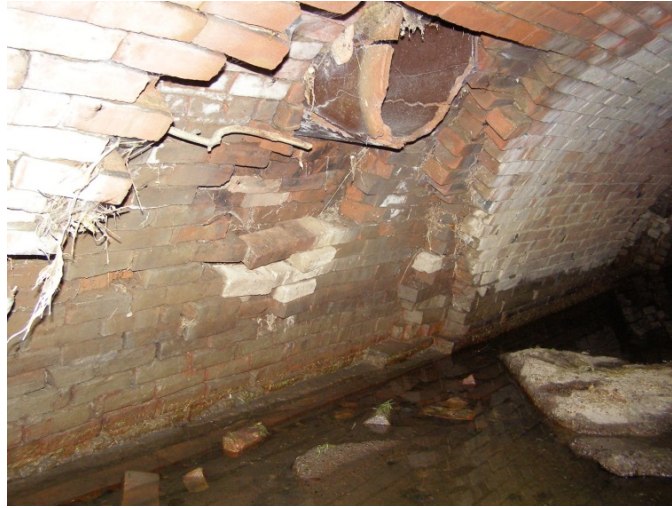
Figure 2. Photo of Missing Bricks in Wall at North Street, Pre-Rehabilitation
