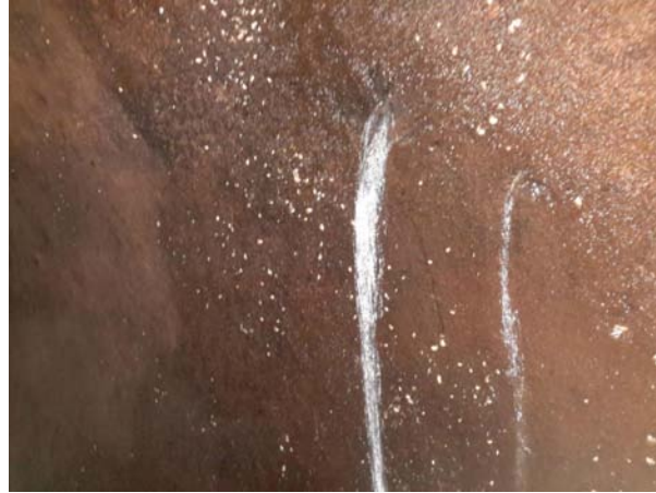
Photo 5. Grossmont Tunnel Joint Leaks
