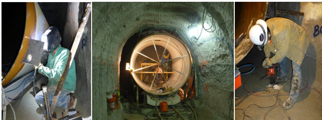
Figures 12a, 12b and 12c. Pipe Bracing.
