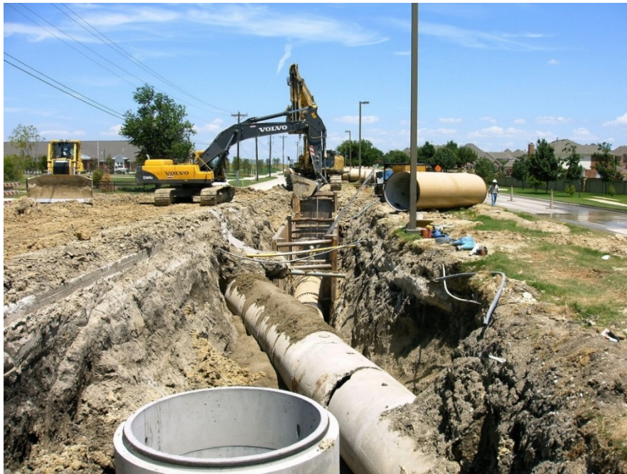
Figure 1 – Allen-Plano-Frisco-McKinney Pipeline Construction down a median with multiple utility conflicts and partial road closures.
