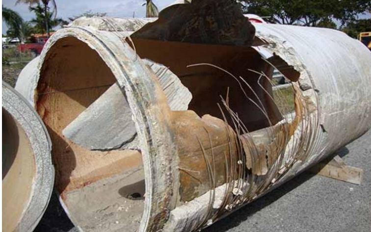
Figure 1 – Ruptured 54-inch PCCP water transmission main
