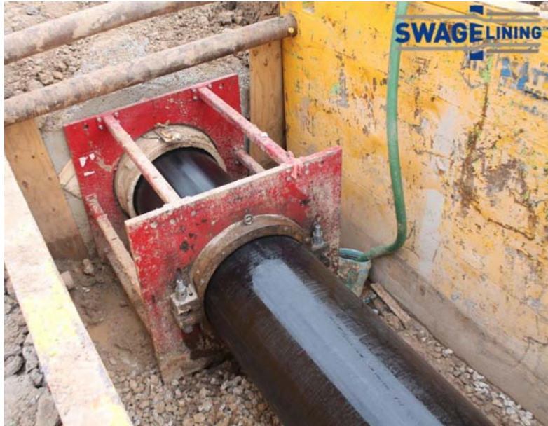
Figure 6: 1000mm (39.4-inch) OD HDPE pipe enters single swage die. The HDPE pipe is temporarily reduced below the ID of the 39-inch PCCP host pipe to allow for insertion.
