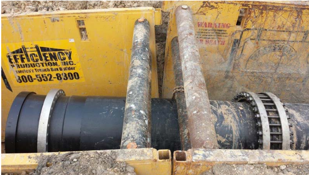
Figure 5: HDPE connections using Flange Adapters with stainless steel back up ring and stainless steel bolts.
