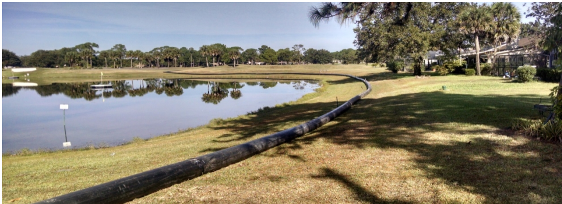
Figure 2. Force main bypassing
