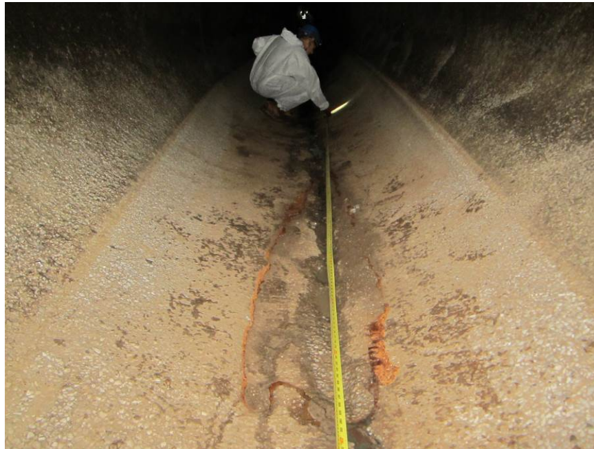
Figure 5. Deterioration observed at the invert of the pipe
