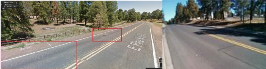
Fig. 1. Road surface with pothole and cracking (L) and smooth condition (R)
