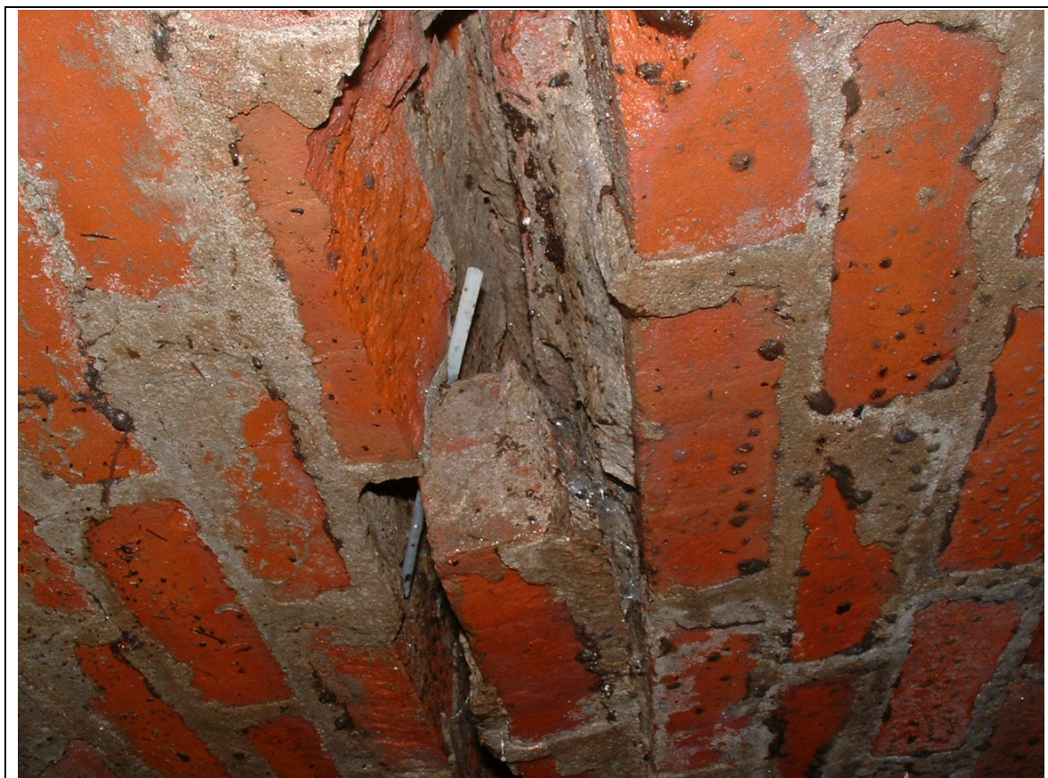
Figure 2 showing a separation at the crown of the conduit
