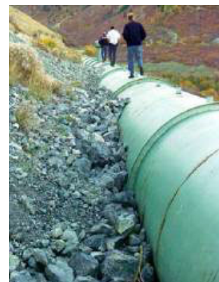
FIGURE 14 Talus buildup on pipe.
