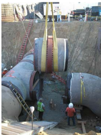
Photo 7 - Insulating Flange Assembly
