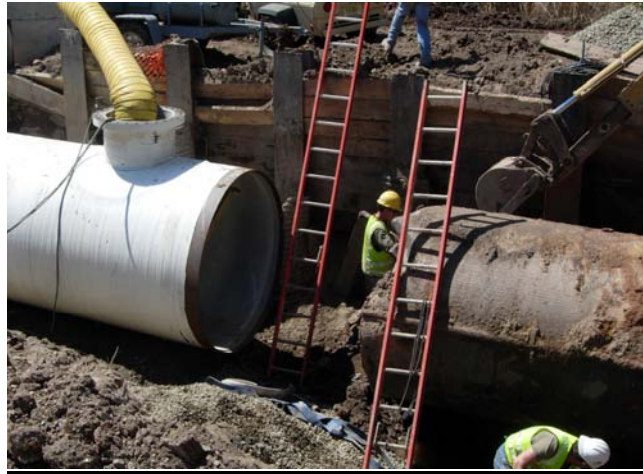
Figure 2. 1906 72” Steel Pipe connected to new Steel Pipe in NJ (National Welding Corporation, 2006)
