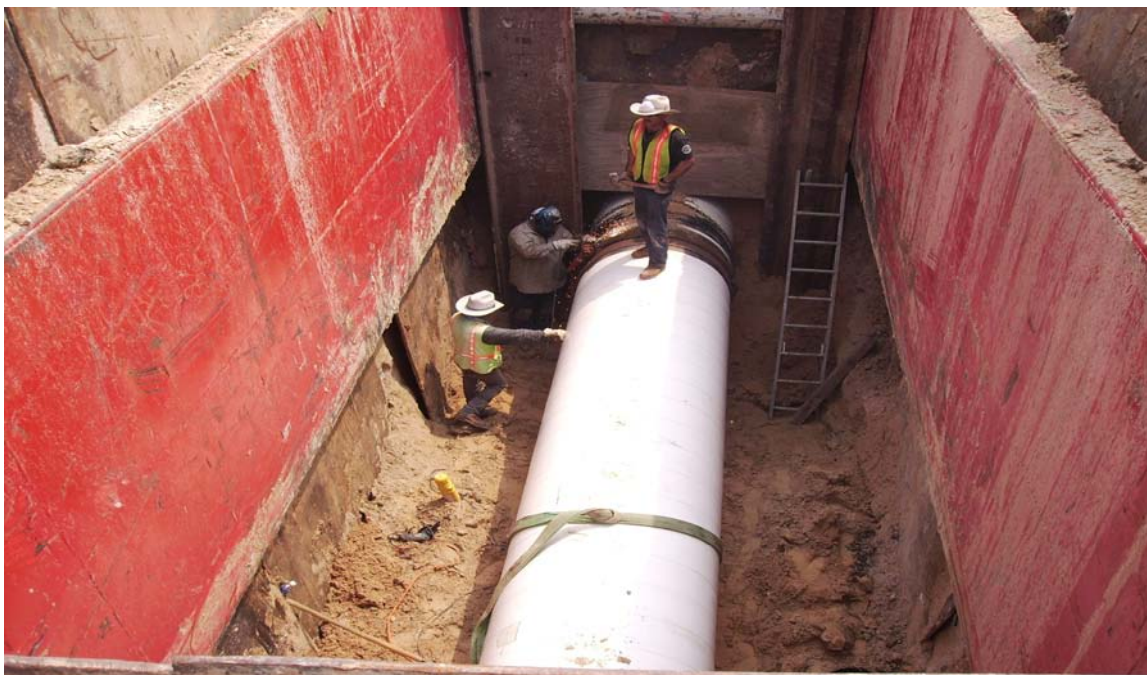
Photo 4: New segment used to replace MK #23, being installed with the use of a butt-strap between MK #23 and MK #24.
