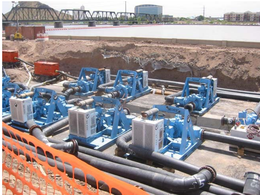
Figure 3 – In this planned outage a temporary bypass of a sewer main allows installation of cured-in-place lining (Pipetech International Photo)
