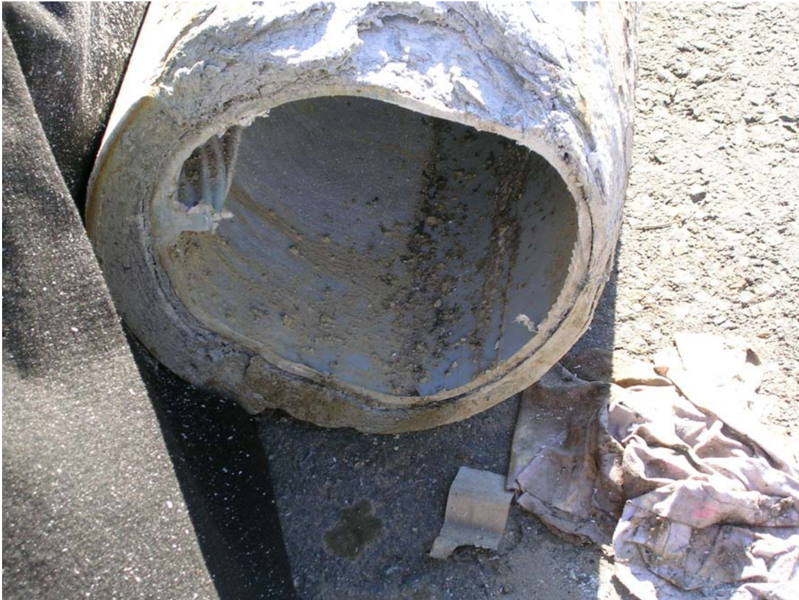
Figure 3: Fold on CIP liner inside AC pipe (9 O'clock position).
