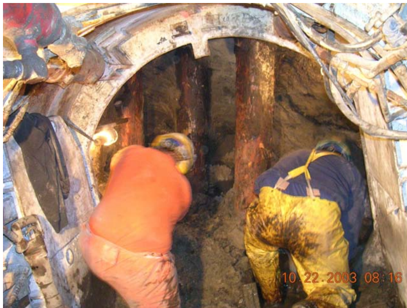
Figure 5. Chemically grouted soil is excavated by hand, and timber piles cut with hydraulic chainsaws and removed. Obstruction removal required some minor excavation ahead of shield.
