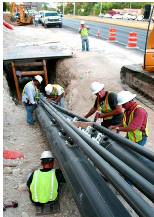
Figure 6 - Bundling our pipes was done in the early morning hours and pipe was pulled inside the casing as the bundles were assembled. A special rack was fabricated to facilitate this operation. Additional tightness was obtained by utilizing a canvas strap to bundle the pipes prior to tightening the steel straps.
