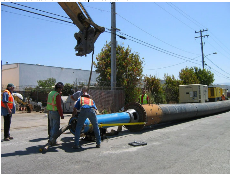
Figure 6 – Setting up the rear dynamic impact pushing tool. An 18-inch diameter pneumatic hammer is setup in a pipe rammer configuration to assist the heavy pipe string along during pipe bursting operations. This added ramming technique improved pipe bursting production over 50% in the Bay mud conditions present. This rear tool was in operation at the same time as the lead tool and lubrication system.
