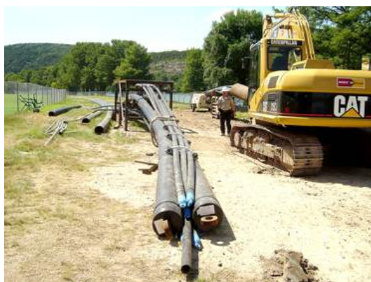
Figure 7 - A special rack was fabricated to facilitate the pullback operation while maintaining correct separation between the multiple HDPE conduits.
