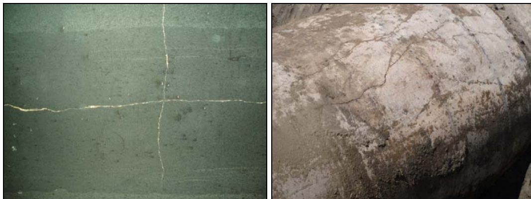
Figure 3 - Longitudinal cracks on pipe R329 (internal and external)
