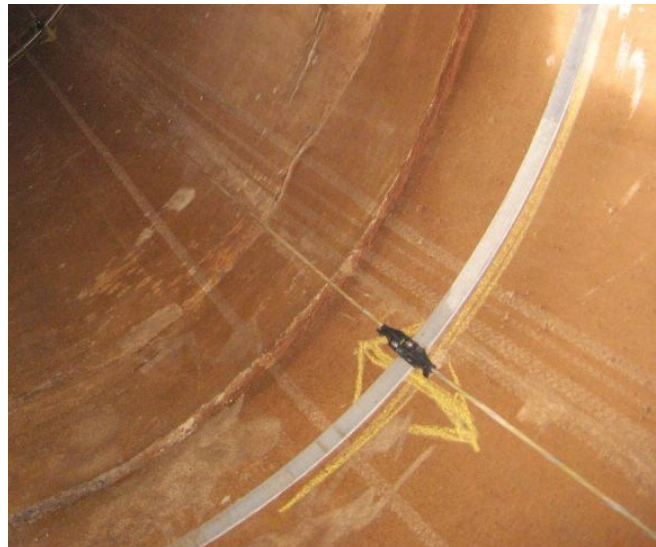
Figure 6: Steel strap and strain relief connection used to attach fiber optic sensor to the interior pipe wall of the 102-inch aqueduct.
