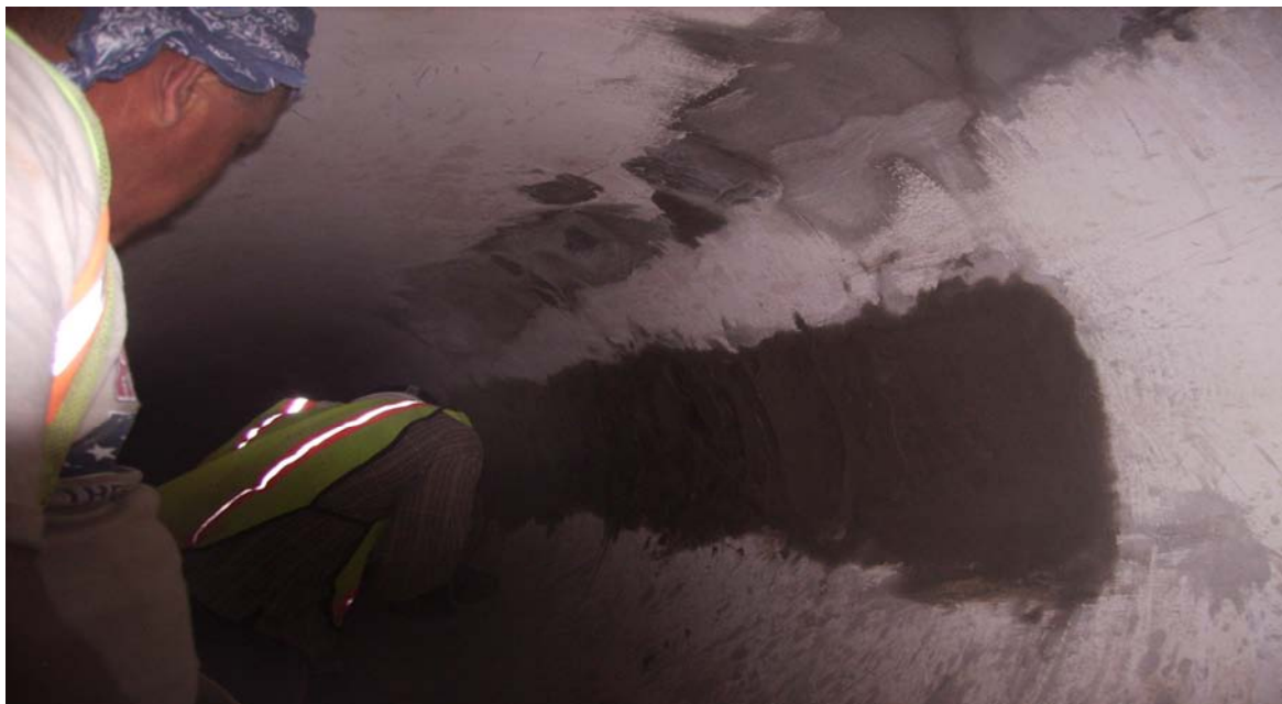
Photo 7: Grout being used to repair a portion of mortar lining which had delaminated from the steel cylinder in MK #33.
