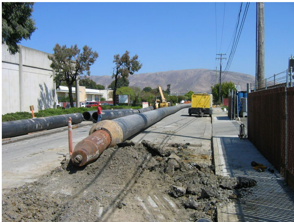
Figure 2 – New 36-inch O.D. HDPE pipe with 24-inch pneumatic hammer and 42-inch diameter pipe bursting expander ready to launch.
