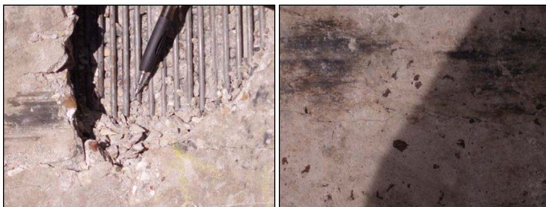
Figure 2 - Broken prestressing wires and external longitudinal crack on pipe R332
