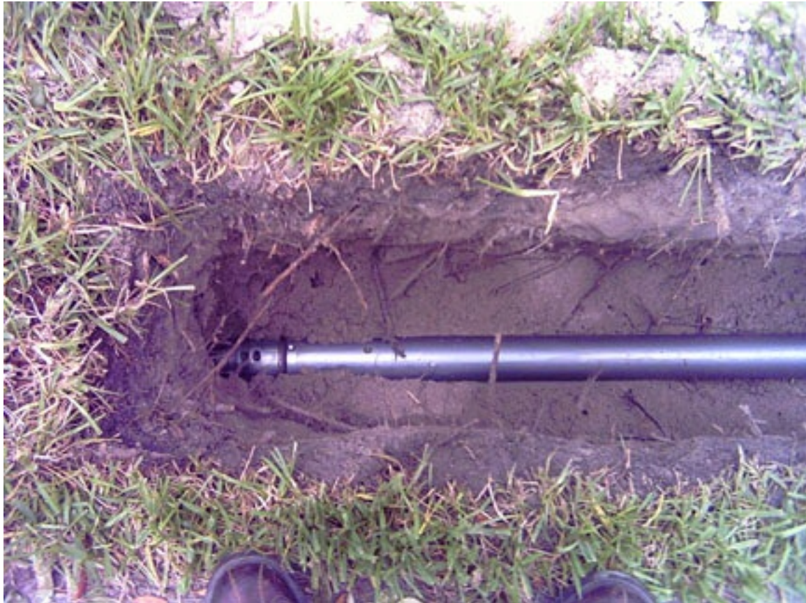
Figure 6 Launch excavations for Piercing tools are normally quite narrow and just long enough for the tool to lie flat on line and grade of the bore.
