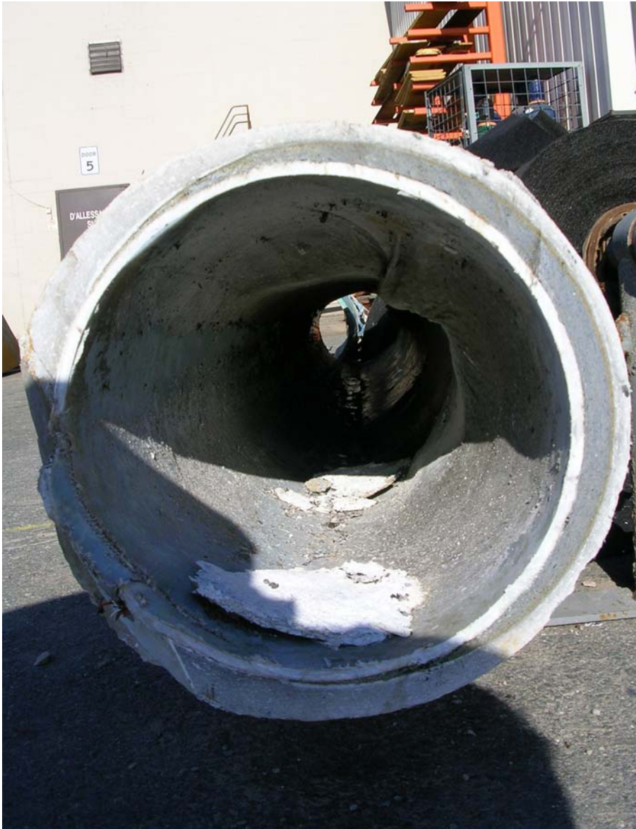
Figure 5: End section of AC pipe showing varying material thicknesses.
