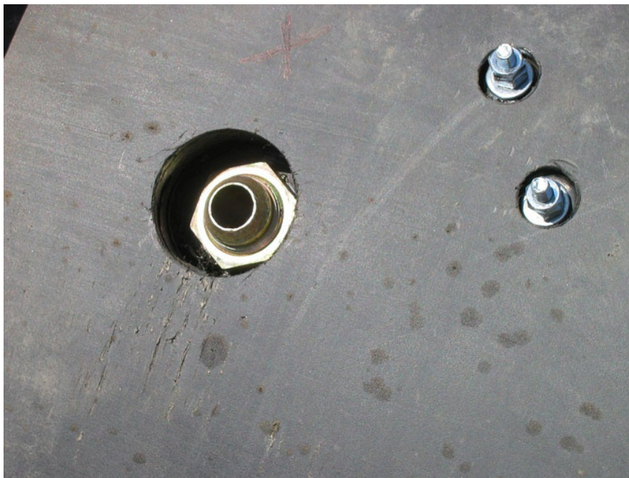
Figure 3 – Typical discharge port for polymer slurry. This assists the new pipe through the sticky Bay Mud during pipe bursting operations. This port is located directly behind the pipe bursting expander.
