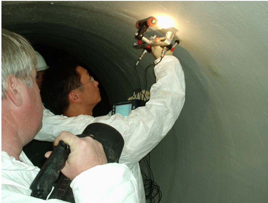
Figure 3 - inspection for “bubble trouble”
