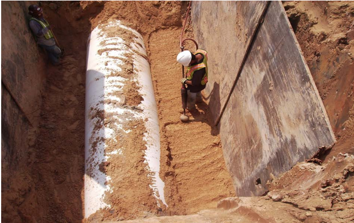
Photo 2: Worker using pneumatically powered hand-held rammer to compact soil around MK #143 as the pipe is backfilled.
