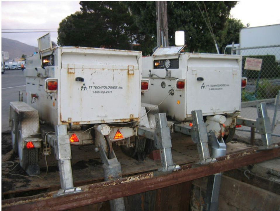
Figure 7 – Dual 20-ton constant tension winches setup over the receiving pit. The added winch tonnage was required because of the overall weight and size of the pipe bursting equipment and the dead weight of the new 36-inch HDPE pipe. Typical winch tension was 30 tons (each winch operating at 15 tons x 2 = 30 tons). Additional tonnage was available as needed up to 40 tons.
