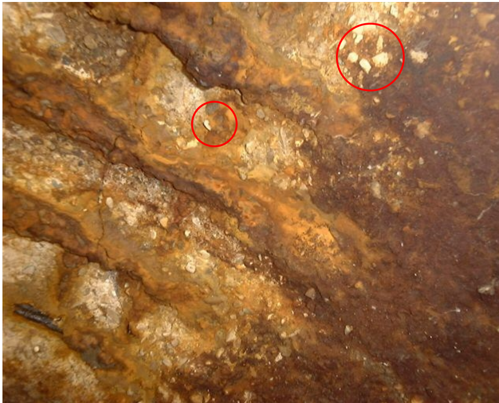
Figure 1. Close-up of a 36 in concrete sewer pipes that experienced severe MIC. The steel reinforcement ribs are either gone or in an advanced corrosion state. The white solids are MIC corrosion products (marked by red circles)
