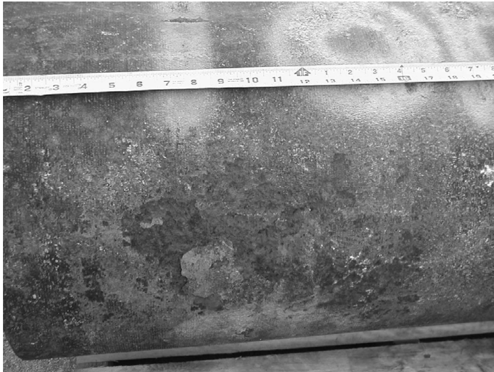
Figure 1 - Corrosive Attack to 16" Ductile Iron Pipe (71% wall max pit depths)
