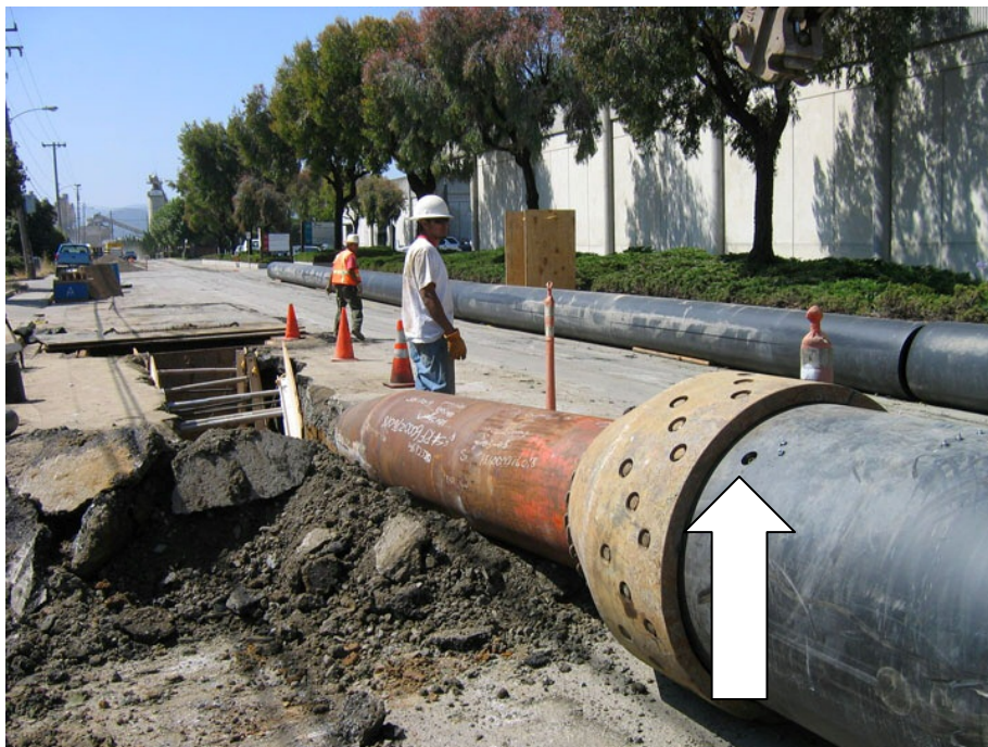
Figure 5 – Note the position of the lubrication discharge port. Also shown are the numerous Grade 8 Bolts securing the HDPE pipe to the pipe bursting expander. Observe that the street is open to traffic.
