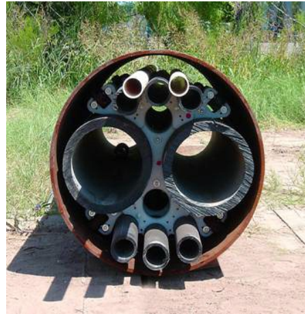
Figure 5 - Based on the mock up results, grouting operations were done in phases. The first two phases consisted of sealing the center sections of each line segment to create a plug. This was followed by grouting at either ends to completely fill the voids. Batch tests of the grout was collected at each phase to determine the Thermal Resistivity of the mixes and verified that grout batches met the specified requirements. Pressure and mandrel testing of pipes were completed after the grout was cured and verified the internal diameter of all conduits met the deflection limits specified.
