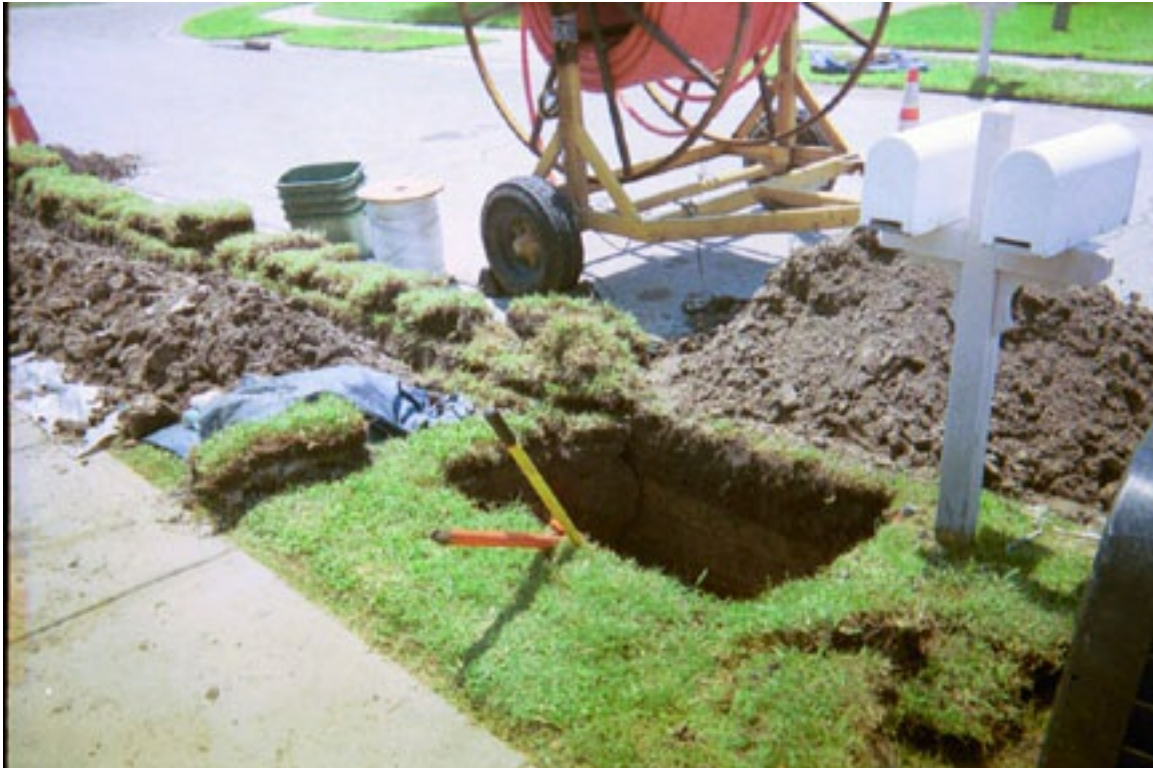
Figure 5 A typical excavation for an FTTH service. This excavation is approximately 2 x 4 feet. Depth is 24-30". Note the reel of conduit, utility boxes, roll of mule tape, turf to be replaced, hand tools and excavated material. Note that the excavated material is placed on plastic sheeting to protect the turf underneath. The mail box was not disturbed.
