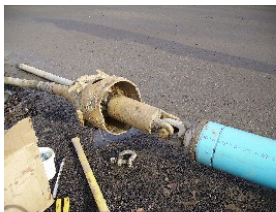
Pullback – Drill rod with reamer attached to swivel in front of lead pipe, ready to commence installation
