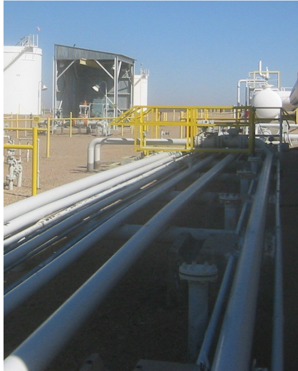
Figure 1 – Petroleum pipeline booster station, Colorado. The petroleum pipeline industry is regulated in planning for risk management (Pipetech International photo)
