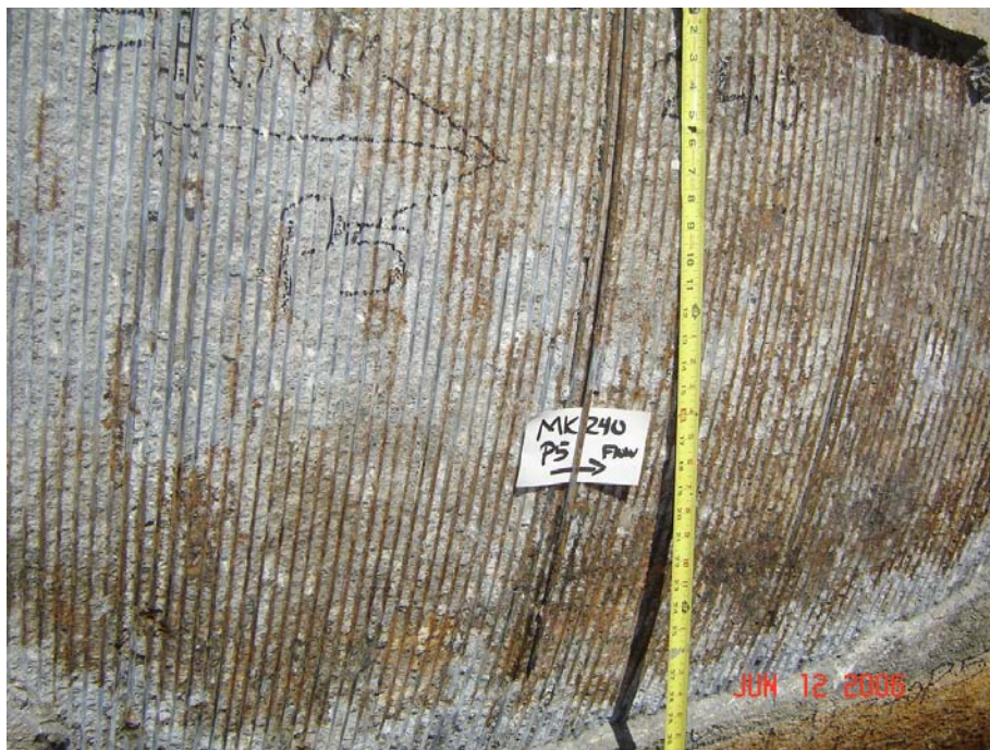
Figure 3 – Damaged wires and corroded area
