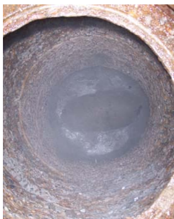
Figure 1 Interior – Deteriorated Manhole
