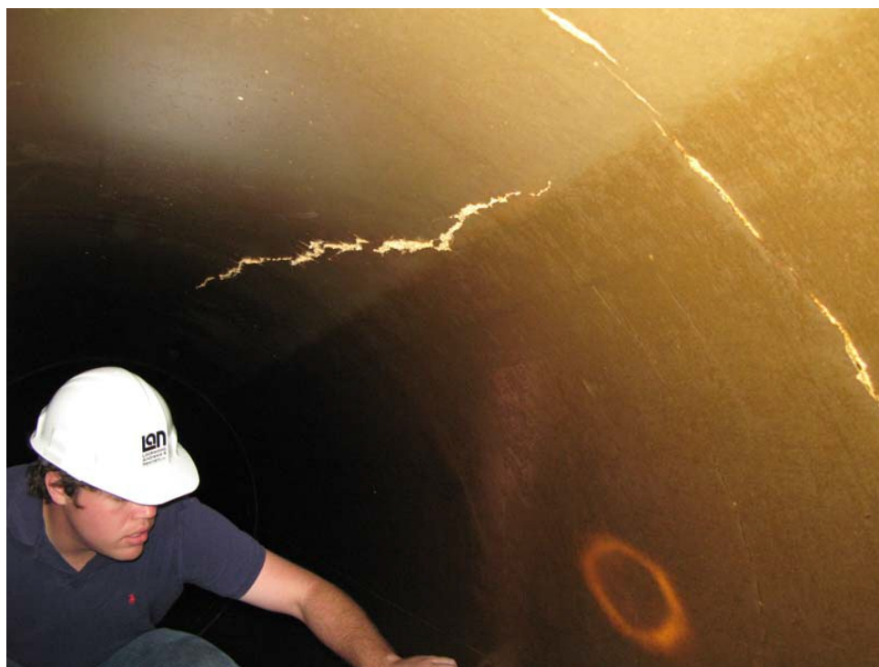
Figure 5. Longitudinal and circumferential damage in PCCP pipe
