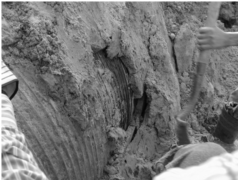
Exhibit 4. Delaminated mortar coating
