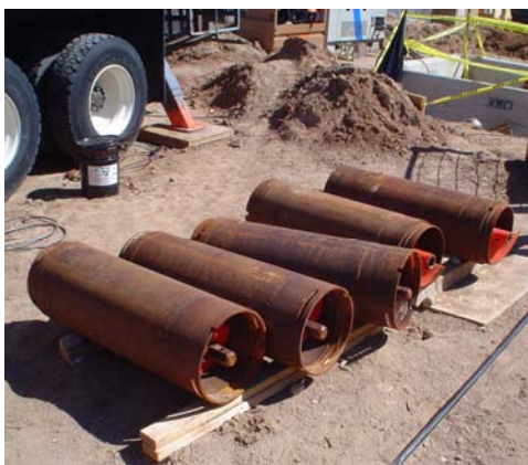
Figure 8- 1 meter length auger flights and steel casings ready to be lowered and jacked into place for spoil removal on the second step in the three pass method.
