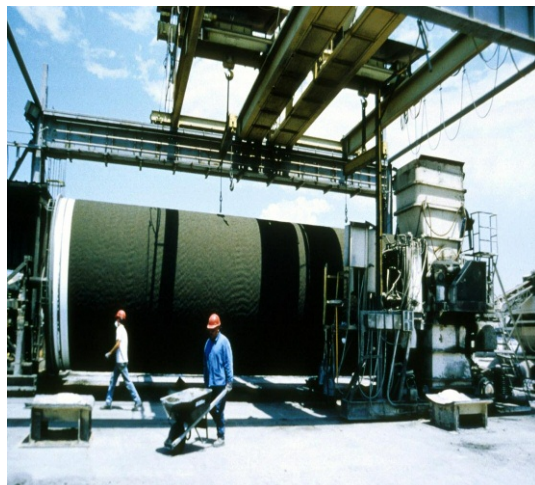
Figure 5. Impacted cement mortar on large diameter WSP.
