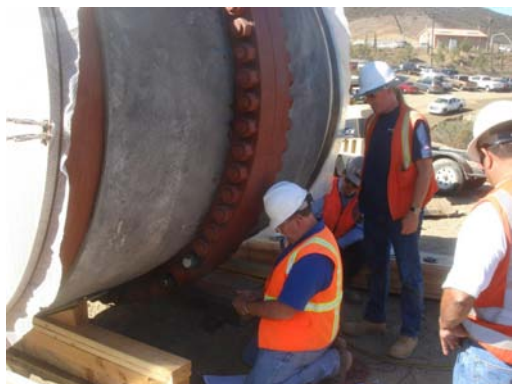
Photo 5 - Bolts Retested at Site
