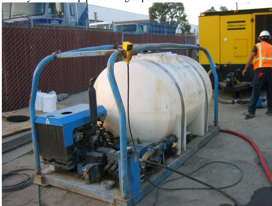
Figure 4 – 500 Gallon mixing and pumping system to supplies lubrication that assists with pipe installation during pipe bursting operations.
