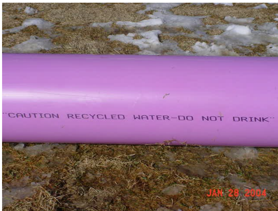
Figure 6 – Photo of purple PVC pipe with warning.
