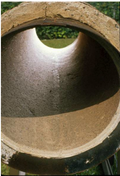
Figure 1. 12-inch diameter riveted steel with concrete lining & field applied conc. coating installed in 1855.
