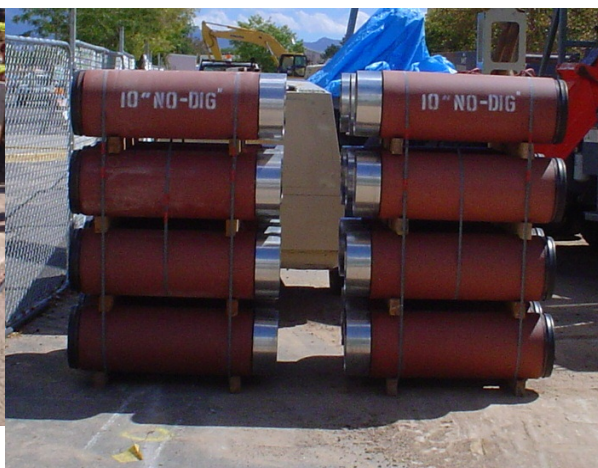
Figure 9- 1 meter length by 10 inch ID product pipe which are installed directly behind the auger casings on the third step in a three pass system. The OD of these product pipes are equal to the OD of the previously installed casings.
