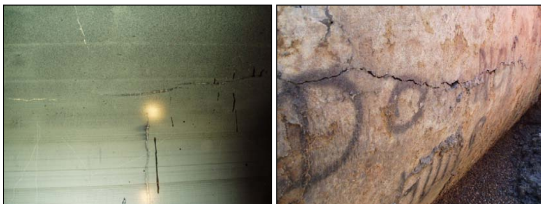
Figure 4 - Longitudinal cracks on pipe R345 (internal and external)
