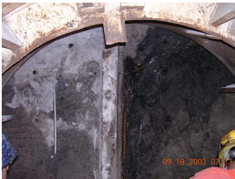
Figure 4. 54-inch shield. On left side, reinforced concrete and concrete-filled sheet pile of abandoned vault. On right side, chemically grouted clean fill.
