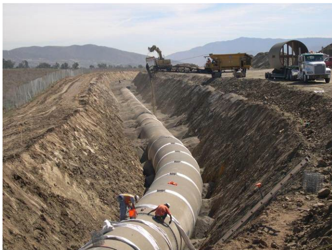
Figure 8. The joint grout bands are filled with cement mortar grout ahead of backfilling with granular material through a Shute.
