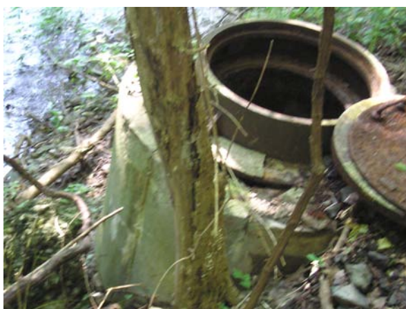
Figure 2 Exterior – Deteriorated Manhole
