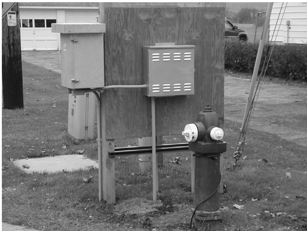
Figure 4 – Rectifier and Anode Box (rectifier negative is connected to hydrant)
