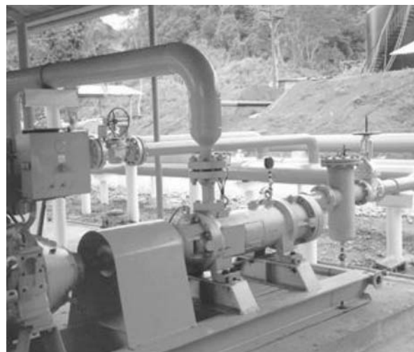
Figure 8. Diesel-driven three-screw pump at 1400 psi.
