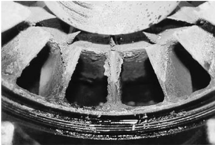
Figure 11. Fouled inlet guide vanes on hydrogen recycle compressor.
