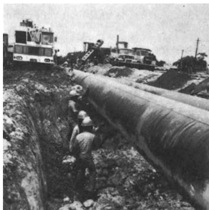
Hand cleaning. The 30-in. and 36-in. crude lines were cleaned by hand to expose corroded areas and prepare for tape wrapping.
