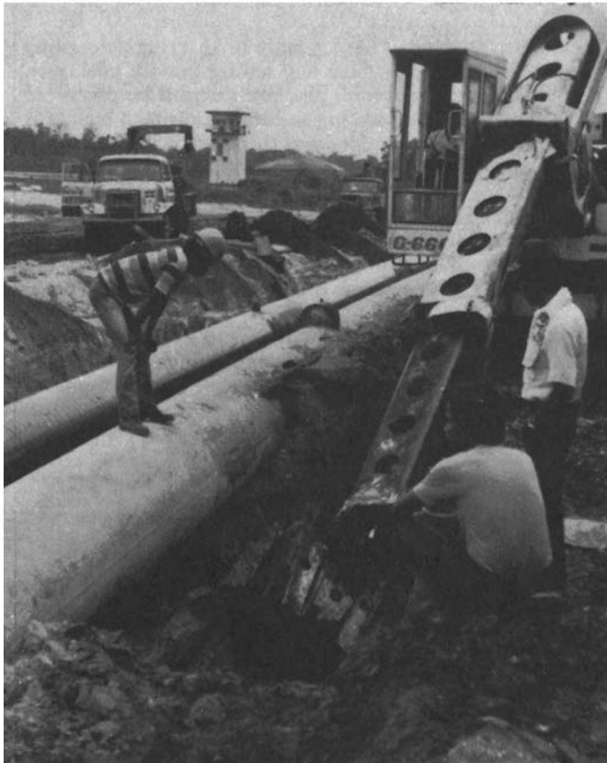
Excavation begins. Ten-foot soil plugs remained at 50-ft centers to act as temporary pipe supports for the 36-in. line.
