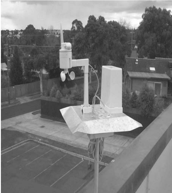
Figure 13-1. La Crosse weather station installed on a roof
