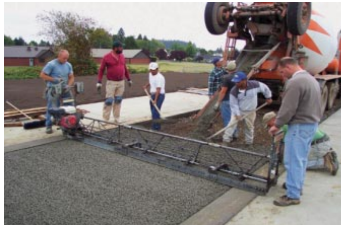
Figure 11. Pervious concrete is usually placed and then struck off with a vibratory screed. (R. Banka) [IMG15891]
