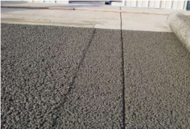
Figure 12. Pervious concrete after screeding (left) and after compaction (right). Note the joint aligned with previously placed slab to avoid reflective cracking. Roller used for compaction is visible on the far right. (R. Banka) [IMG15892]
