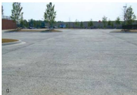
Figure 2. Example applications of pervious concrete. (a) Oregon zoo sidewalk, Portland, OR (P. Davis) [IMG15881]; (b) Miller Park in Fair Oaks, CA, (A. Youngs) [IMG15882]; (c) Finley Stadium parking lot, Chattanooga, TN (L. Tiefenthaler) [IMG15883]; (d) Imperial Beach Sports Park, CA (D. Akers) [IMG15884]; (e) Storage facility lot, Mt. Angel, OR (R. Banka) [IMG15885]; (f) Colored pervious concrete walkway, Bainbridge Island, WA (G. McKinnon) [IMG15886]; (g) Large concrete parking lot, Buford, GA (L. Tiefenthaler) [IMG15887]
