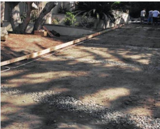
Figure 8. Preparation for a sloped installation. Crushed rock drains at intervals down the slope direct water away from the pavement and prevent water from flowing out of the pervious concrete (See also Figures 9 and 10). (S. Gallego) [IMG15890]
