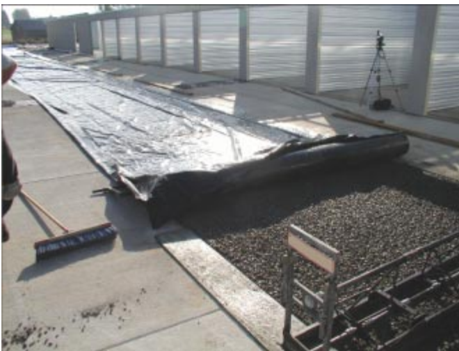
Figure 15. Plastic sheeting should be used to cover the pervious concrete and be installed within a few minutes of consolidation to prevent moisture loss. (R. Banka) [IMG15898]
