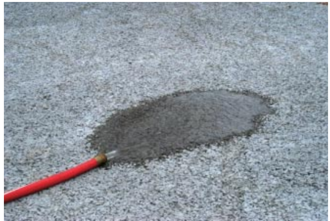
Figure 1. Pervious concrete's key characteristic is its open pore structure that allows high rates of water transmission. Trail in Athens Regional Park in Athens, TN, (A. Sparkman). [IMG15880]
