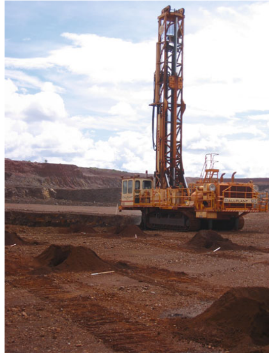
Fig. 4.21 Drilling blastholes using truck mounted open hole percussion drill rig, Yandi iron-ore mine, Western Australia
