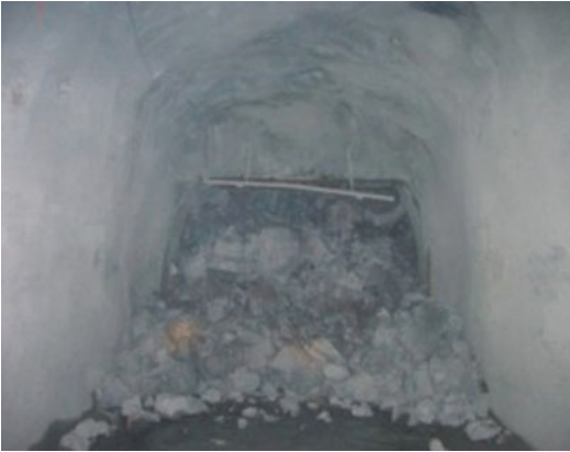
Fig. 5.5 Broken ore at the draw point of the underground stope at the Northparkes copper mine
