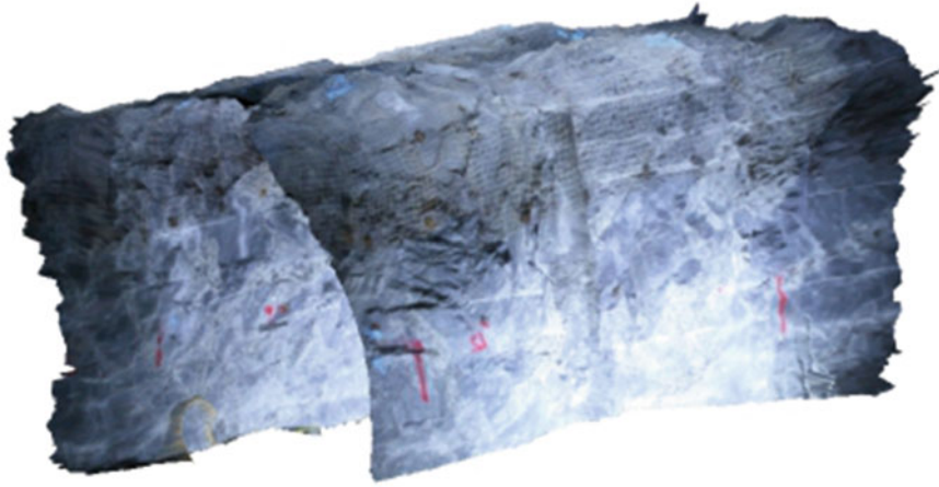
Fig. 3.18 Detailed 3D image of part of the underground drift (8 m long) recorded using ADAM photogrammetric technology, Diavik diamond mine, Canada
