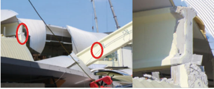
Fig. 4.11 Collapse of the beam during Emilia earthquake due to the loss of the seating; general view – left and the detail of the support – right (Bournas et al. 2013a)
