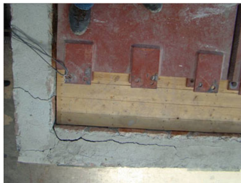
Fig. 8.7 Separation of the leaves of masonry walls during tests on the shaking table (Mouzakis et al. 2012a)
