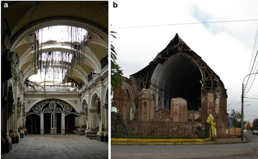
Fig. 15.2 (a) Ica cathedral, (Peru') collapse of the timber barrel vaults. (b) Collapse of the brickwork façade of the Church San Francisco of Curico', revealing the timber structure supporting the roof. Maule, Chile
