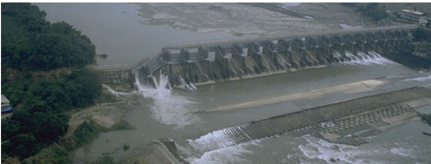
Fig. 20.2 Failure of two openings of the Shih-Kang weir caused by fault movements during the 1999 Chi-Chi earthquake in Taiwan
