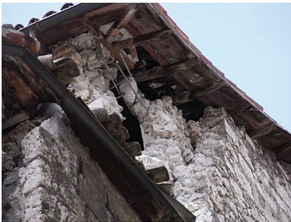
Fig. 15.5 Partial collapse and evidence of a reinforced masonry ring beam in the Church of Santa Giusta in L'Aquila
