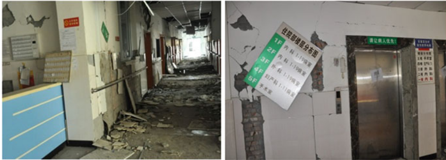
Fig. 14.10 Damage suffered by the two conventionally founded buildings of the hospital of Fig. 14.9 (Zhou et al. 2013)
