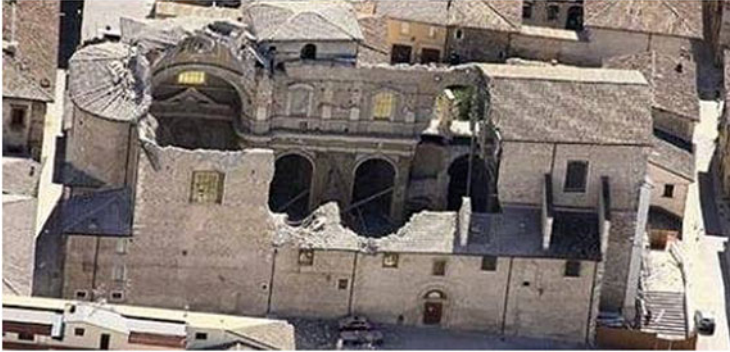
Fig. 15.4 Collapse of the roof and vaults of the church of Santa Maria Paganica, L'Aquila
