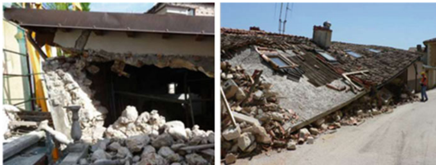
Fig. 8.30 Catastrophic effect of RC slabs on poor quality (unstrengthened) masonry (courtesy of Prof. C.Modena)
