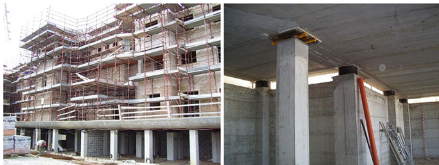
Fig. 14.24 Left : seismically isolated dwelling building complex under construction in Ozzano Emilia (Bologna), irregular in shape (61 m \times 28 m; 2 buildings with 2 staircases, connected to the second floor; 4 isolated above ground isolated floors, with the isolators installed in the non-isolated basement). Right : some of the isolators of the building (61 HDRBs and 56 SDs)
