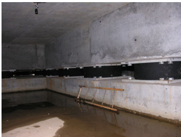
Fig. 14.13 Some of the 193 HDRBs, manufactured in Italy, which protect the building of Fig. 14.12 (picture taken on September 23, 2011, during the 2011 Sochi Conference) (Martelli et al. 2012a)
