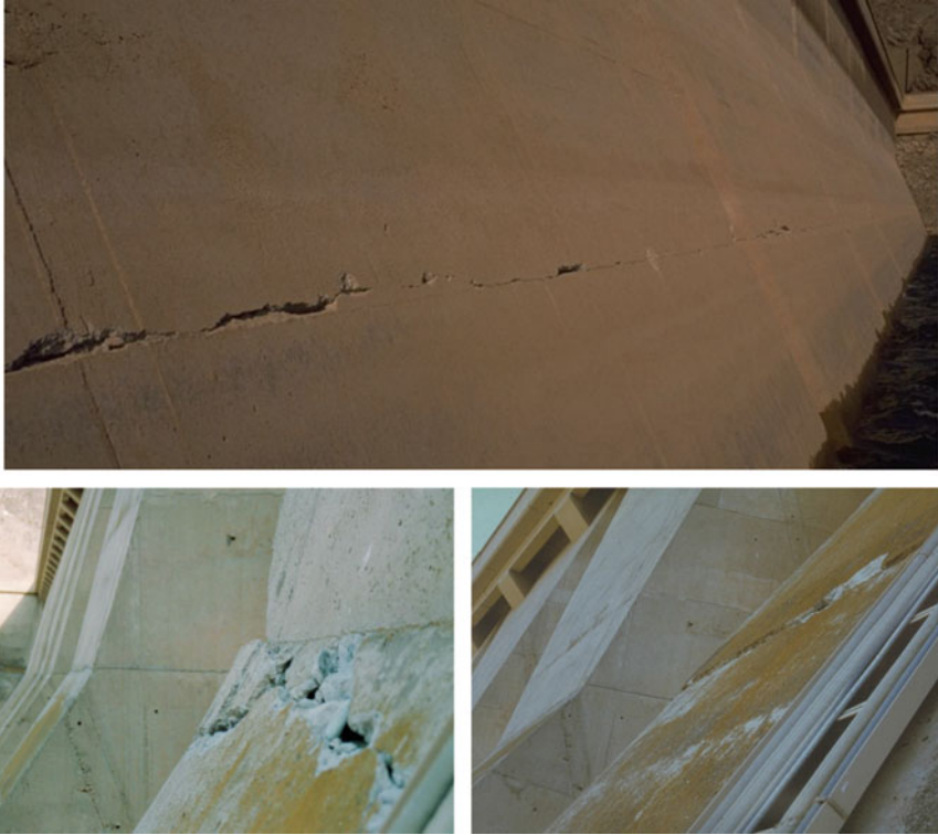
Fig. 20.1 Crack at upstream face ( top ) and at the kink ( left bottom ) and crack showing sliding movement of wedge formed by cracks at the kink ( right bottom ) of the buttress at the downstream face of the Sefid Rud buttress dam caused by ground shaking during the 1990 Manjil earthquake in Iran
