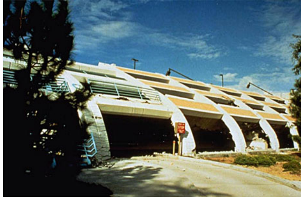
Fig. 1.13 Damage to precast concrete garage structure in the 1994 Northridge earthquake from the EERI photographic dataset for that earthquake (EERI 1995a)
