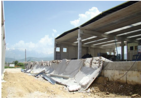
Fig. 4.8 Many cladding panels fell off the structures during recent Italian earthquakes (Toniolo and Colombo 2012)
